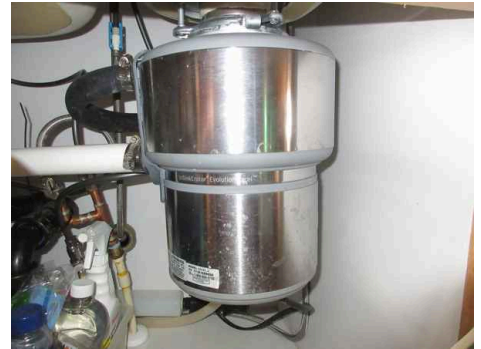
The waste disposal is functional
