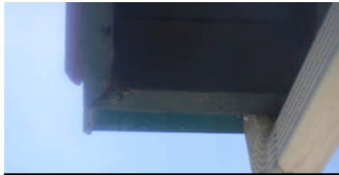
Exterior trim issues
