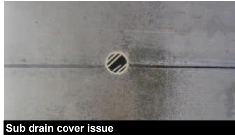
Sub drain cover issue
