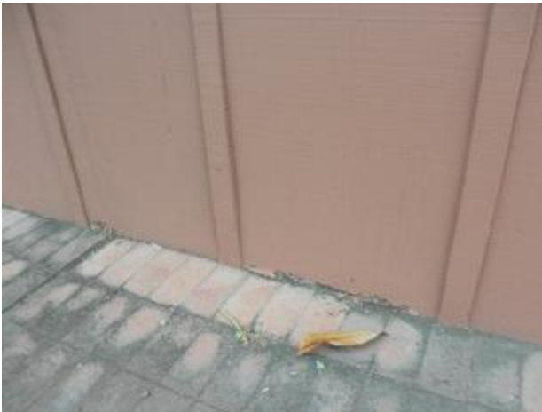
Moisture damage to the base of the wood siding.
