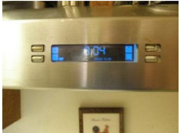
Buttons missing for exhaust fan in unit 3.
