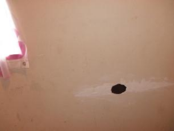
Hole in the interior wall at the community laundry.
