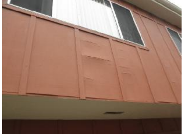
Example of some of the delamination at the exterior wood siding.
