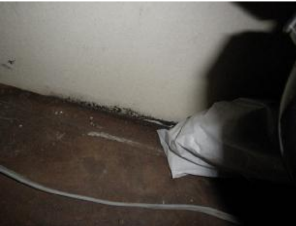
Black mildew like substance below the kitchen sink in unit 2.
