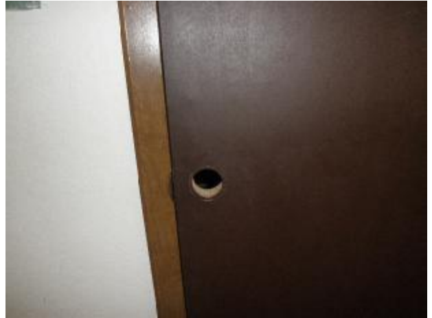
Door knob missing at living room closet in unit 2.
