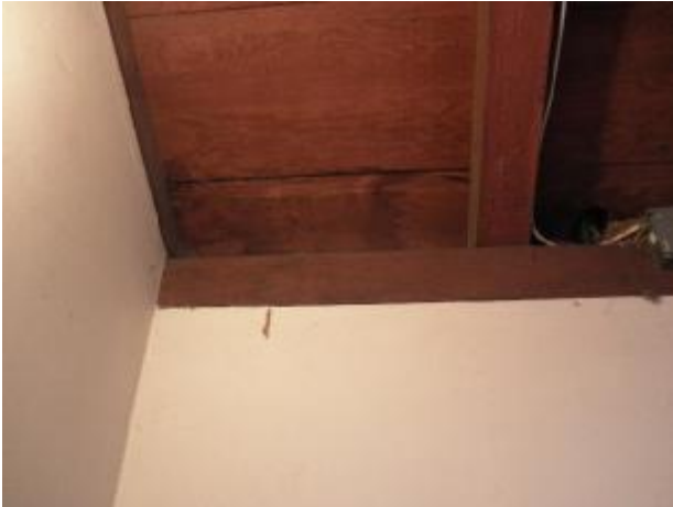
Evidence of a roof leak at the community laundry.
