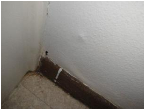
Example of moisture damage tot he drywall next to the shower.
