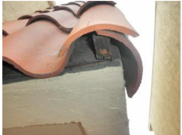
Moisture damage to the base of the 2X roof trim at the front of unit 3.
