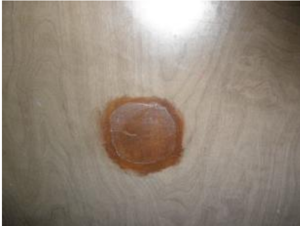
Patches and damage to bedroom door in unit 4.
