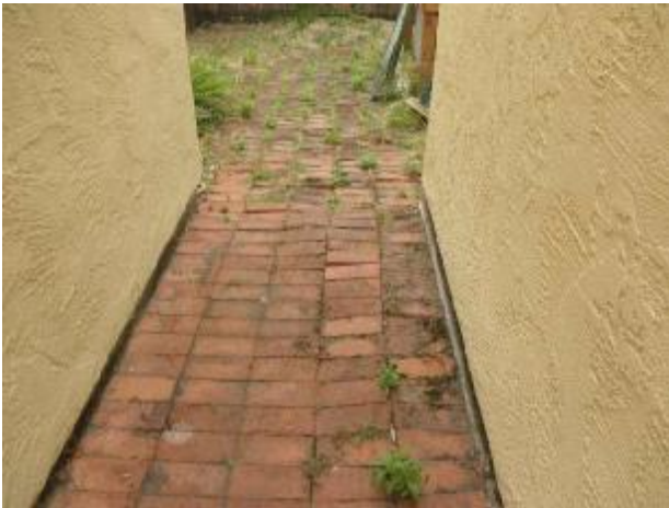
Uplifted and dislodged bricks in the breezeway.
