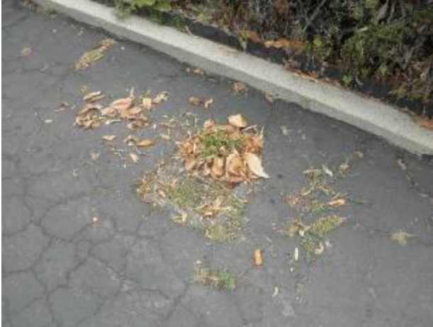
The surface site drain at the base of the driveway i clogged.
