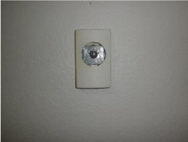
Example of missing control knobs for heating thermostats.
