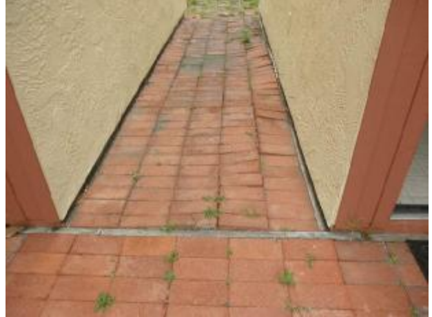
Uplifted and dislodged bricks in the breezeway.
