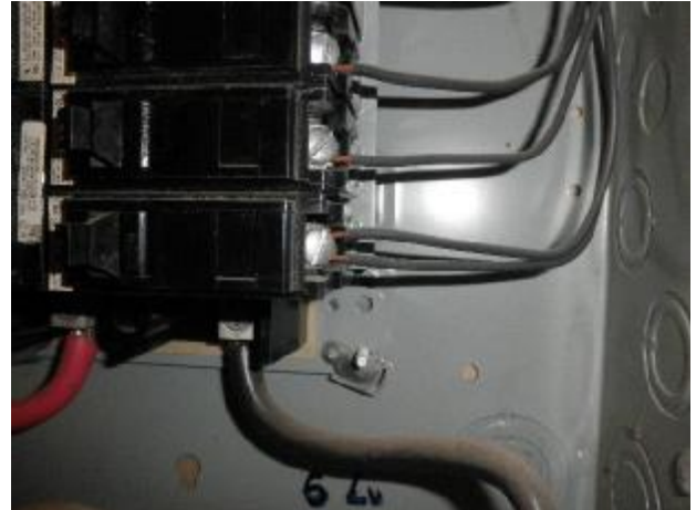
Example of double tapping in the subpanels.
