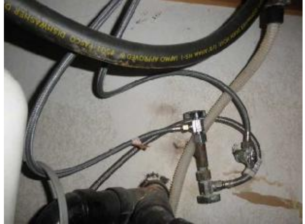
Black mildew like substance under the kitchen sink in unit 4.
