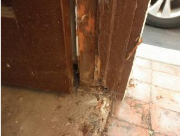
Termite infestation/damage to the base of the jamb at the exterior door in the community laundry.
