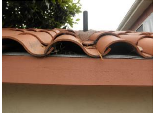
No double flashing at the vent pipe at the community laundry roof.
