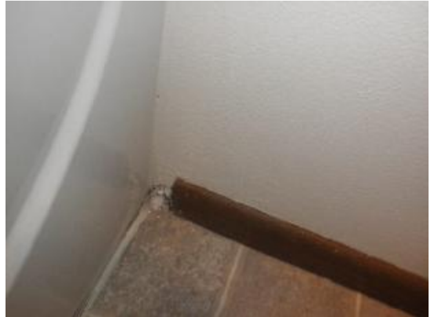
Example of moisture damage to the side of the shower.
