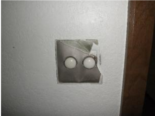
Example of cracked/damaged light switch cover plates.
