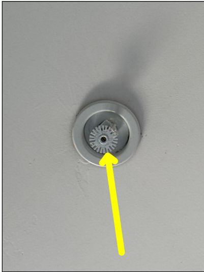
Garage fire sprinkler heads
