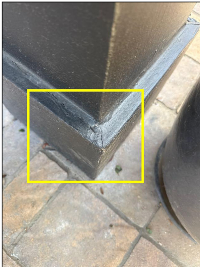
Minor moisture damage, wood rot, observed at the trim around the back patio posts.
