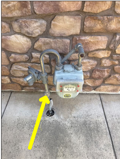
Main gas shut off to the home.
