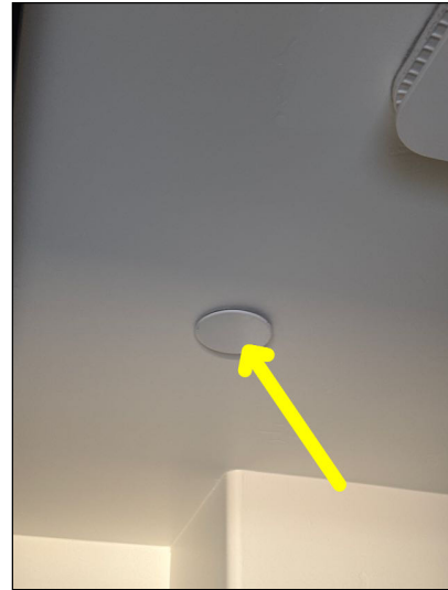
Fire sprinkler heads
