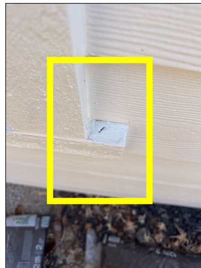
Moisture damage, wood rot, observed.
