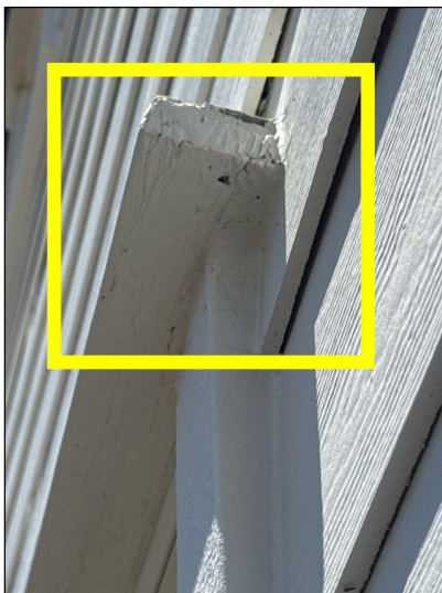
Moisture damage, wood rot, observed.
