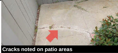
Cracks noted on patio areas
