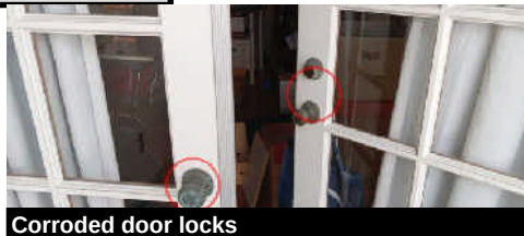
Corroded door locks
