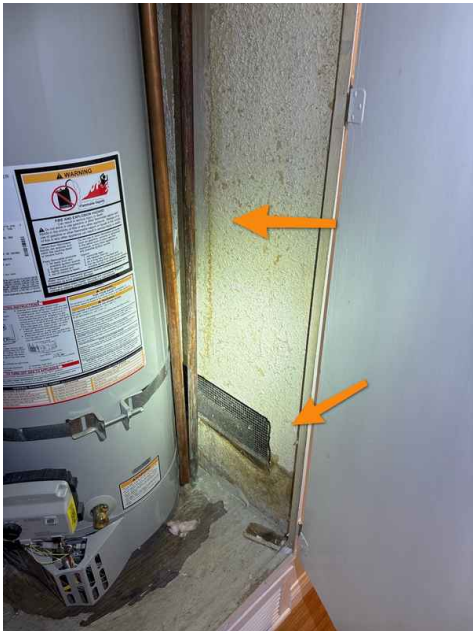
Water Heater closet
