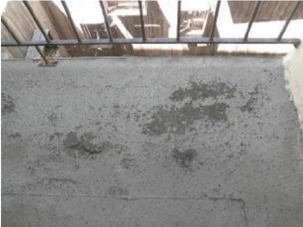
Example of wrong material for water proof decks and no flashings installed.
