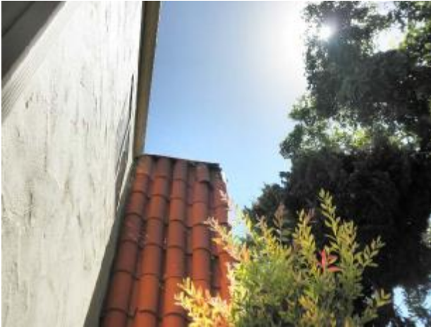
Damaged clay tiles at the SW corner of the roof.
