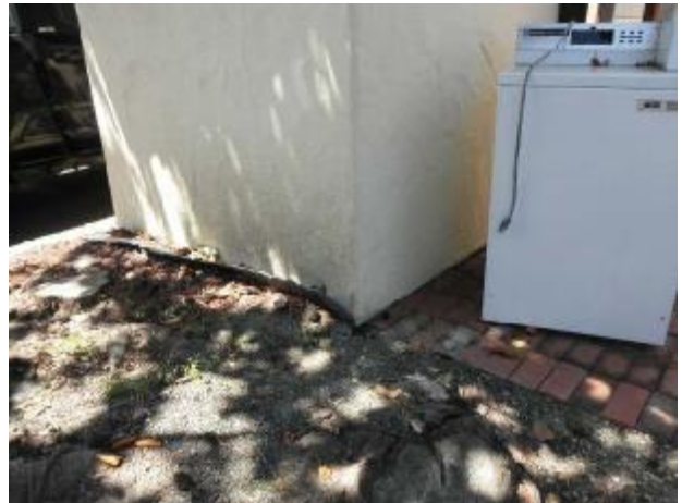
Faulty grade along the east wall of the community laundry building.
