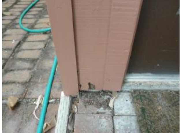
Example of some of the moisture damage at the exterior of the building.
