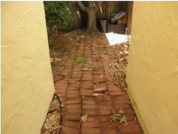
Uplifted and dislodged bricks at the walkway in the breezeway.
