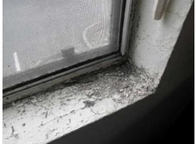
Moisture damage to the window sills in the bedrooms in unit 3.
