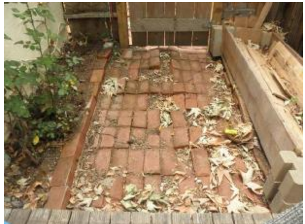
Uplifted and dislodged bricks at the walkway in the backyard at unit 3.
