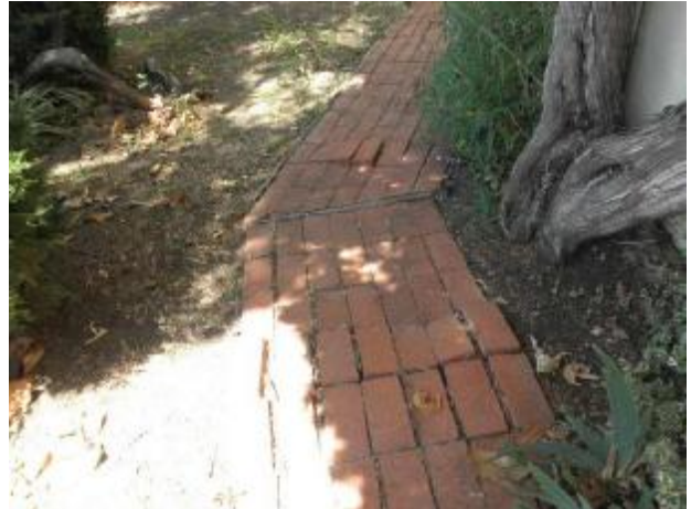
Uplifted and dislodged bricks at the walkway in the south lawn.
