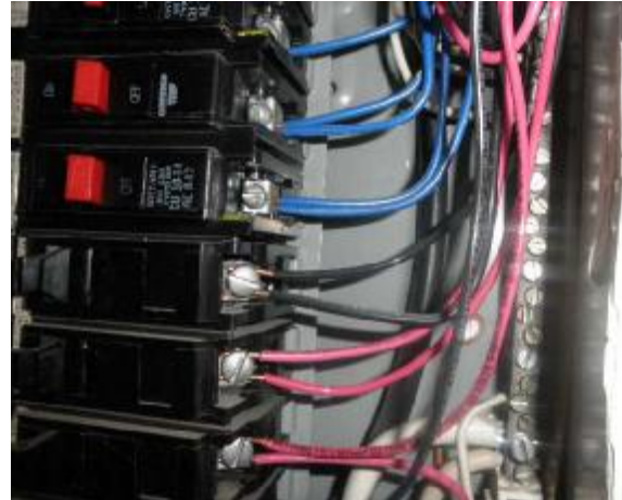
Example of double tapping in the electrical subpanels.
