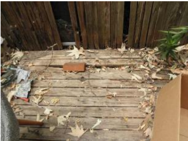
Example of the moisture damage at the wood decks.
