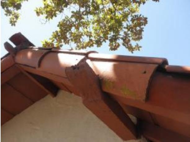
Moisture damage to the barge rafter at the community laundry room.
