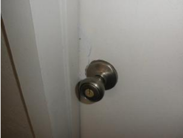
Damage to the center bedroom door in unit 4.
