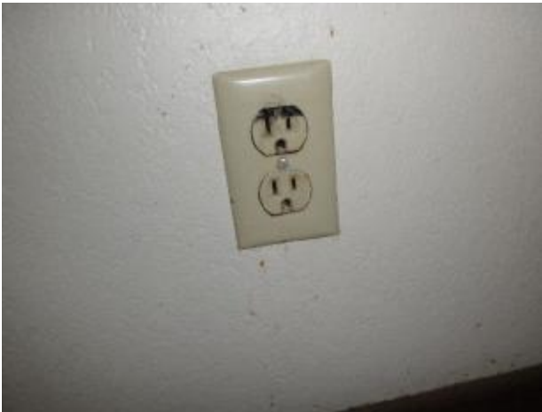
Scorched outlet in the bedroom in unit 3.
