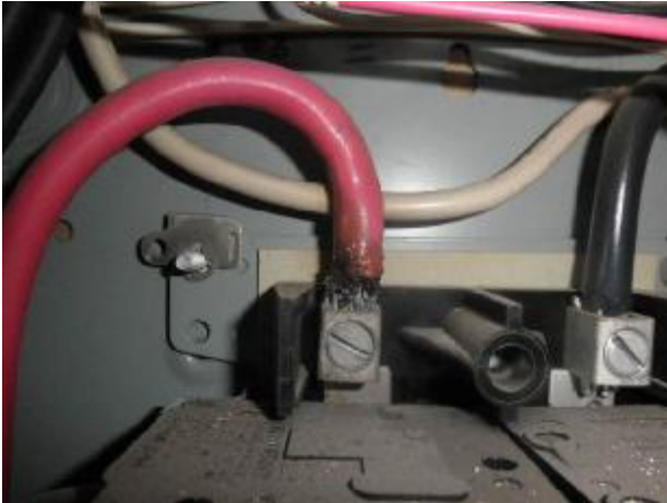
Scorched/melted wire at the at the electrical subpanel in unit 1.
