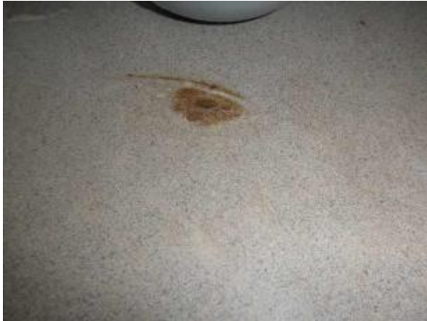
Burn mark in the kitchen counter in unit 4.
