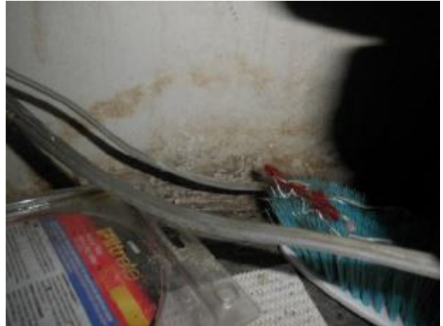
Black mildew like substance on the drywall below the kitchen sink in unit 3.
