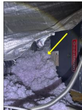
Combustible materials too close/touching unit - needs to be serviced
