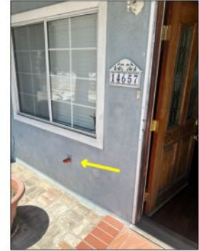
Three prong outlets not grounded - needs to be serviced
