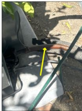
Missing insulation at compressor unit - needs to be serviced
