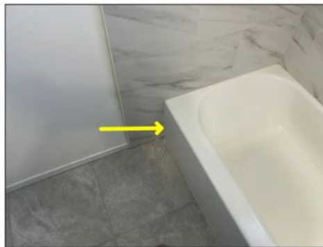
Caulking needed around perimeter
