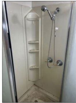
Wall materials in a worn/stained-faded/old condition - typical for age - recommend routine grout and sealer maintenance
