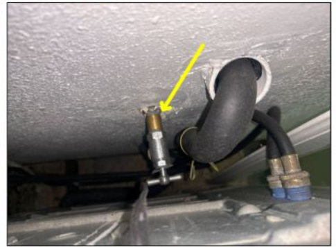
Fire caulk needed at plumbing/electrical penetrations
