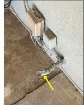
Bibb(s) not functional at one or more locations - needs to be serviced
