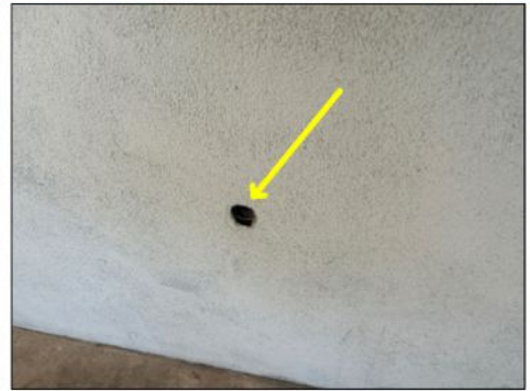
Holes more than typical - needs to be serviced
