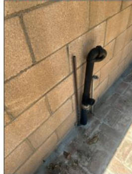
Plumbing pipes at exterior of structure are uncapped and not properly secured - needs to be serviced
