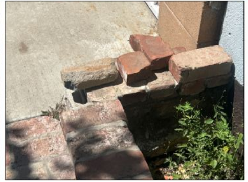
Damaged areas - needs to be serviced
