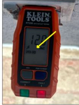
Three prong outlets not grounded - needs to be serviced
