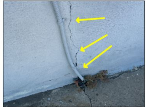
Cracking - more than normal - needs to be serviced - by main electrical panel
