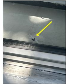
Cracked glass - needs to be serviced - south side
