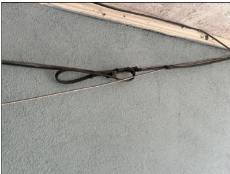
Interior rated wiring used outside - recommend servicing
