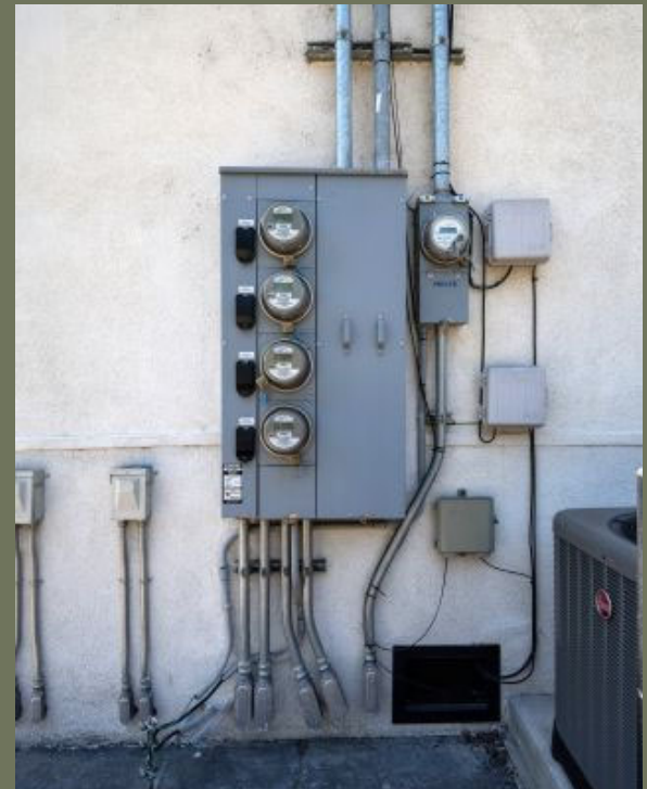
New main and sub panels
