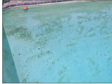
Flaking/peeling surface in areas - plaster is in a worn/older condition
