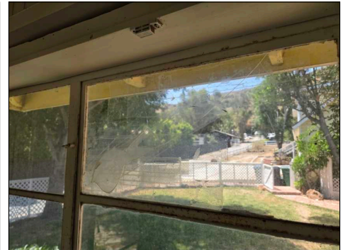
Cracked glass- needs to be serviced
