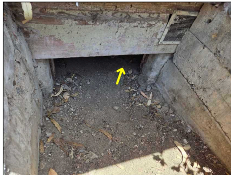
Inadequate clearance at entry - may be problematic
