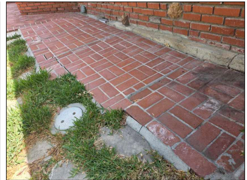
Cracking/chipping large - recommend servicing
