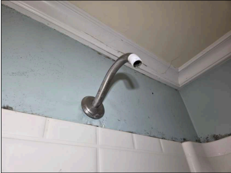
Missing shower fixture - needs to be serviced @ ADU
