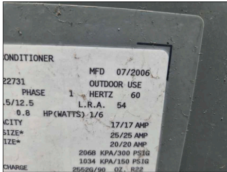
Unit old and appears to be nearing end of useful life - will likely need replacement soon @ ADU
