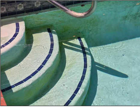
Stained more than normal in areas - needs to be serviced/cleaned
