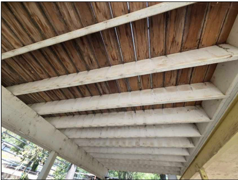
Deteriorated wood - consult termite report - needs to be serviced
