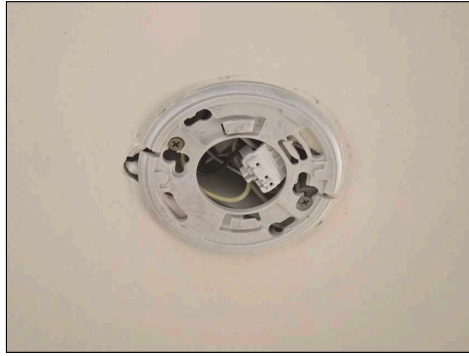
Missing - needs to be installed @ ADU
