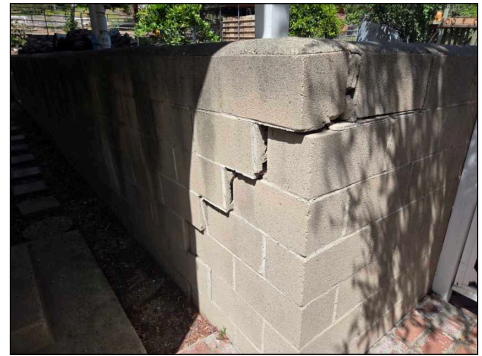
Leaning retaining wall - needs to be serviced
