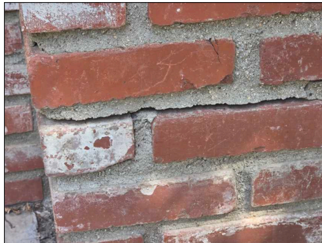
Cracking more than typical - needs to be serviced - signs of settlement at east side of the structure
