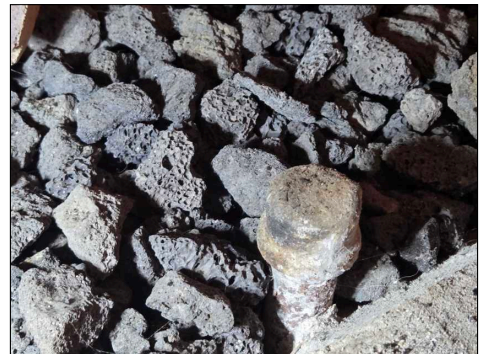
Gas line capped - no test
