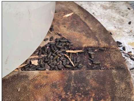
Evidence of rodents on or around the water heater base - recommend pest services inspection for further evaluation
