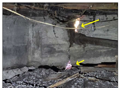
Damaged areas present - needs to be serviced
