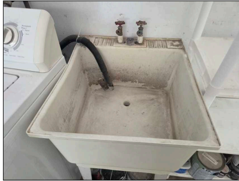
Not operating - needs to be serviced
