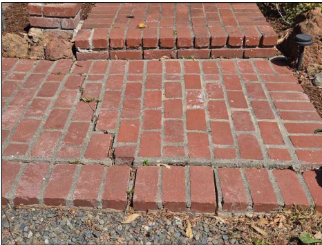
Walkway displacement/uplifted/uneven areas - potential trip hazard - needs to be serviced
