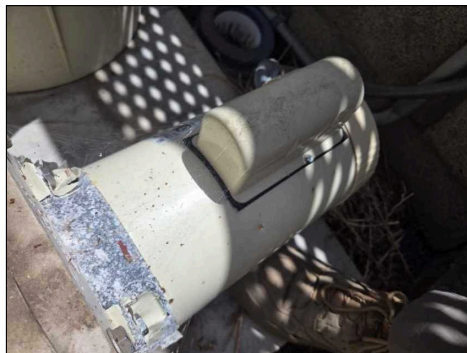
No bonding wire(s) visible at pumps/equipment – needs to be serviced
