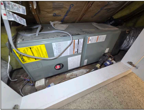
Operated at time of inspection
