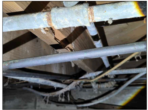
Galvanized water piping present - recommend upgrading all older pipes @ kitchen
