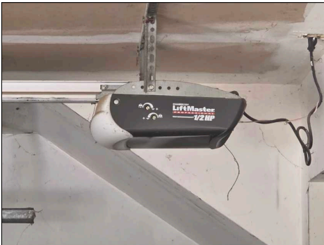
Did not operate - needs to be serviced - hardware not latching
