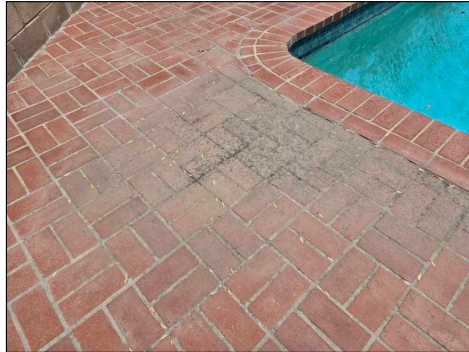
Evidence of poor drainage around pool areas - needs to be serviced
