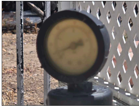
Fogging - needs to be serviced/replaced for optimum readability
