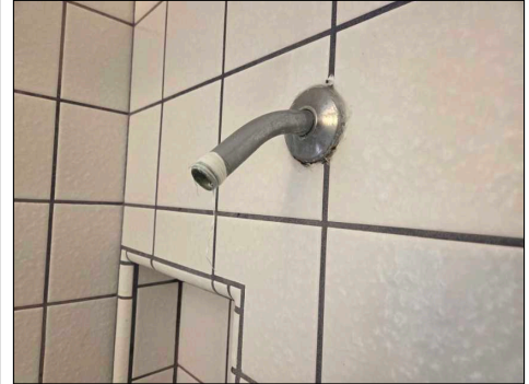
Missing shower fixture - needs to be serviced @ kitchen
