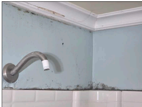
Microbial growth/irregular staining present - needs to be serviced @ ADU bathroom
