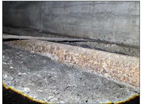
Older/corroded cast iron pipes present - materials nearing the end of their useful life
