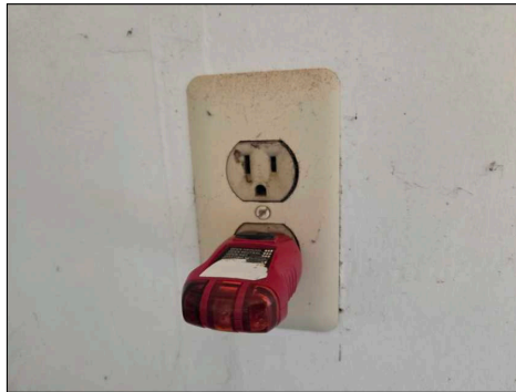
Non-energized (dead) outlet(s) - needs to be serviced
