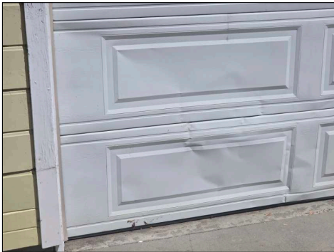
Dented/damaged areas - didn't affect performance - recommend servicing
