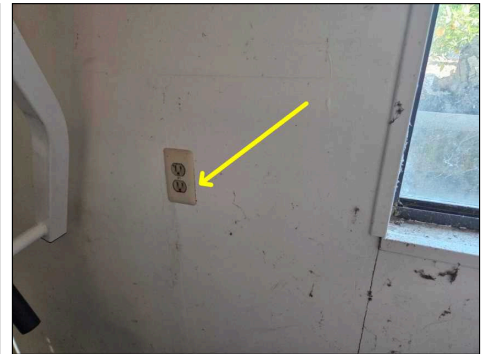
Non-energized (dead) outlet(s) - needs to be serviced
