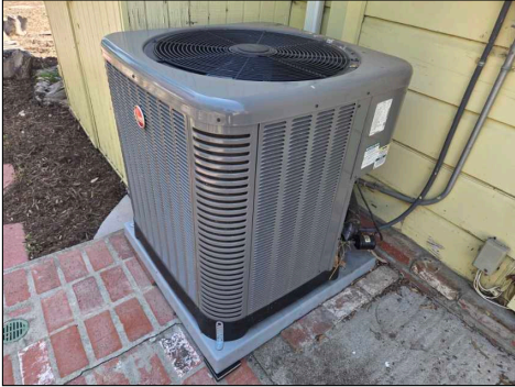
Operated at the time of inspection
