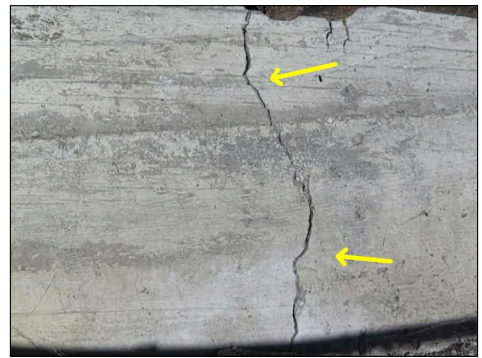
Cracked more than typical - needs to be serviced/further evaluated
