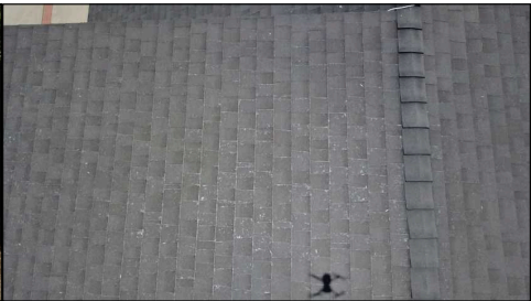
Shingles have moderate granule loss at ADU - older materials present
