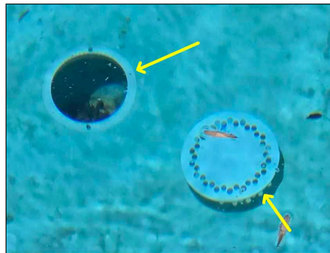
Main drain cover missing - needs to be serviced - drain clogged
