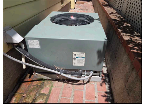
Operated at the time of inspection
