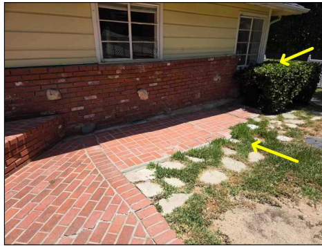
Evidence of settlement around the property at east side
