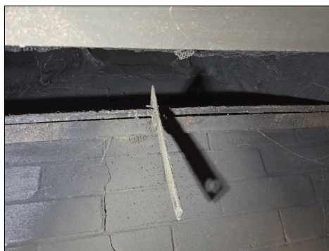
No damper stop clamp - required for cosmetic gas logs, fire-glass or other cosmetic fire system that uses gas at the primary fuel
