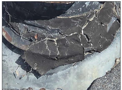
Deteriorated mastic at flashings - needs to be serviced and resealed at all penetration points
