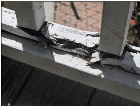
Deteriorated wood - consult termite report - needs to be serviced
