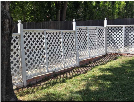
Loose/leaning areas of fencing/walls – needs to be serviced
