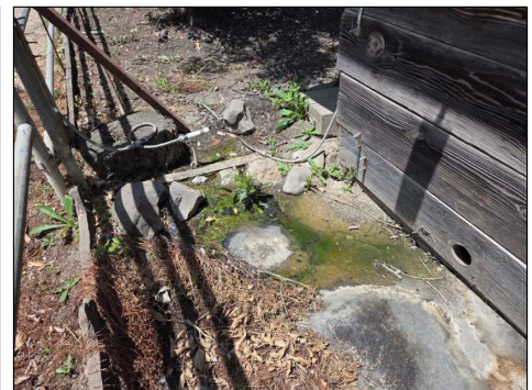
Evidence of water pipe leaking beneath the surface - water ponding in areas - needs to be serviced
