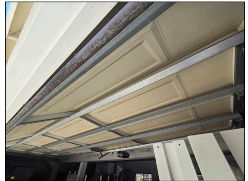
Dented/damaged areas - didn't affect performance - recommend servicing
