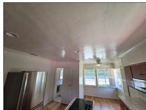
None present - recommend installing an exhaust vent system @ main
