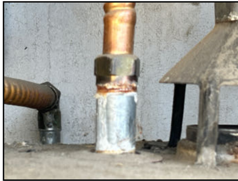
Corrosion present - signs of wear - monitor for moisture
