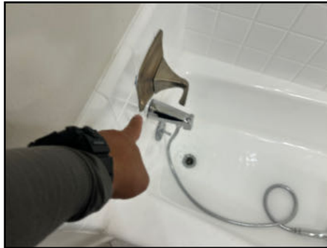
Caulk maintenance needed at wall to fixture juncture
