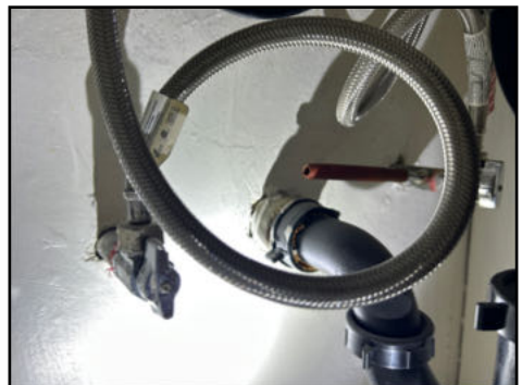
Galvanized water piping present - recommend complete water distribution system evaluation due to age
