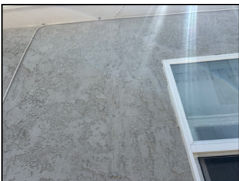
Cold joint cracking present - evidence of past patchwork or addition - check permits and seal joint regularly to ensure against moisture intrusion
