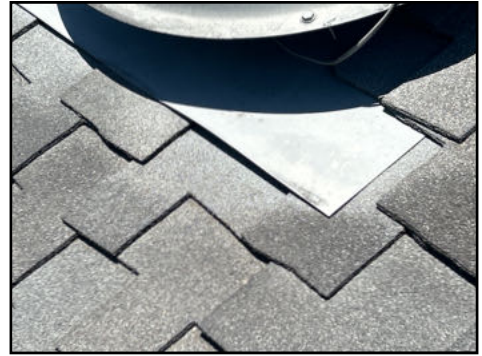
Flashings lifting in areas - needs to be serviced as part of your preventative roof maintenance
