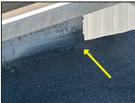
No kick-out flashing at roof to wall connection - needs to be serviced
