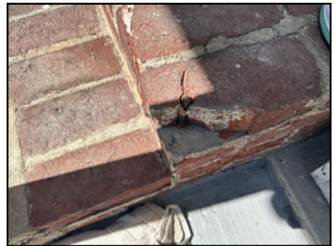
Damaged steps - unsafe - needs to be serviced
