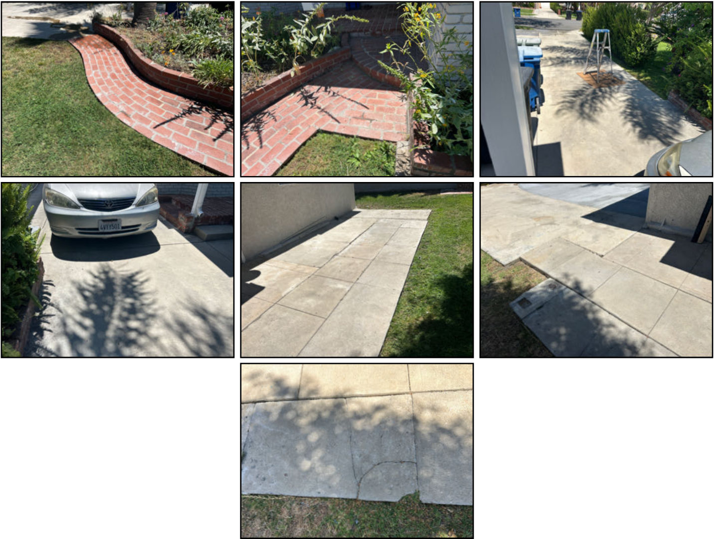
Cracking/chipping large - recommend servicing
