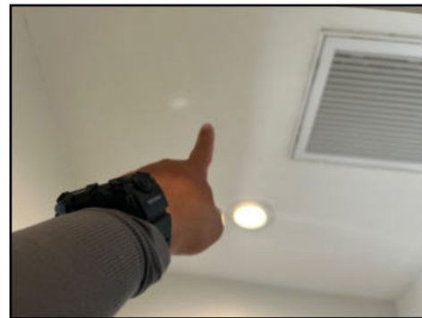
Missing at hall - needs to be installed
