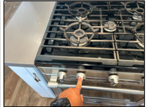
Left front element/burner not operating - needs to be serviced
