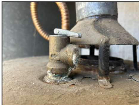
None - needs to be serviced/installed
