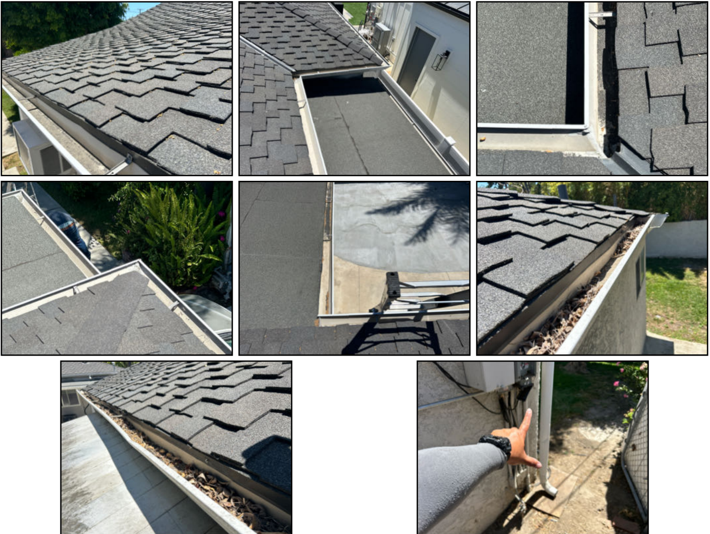
Separating from structure/loose in areas - needs to be serviced
