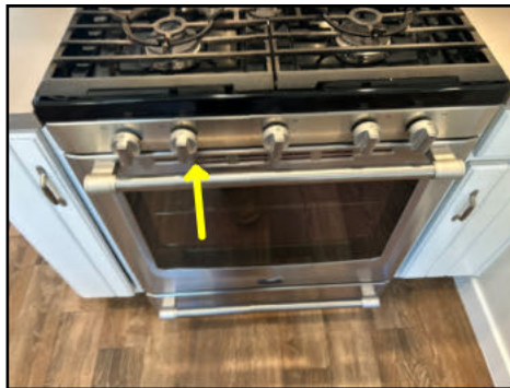
Electric ignitor does not appear to function - needs to be serviced
