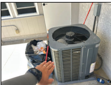
Unit is not level, this can affect system performance - needs to be serviced
