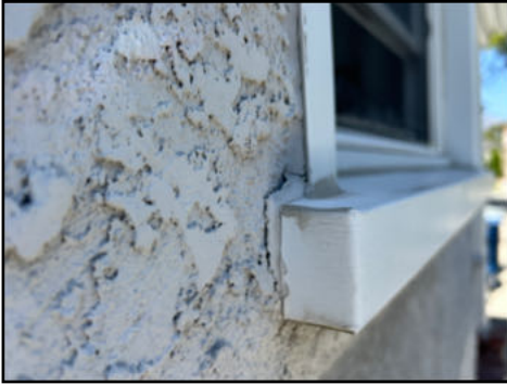
Gaps around windows - recommend servicing to prevent moisture entry
