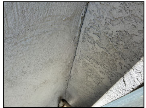
Cold joint cracking present - evidence of past patchwork or addition - check permits and seal joint regularly to ensure against moisture intrusion
