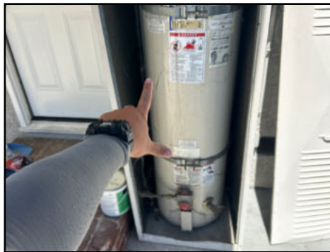
Loose strapping - needs to be serviced
