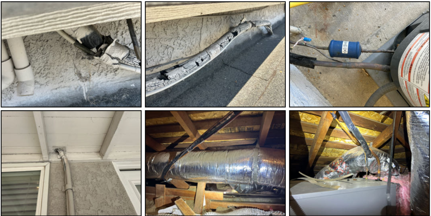
Insulation gaps observed in areas - needs to be serviced
