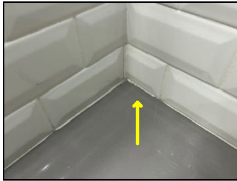
Gap at backsplash to countertop joint - needs to be serviced
