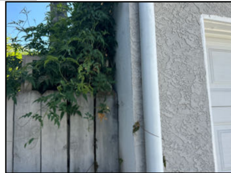
Zero Lot Line present - some areas around the structure are not accessible and not inspected
