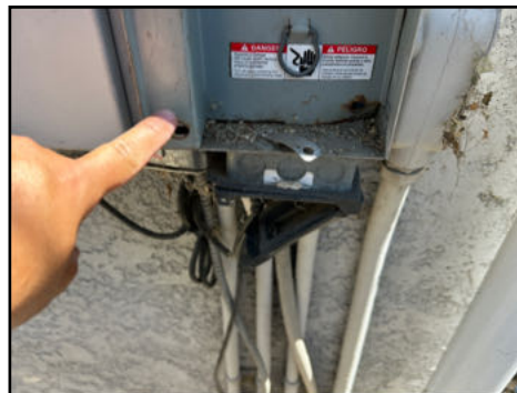
Panel cover screw(s) missing - recommend installing appropriate screws
