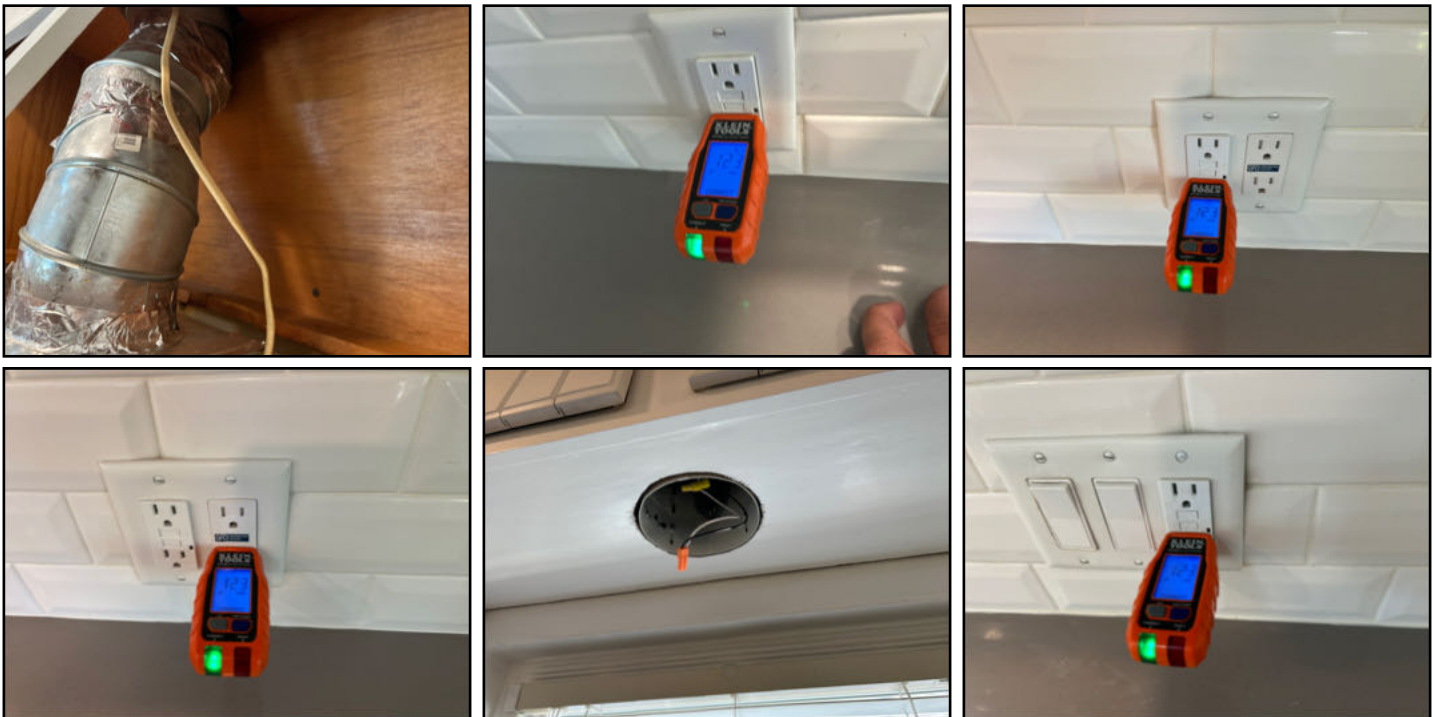
Exposed connections - potential hazard - needs to be serviced
