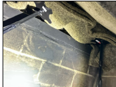
Flue sealed off did not test - needs further evaluation
