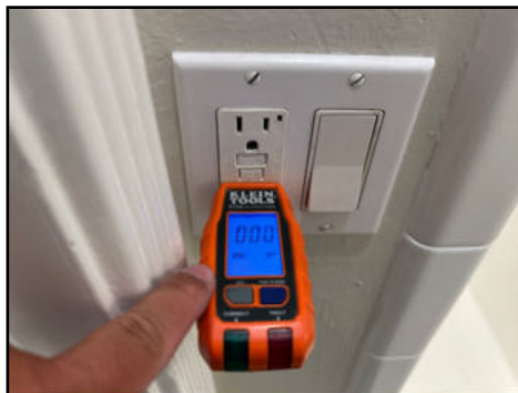
Non-energized (dead) outlet(s) - needs to be serviced
