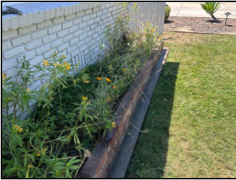
Trees or vegetation too close to structure areas - recommend servicing
