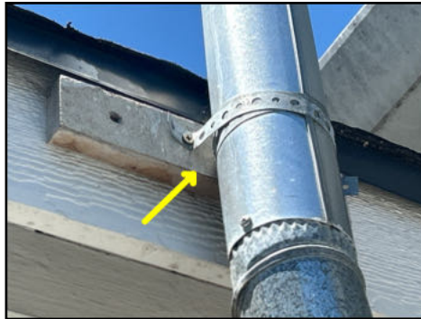
Minimum water heater single-wall vent pipe clearance from combustable material is 6" - needs to be serviced
