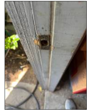
Recommend weather tight service/maintenance to prevent moisture intrusion
