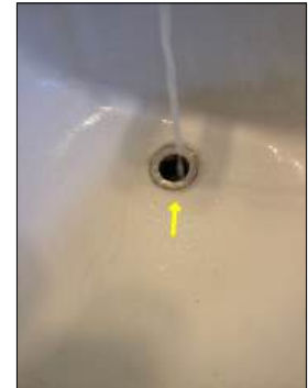
Drain stopper missing - needs to be serviced
