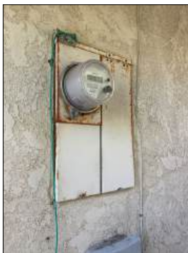
Heavy rusting or rust damage present - needs to be serviced
