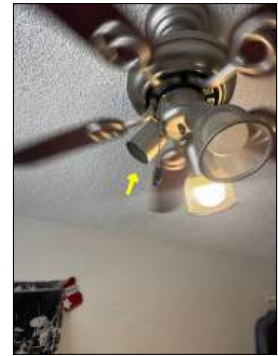
Missing light fixture globe(s) north bedroom
