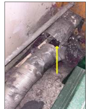
Dryer vent disconnected - needs to be serviced
