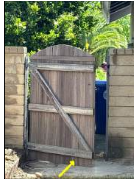
Gate is sagging - recommend servicing
