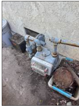
Seismic safety valve present - inspector cannot determine if valve is installed properly (seismic valves cannot be tested with this inspection)
