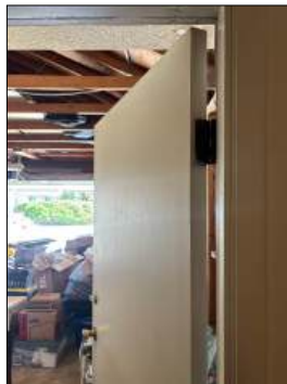
Door rating label painted over/missing - Inspector cannot determine fire rating
