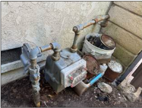
Minor rusting - typical for exterior weathering - recommend rust treatment
