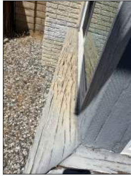
Weathered/worn more than normal - needs to be serviced
