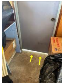
Visible daylight is present around the exterior door. Recommend proper weatherstrip seal and/or maintenance.
