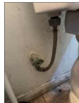
Water shutoff under toilet corroded - needs to be serviced - this will be an ongoing maintenance issue for ALL plumbing valves hall bath
