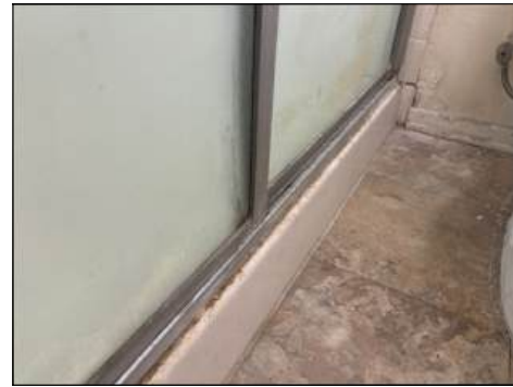
Corrosion present in areas - signs of wear and moisture accumulation
