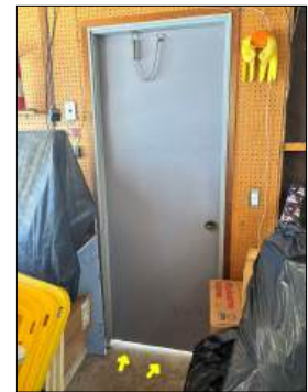
Missing threshold - needs to be serviced
