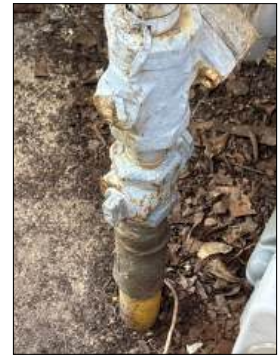
Recommend gas valve wrench be placed near valve for optimal preparedness
