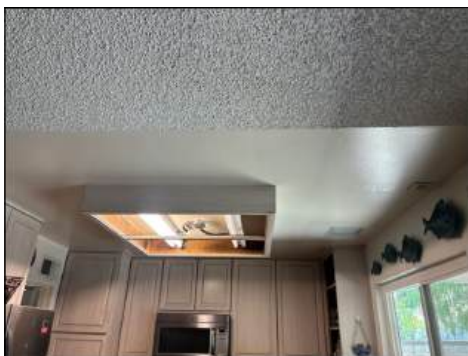
Some bulbs defective/missing/light(s) did not function - check bulbs/consult electrician to further evaluate
