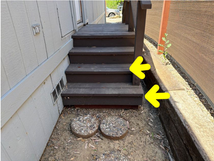
One or more steps have unequal treads or risers. Steps are required to be uniform to prevent trip-hazards. The rise of any step should be no less than four inches and no greater than seven and three-quarter inches, and the run should be no less than eleven inches. Also, the dimensions of the largest step should not exceed that of the smallest by more than three-eighths of an inch.
