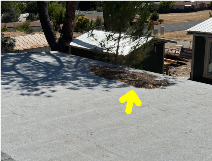
The roof needs to be cleaned and any foliage trimmed away to promote and insure proper drainage.
