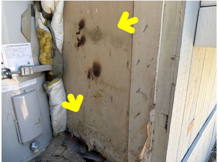
There is a dark staining within the water heater closet that should be evaluated by a qualified specialist and cleaned as necessary.
