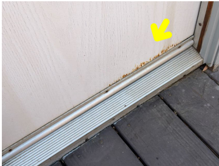
The finish on one or more of the exterior doors is weathered, and you may wish to have them refinished or replaced.
