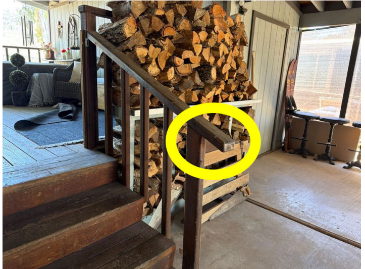
The handrail does not return, which is required at the top and bottom of the stairs by current building standards. This condition could allow a purse or clothing to initiate a fall.
