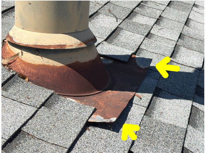
The toe of one or more of the flashings has been lifted, probably by the wind, and should be serviced.
