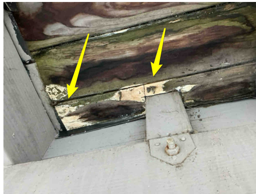
Fungus/ moisture damage
