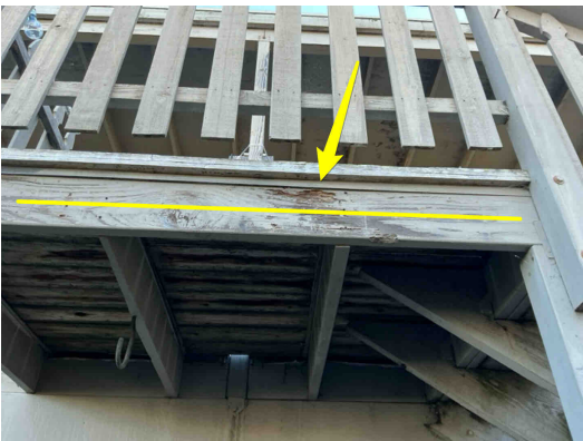
Moisture damage and improper use of a rim joist as a beam
