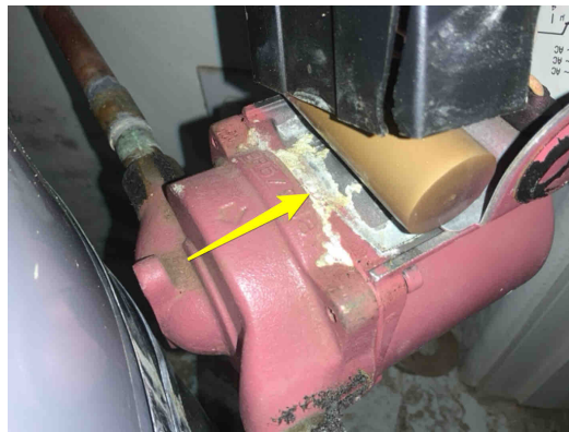
Evidence of past leakage
