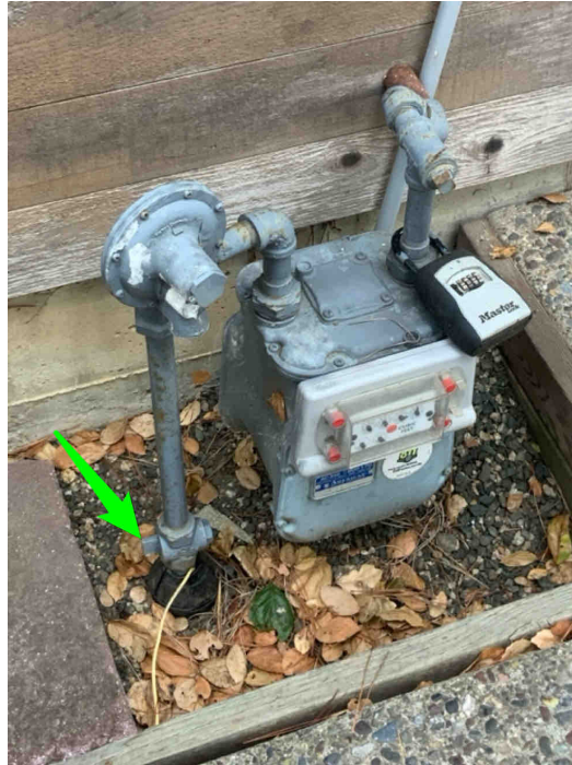
Main gas shut off valve
