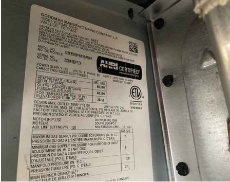
HVAC Equipment: Heater Energy Source Gas
