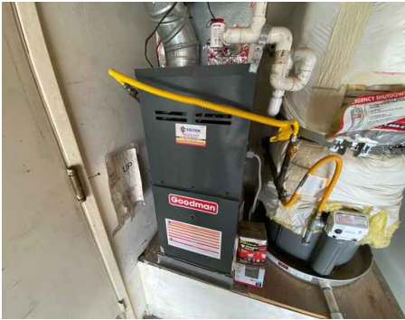
HVAC Equipment: Heater Brand Goodman
