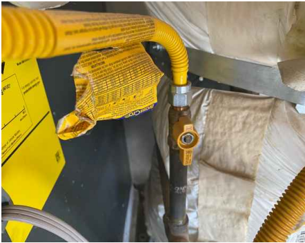
HVAC Equipment: A/C Brand Goodman
