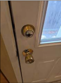
Emergency Egress Concern. Exterior door(s) have a double-sided keyed dead bolt lock set. This type of lock requires a key to unlock the door from the inside and can present an obstacle to anyone trying to evacuate the home in the event of a fire.
