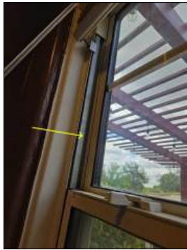
Broken sash cables or springs- unsafe - needs to be serviced - at half bath
