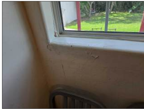
Stains/blistered areas present - tested dry with moisture meter at time of inspection - at bedroom southwest
