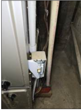
Switch cover damaged - needs to be serviced - at heater
