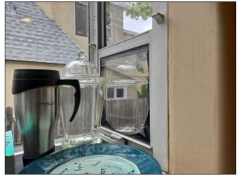
Inner seals at double pane windows are bulging/moving due to heat - needs to be serviced - at northwest, kitchen
