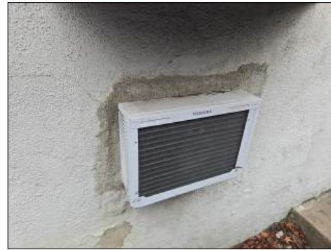
Irregular installation - may be problematic - further evaluation recommended
