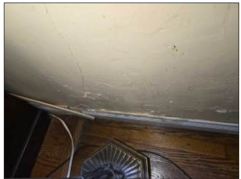
Stains/blistered at base - tested dry with moisture meter at time of inspection - monitor area for moisture/potential moisture intrusion - at master bedroom, family room
