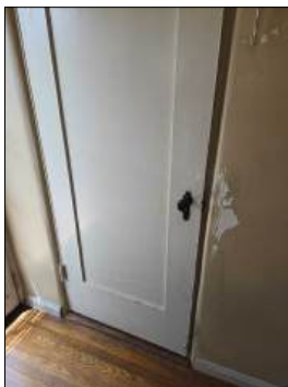
Did not latch properly - needs to be serviced - at bedroom southwest, half bath
