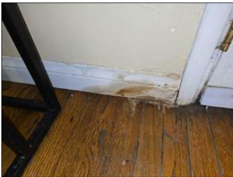
Stains/blistered at base - tested dry with moisture meter at time of inspection - monitor area for moisture/potential moisture intrusion - at master bedroom, family room
