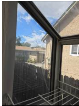
Cracked glass - needs to be serviced - at bedroom northwest
