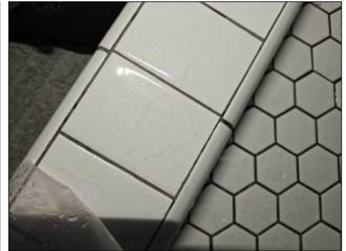
Broken/cracked tile(s) - needs to be serviced - at master, hall
