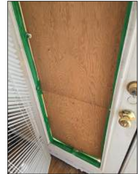
Broken/missing glass - needs to be serviced - at family room
