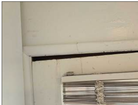
Gap(s) present/not square - needs to be serviced - at laundry area
