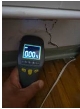
Stains/blistered at base - tested dry with moisture meter at time of inspection - monitor area for moisture/potential moisture intrusion - at master bedroom
