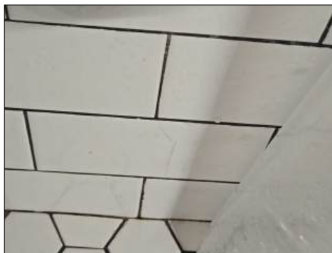
Broken/cracked tile(s) - needs to be serviced - at master, hall
