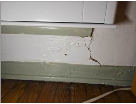
Stains/blistered at base - tested dry with moisture meter at time of inspection - monitor area for moisture/potential moisture intrusion - at master bedroom, family room
