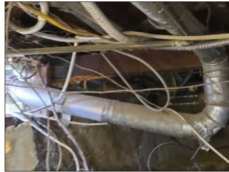
Loose connections under structure - irregular installation - heavy lint under structure - needs to be serviced
