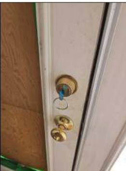
Emergency Egress Concern. Exterior door(s) have a double-sided keyed dead bolt lock set. This type of lock requires a key to unlock the door from the inside and can present an obstacle to anyone trying to evacuate the home in the event of a fire.
