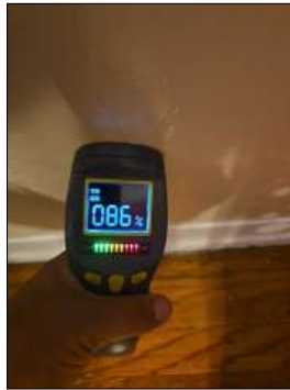
Stains/blistered areas present - moisture present when tested with moisture meter - recommend further evaluation - at middle bedroom, half bath, family room
