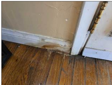
Evidence of possible moisture intrusion - dry at time of inspection - monitor for moisture - at family room
