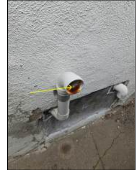
Missing/damaged screens at exterior - recommend service to prevent pest entry
