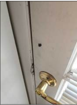
Screwed shut - needs to be serviced - at laundry area
