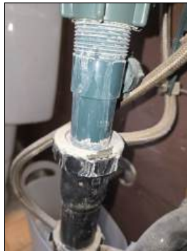
Visible leaking under sink - recommend licensed plumbing contractor for further evaluation and repair - at half bath
