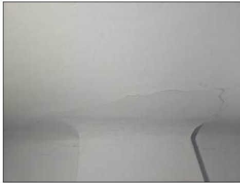
Large cracks present - needs to be further evaluated/serviced - at living room by fireplace
