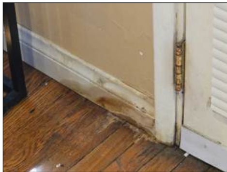
Moisture damage at base - needs to be serviced - additional hidden defects may exist - at family room
