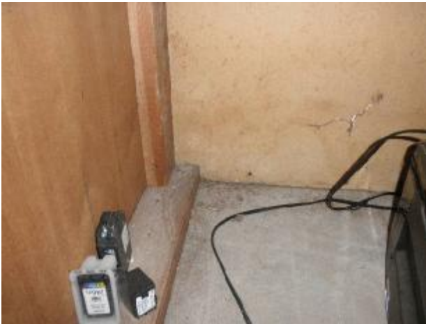
Subterranean termites in the cabinet below the stairs.
