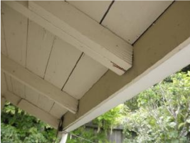
Termite infestation/damage at the eave and rafter tails.
