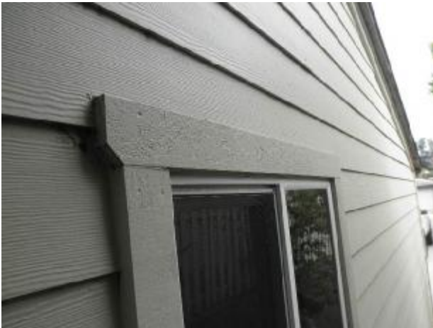
Missing Z bar flashing above the header trim where the cement board siding is installed.
