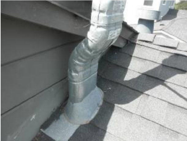
Missing storm collar at the wall heater exhaust vent flashing.
