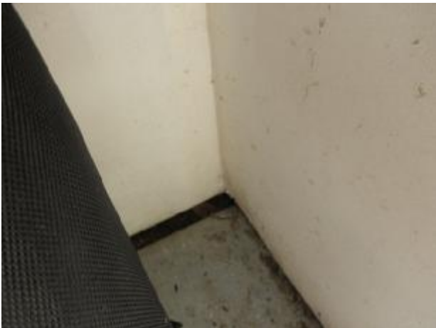
Faulty grade at the front NW corner of the garage with evidence of water intrusion.
