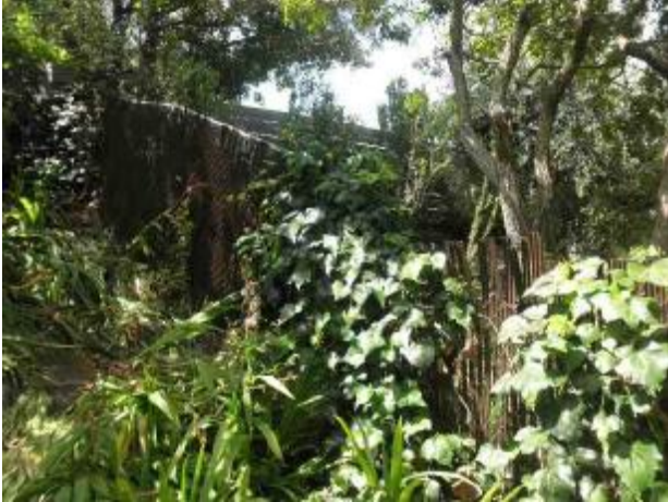
Parts of the fencing in the backyard is damaged.
