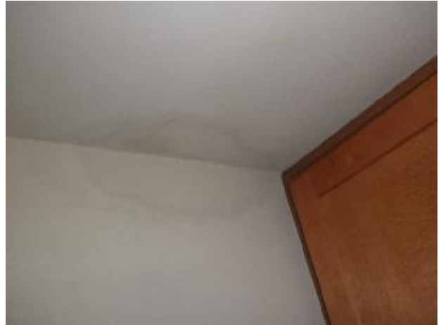
Water stain at the family room alcove.
