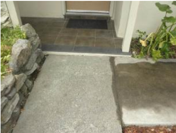
Tripping hazard at the interface of the front concrete walkway and the front patio.
