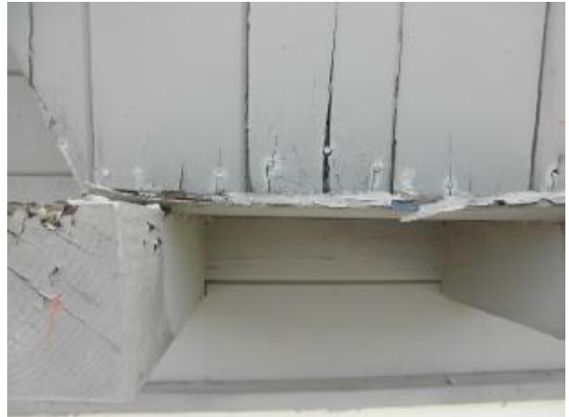
Moisture damage to the wood siding and beam at the second story Copula.
