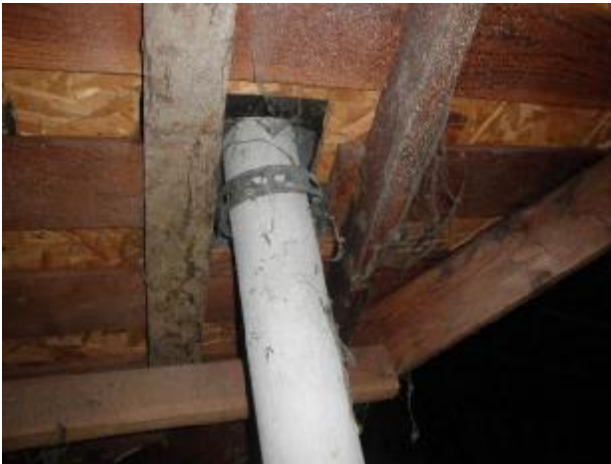
Transit pipe for the water heater exhaust.
