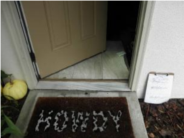
Low threshold condition at the entry door to the front bedroom.
