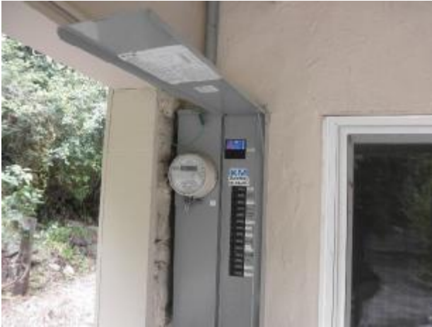
The main electrical service panel has been upgraded.
