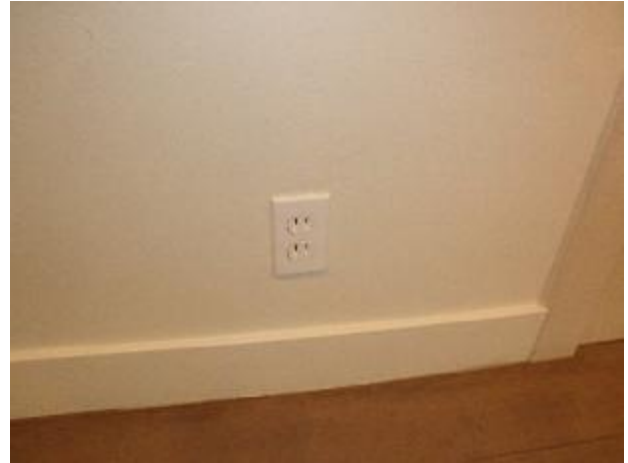
Two prong outlets in the living room.
