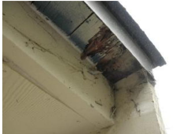
Old termite damage to the eave at the NE corner of the garage.
