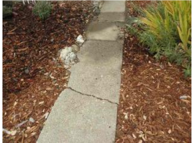
General settlement cracks in the front yard concrete walkways.
