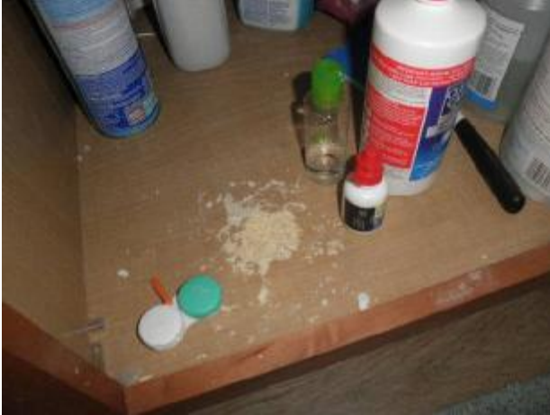
Moisture damage at the sink cabinet in the hall bathroom.
