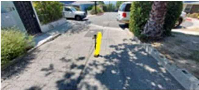
Section of fiberglass liner. Depth about 2 ½'.
