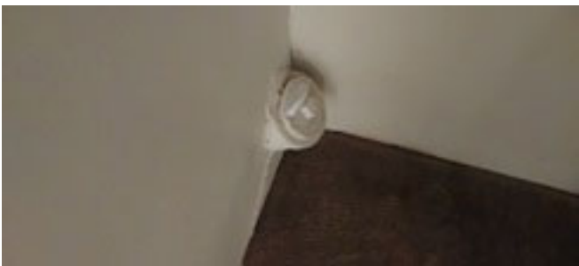
Second inspection attempted here.
