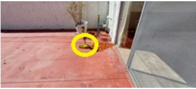
Location of main cleanout. Transition from cast iron to plastic pipe. Depth about 2'.
