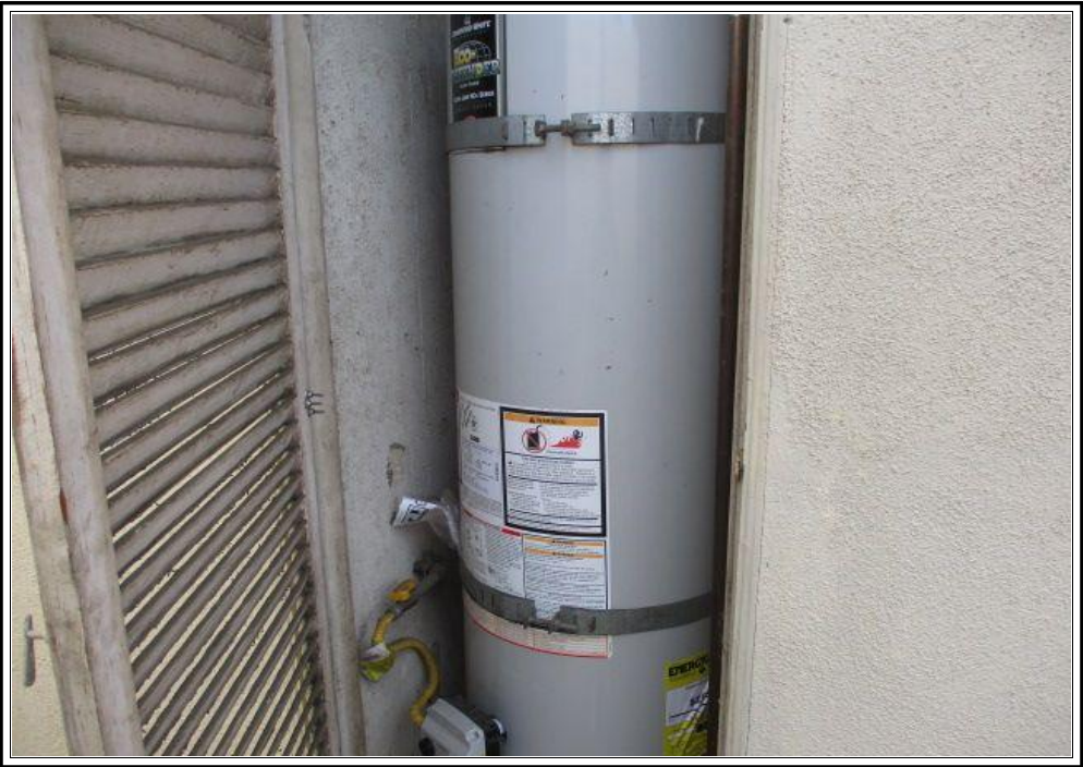
HOT WATER HEATER #1
