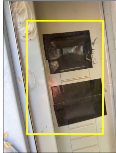
Unfilled openings in the electrical service panel were covered with tape.
