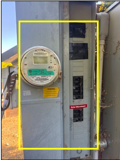
Main electrical service panel to the home.
