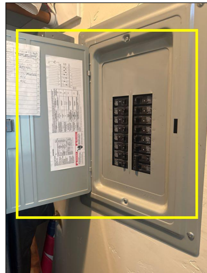
Sub panel to the home in the closet
