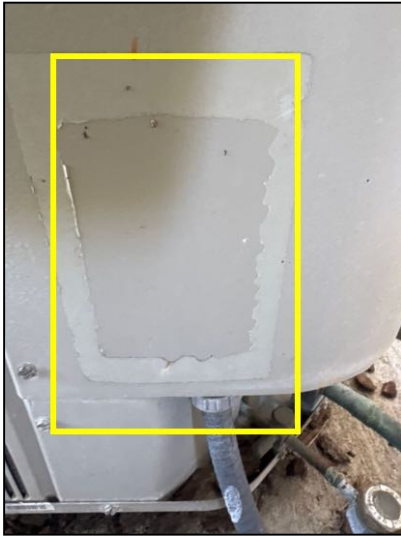
The data plate containing information about this A/C unit was illegible.
