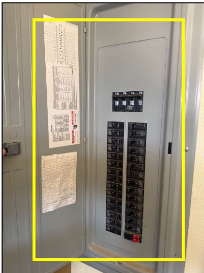
Sub panel to the home in the garage
