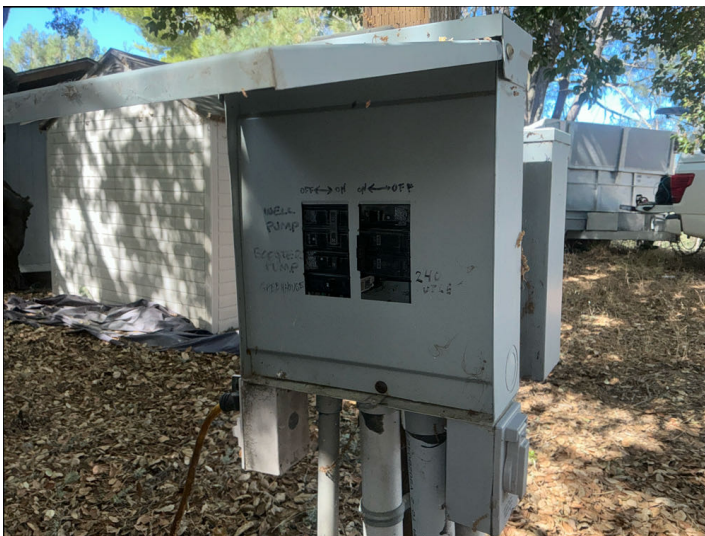
The sub panel is located adjacent to the well equipment.
