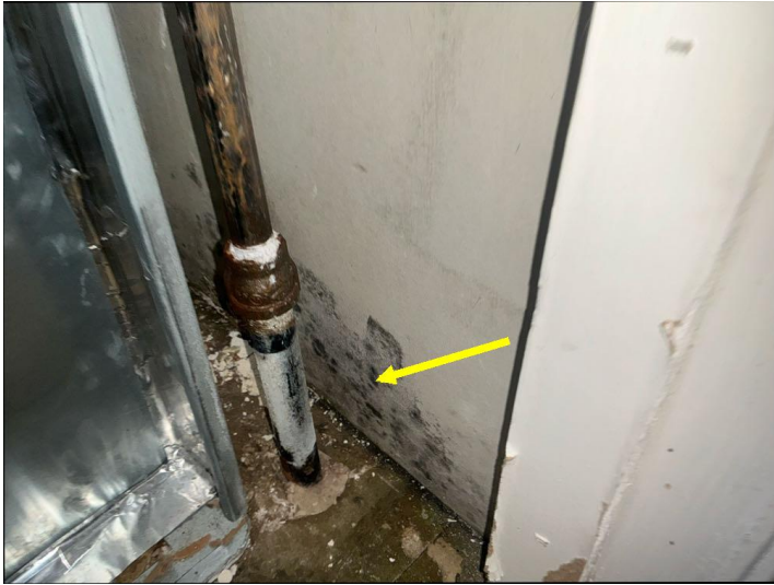
There is a bio-organic substance adjacent the water heater that should be evaluated by a specialist. All molds flourish in a damp environment and many are commonplace, but some are toxic and pose a health risk.
