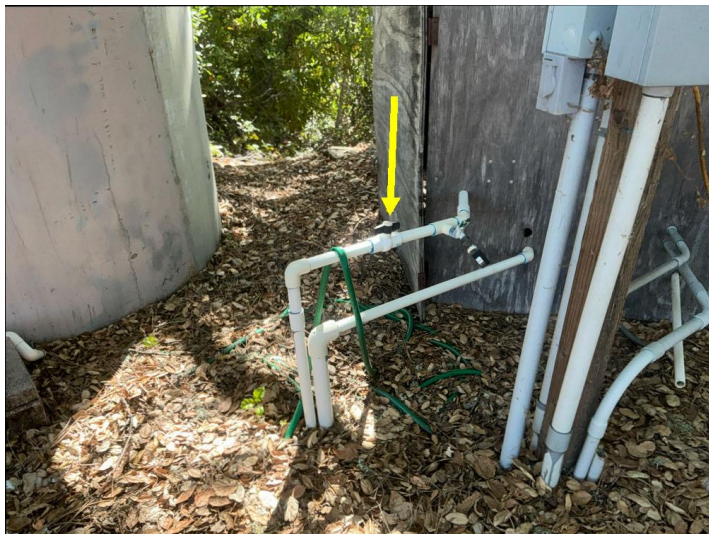
Main water shutoff
