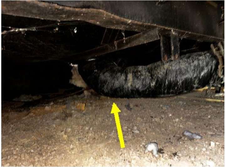
The flexible ducts in the crawlspace are in contact with the soil and should be a minimum of 4" off the ground. The plastic covering will deteriorate when in contact with the soil.
