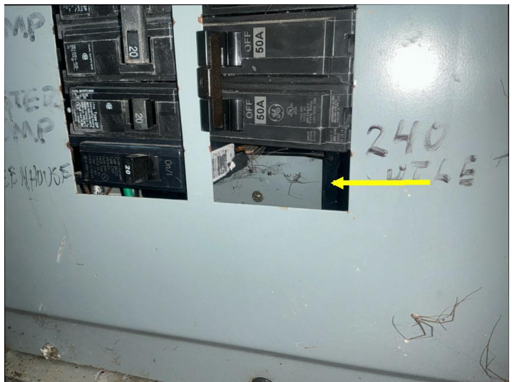
The interior panel cover has voids, or open knock-outs that should be covered, could prove to be hazardous to small children.
