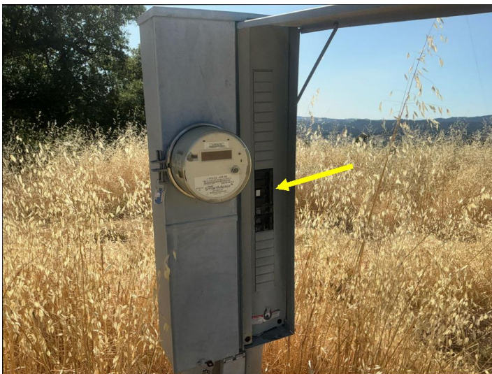
Main electrical service disconnect(Shutoff)
