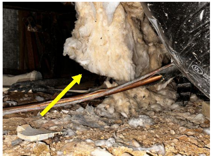
Some pieces of insulation are hanging or have fallen from between the floor joists. This does not have any serious consequences, but you may wish to have it serviced.
