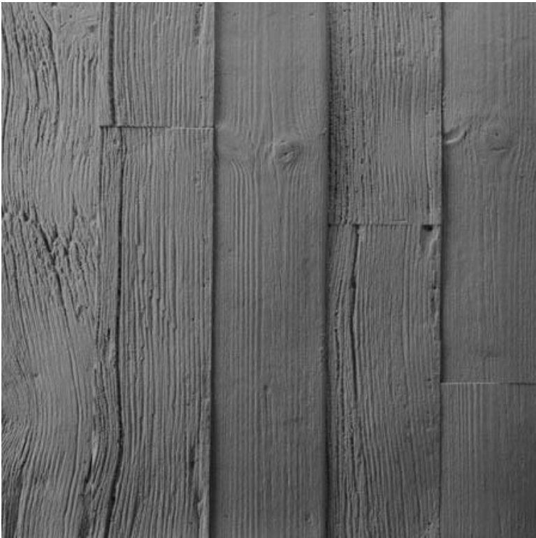
CAST IN PLACE RETAINING WALL - COLOR: NATURAL FINISH: WEATHER WOODGRAIN SEE T-4.0 FOR ADDITIONAL INFORMATION
