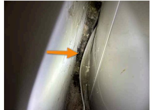
Water Heater Area
