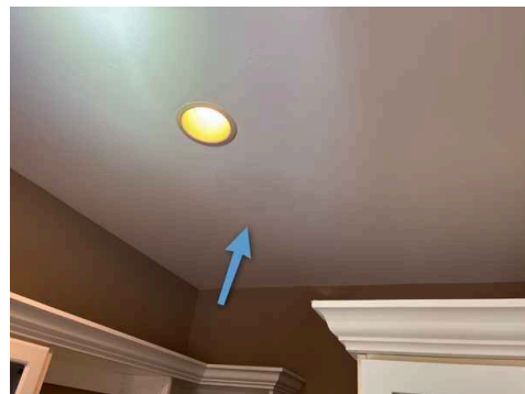
Master Bathroom Closet
