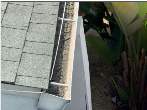
Clogged/restricted by debris in areas - recommend servicing
