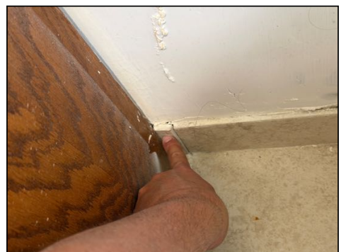
Loose baseboards in areas - needs to be serviced
