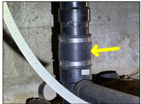
Rubber drain connections present - these are not for long term use - recommend upgrading connections
