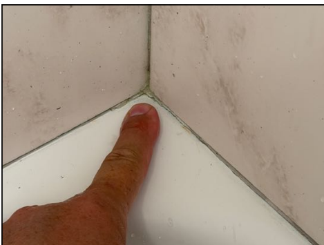
Cracked/loose/missing grout in areas - recommend grout and sealer
