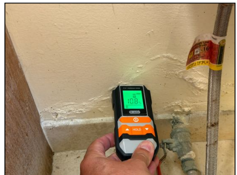
Stains at base - tested dry with moisture meter at time of inspection - monitor area for moisture
