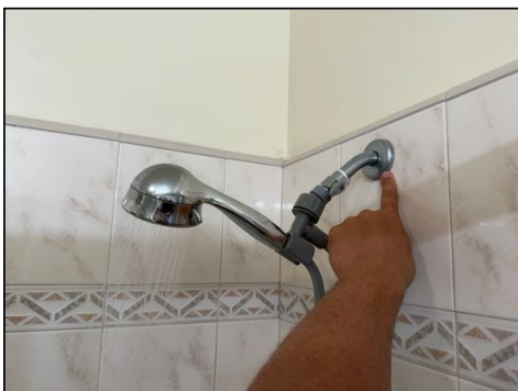
Shower arm faceplate is loose at the wall - recommend securing and sealing this area - both
