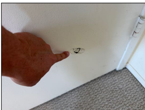
Hole in bedroom door - service recommended
