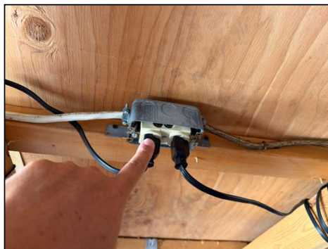
Outlet covers missing inside shed – service needed
