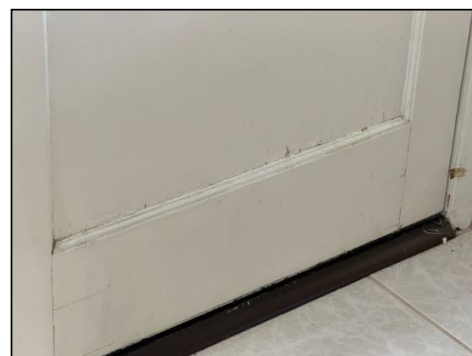
Weathered/worn door(s) - typical for age
