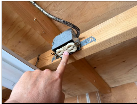
Outlet covers missing inside shed – service needed
