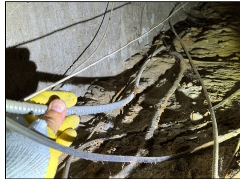
Conduit or metal wire sheathing in contact with soil - needs to be serviced
