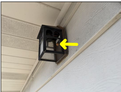
Fixture globes/covers damaged or missing – service needed
