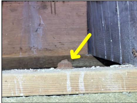
Anchor bolts present - worn with rust present - typical for age
