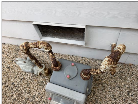
Significant rusting - needs to be serviced
