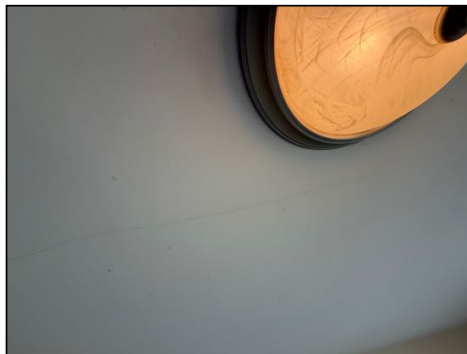
Small cracks/holes/chipped/dirty areas/cosmetic blemishes observed - typical for age of structure
