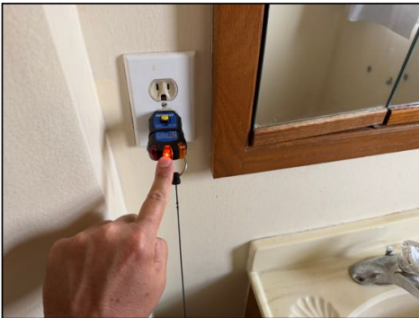
Three prong outlet(s) not grounded - needs to be serviced - both
