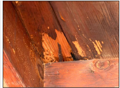
Wood deterioration observed - consult termite report for any wood areas in garage area
