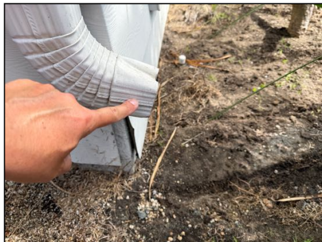
Extensions/splashblocks needed at downspout terminations to direct water away from foundation
