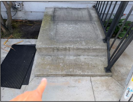
Rise too short - unsafe - needs to be serviced
