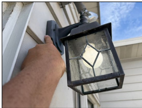
Electrical fixtures need to be caulked/sealed to wall attachments to help prevent moisture entry
