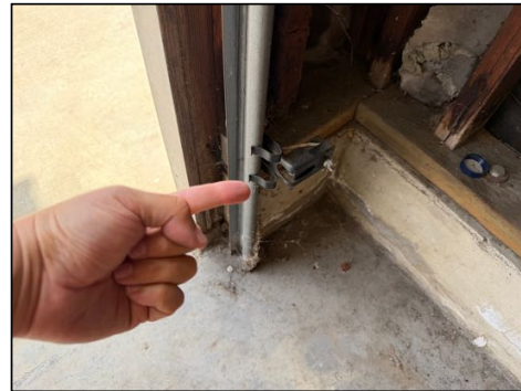
Light beam sensors are installed too high - needs to be serviced (recommended height is between 6 and 8 inches off the ground - manufacturer specifications may differ)
