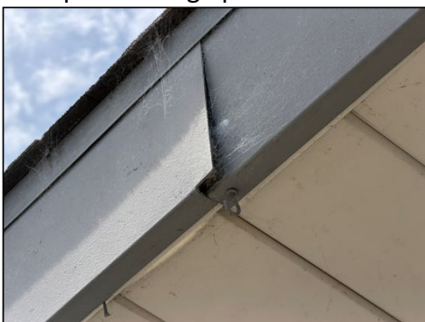
Missing/loose materials – service needed
