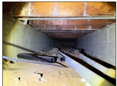
Debris present under structure - recommend removal of debris to allow for optimal ventilation
