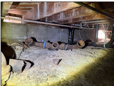
Debris present under structure - recommend removal of debris to allow for optimal ventilation
