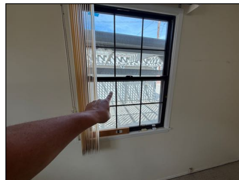
Broken sash cables or springs - unsafe - needs to be serviced
