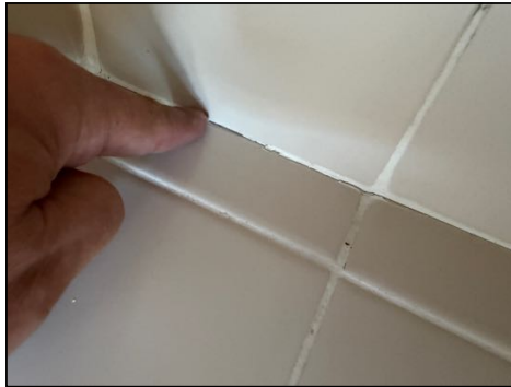
Cracked/loose/missing grout in areas – service needed
