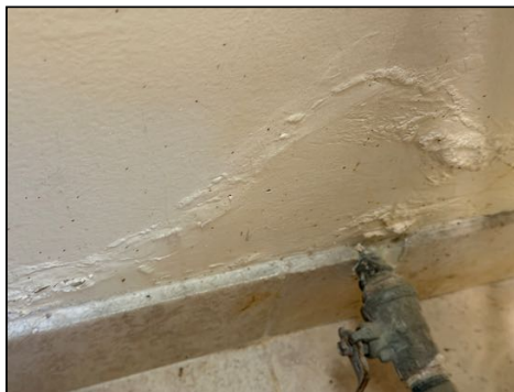
Stains at base - tested dry with moisture meter at time of inspection - monitor area for moisture
