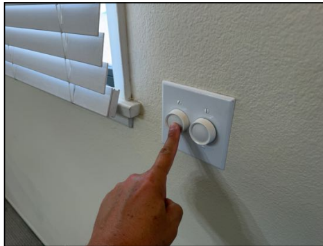
Dimmer switch not operating properly – service needed
