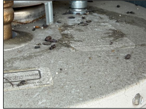
Evidence of rodents inside enclosure, on and around water heater
