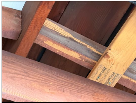
Wood deterioration observed - consult termite report for any wood areas in garage area
