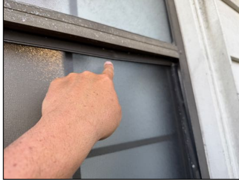
Torn/bent/worn screens - needs maintenance/repair
