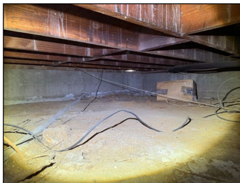
Debris present under structure - recommend removal of debris to allow for optimal ventilation
