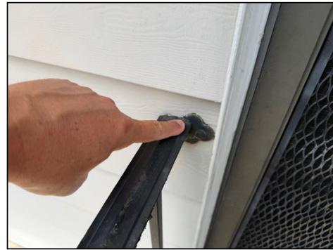
Worn/loose rails - typical for the age of the materials
