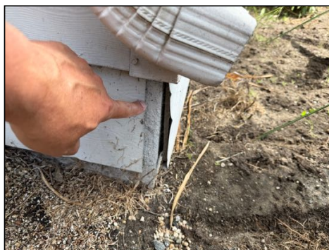
Missing/loose materials – service needed
