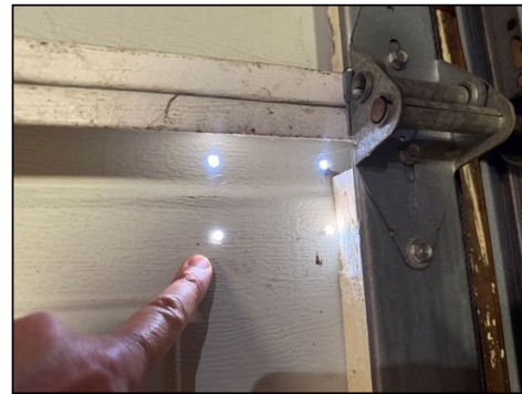
Holes present - repairs recommended, to prevent moisture intrusion
