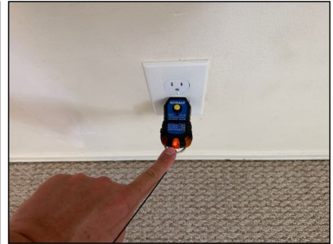
Three prong outlet(s) not grounded - needs to be serviced - ALL
