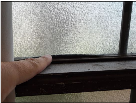
Inner seals at double pane windows are bulging/moving due to heat - needs to be serviced
