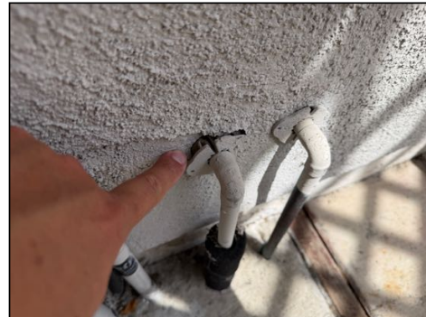
Recommend sealing any holes/gaps or cracks to prevent moisture or pest entry
