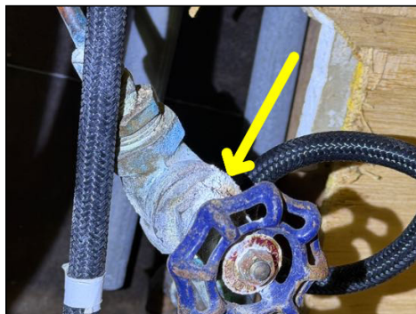
Shutoffs under sink corroded - needs to be serviced - this will be an ongoing maintenance issue for ALL plumbing valves
