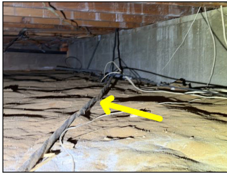
Wires/conduit lying on ground - potential hazard - needs to be serviced
