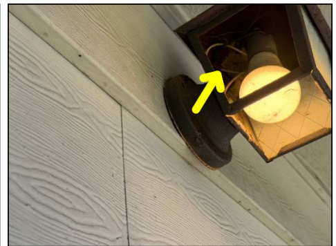
Fixture globes/covers damaged or missing – service needed
