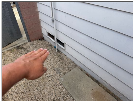
Grade slopes towards structure - needs to be serviced
