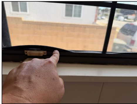
Inner seals at double pane windows are bulging/moving due to heat - needs to be serviced
