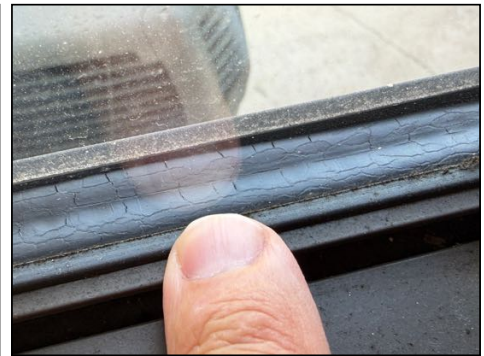
Inner seals at double pane windows are worn and cracked - signs of wear
