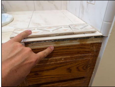
Missing/loose/damaged materials – service needed
