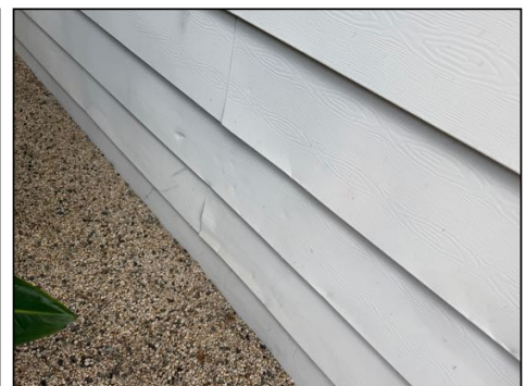
Impact damage present in areas
