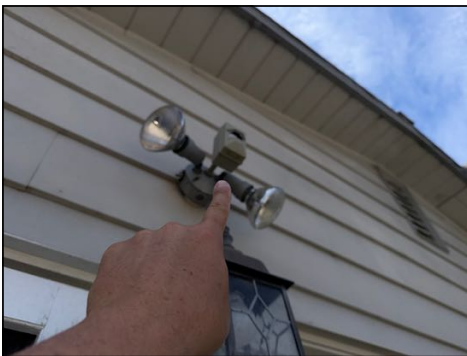
Some light(s) did not function (some may be on sensors or timers) - check bulbs first, then consult an electrician to further evaluate as needed
