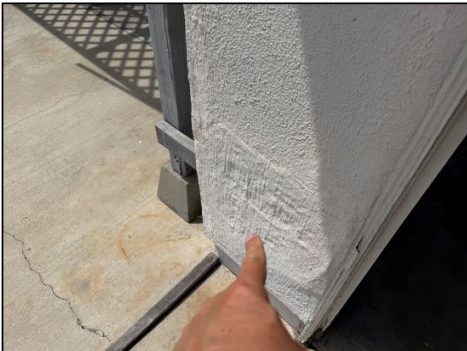
Patching present - consult seller for past repaired areas
