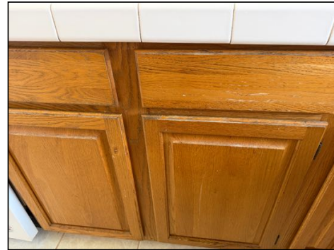
Worn/scratched/stained cabinets - typical for age
