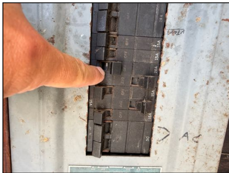
Breaker in off position
