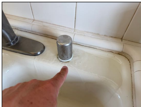
Water discharged out of air gap when draining - needs to be serviced
