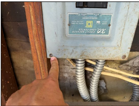
Panel cover screw(s) missing - recommend installing appropriate screws
