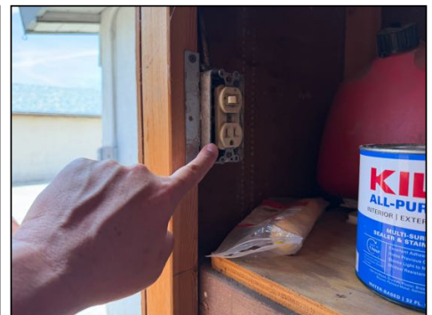
Outlet covers missing inside shed – service needed
