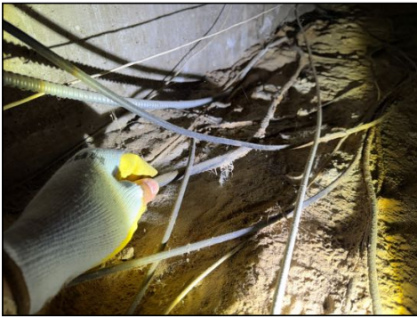
Wires/conduit lying on ground - potential hazard - needs to be serviced
