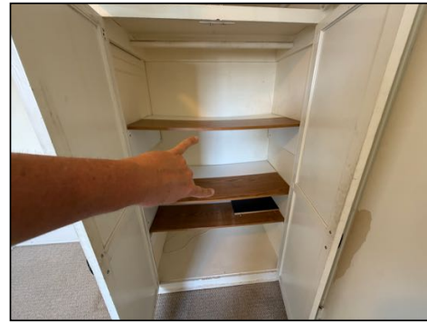
Shelving is sagging in areas
