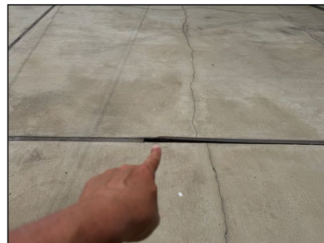
Displaced/lifted/uneven areas trip hazard - needs to be serviced
