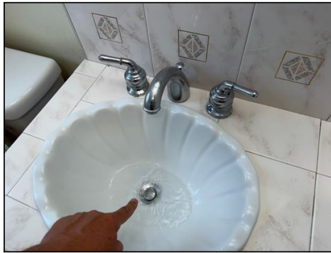
Drain operated slowly - needs to be serviced
