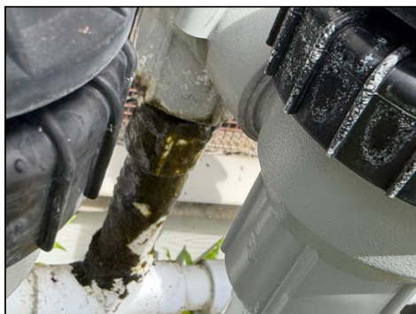
Leaking/evidence of leaking at valves – recommend servicing
