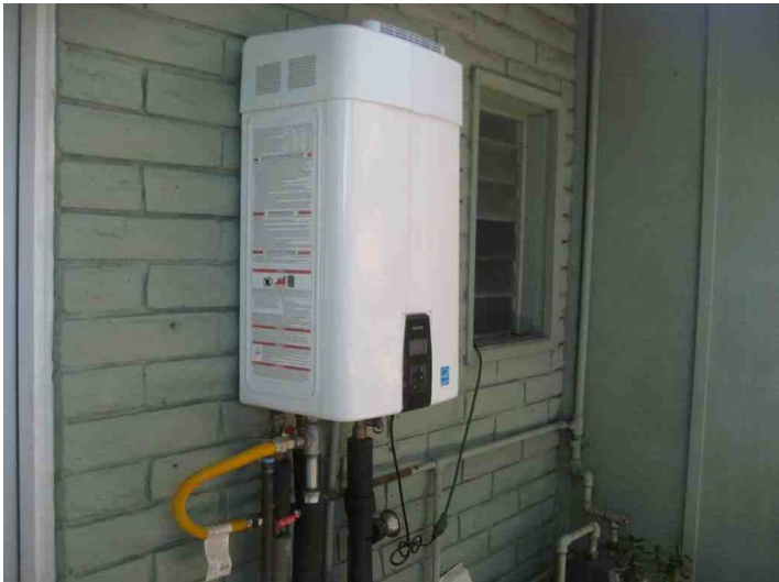
TANK LESS WATER HEATER
