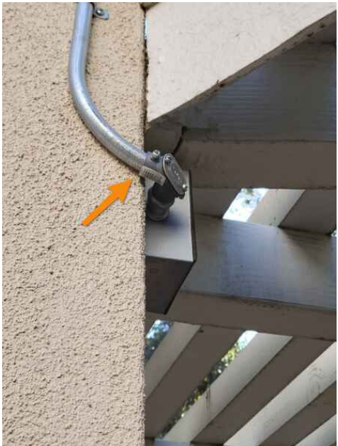
the exterior conduits are not installed with weatherproof fittings as required
