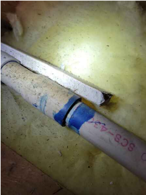
drainpipes are not properly glued and separating
