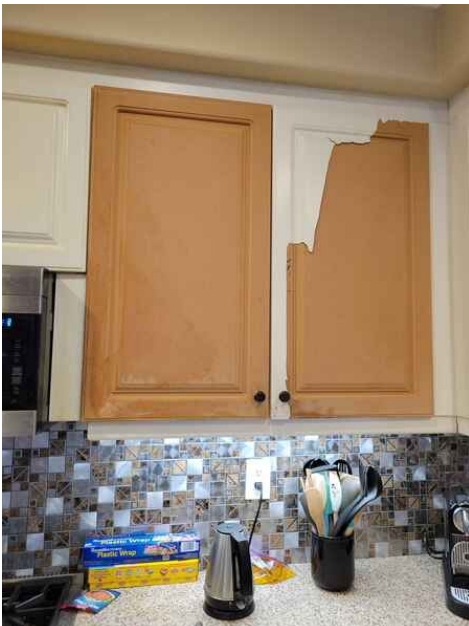
there is a complete thermofoil failure throughout
