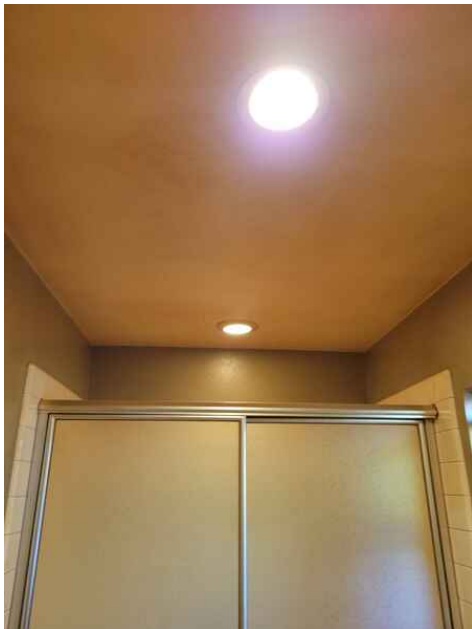
ceilings and walls coated with nicotine damage
