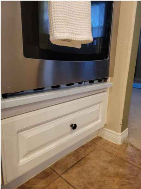
oven not installed to standards
