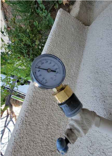
apprx 70psi at time of inspection
