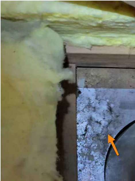
drip evidence from chimney
