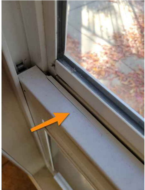
several of the single hung windows have this damage
