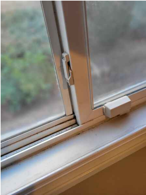
window not operating correctly
