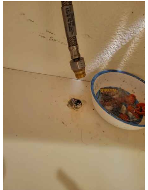
leak under faucet not fully installed
