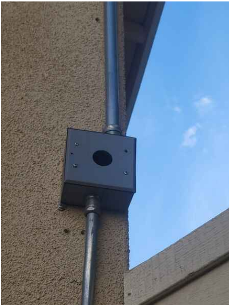
junction boxes open to weather
