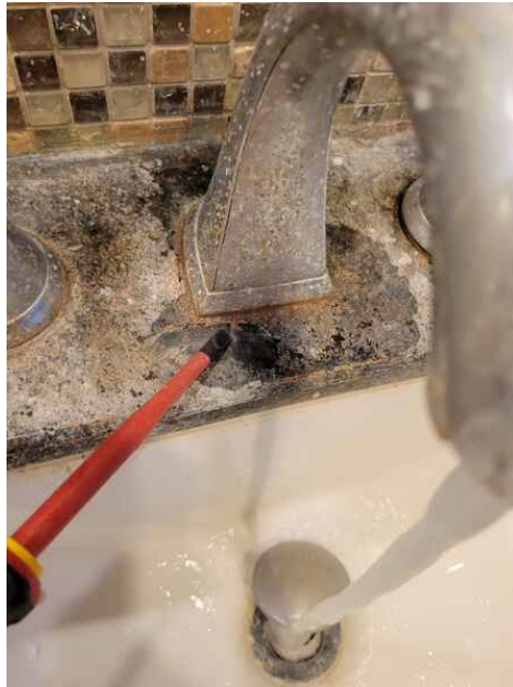
leak at base of faucet
