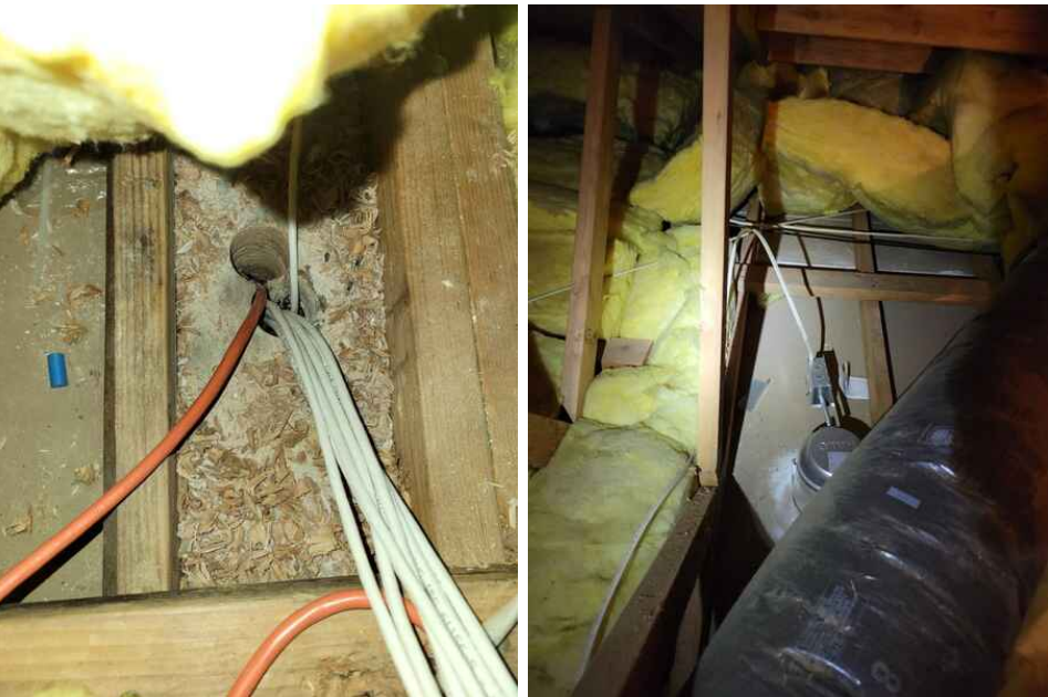
areas around all added recessed lights need improvement
