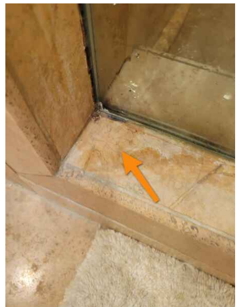
shower leaking at enclosure
