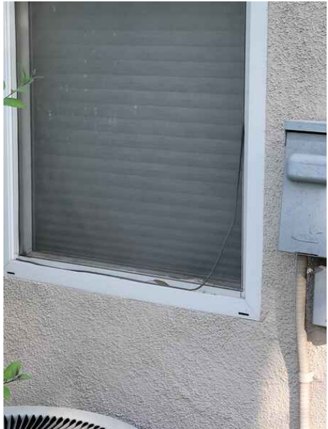
damaged screen and water damage
