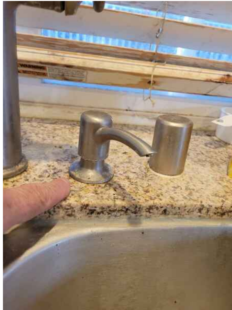
loose and leaking at base
