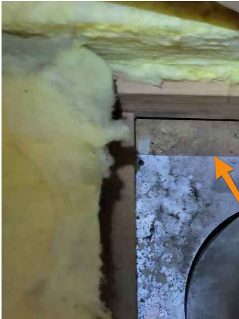
leakage from chimney
