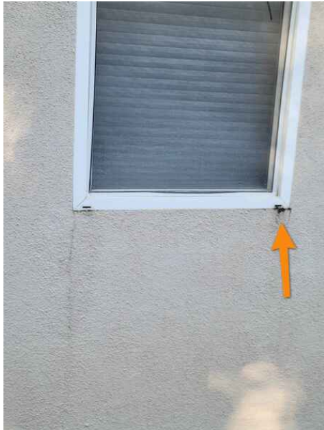
moisture intrusion from this area
