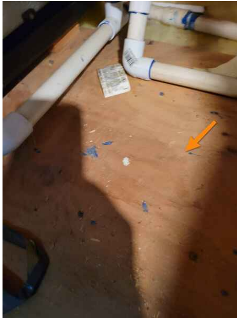
water staining around drain pipes
