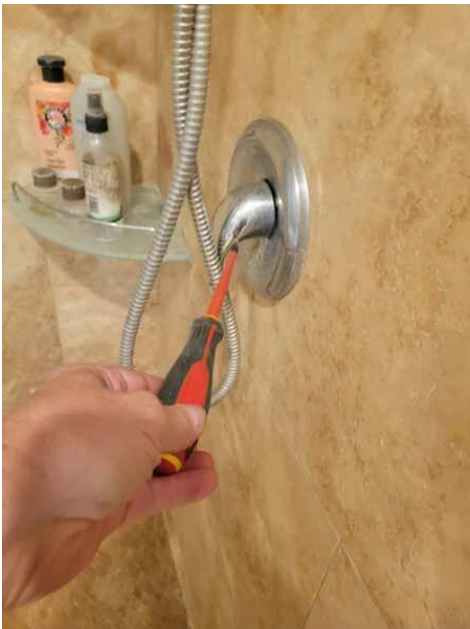
loose handle with leak from cartridge
