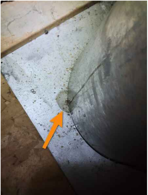
water pooling area
