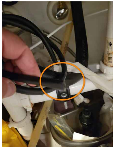
uncapped drain tube from previous reverse osmosis type system
