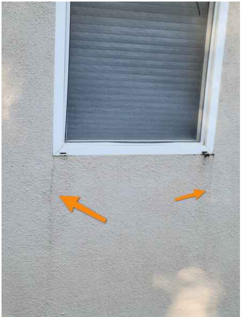
vertical cracking requires repair
