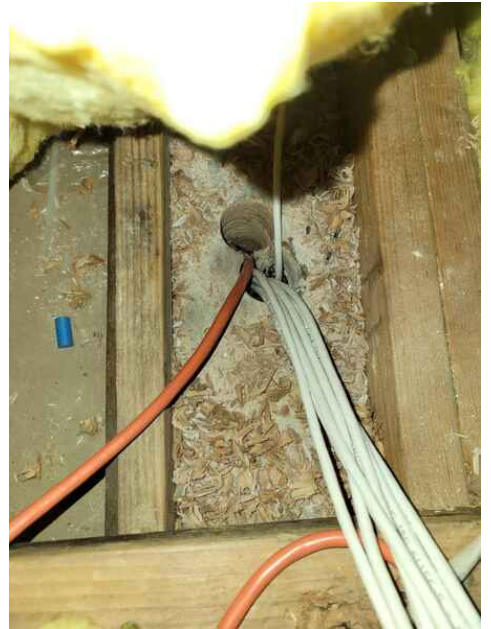
extension cord running between walls
