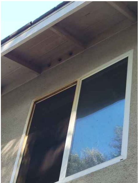
nicotine has affected the exterior in this area
