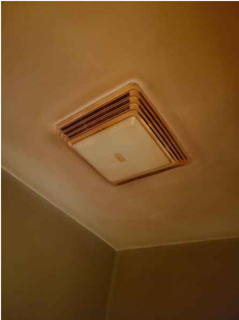
light not operating
