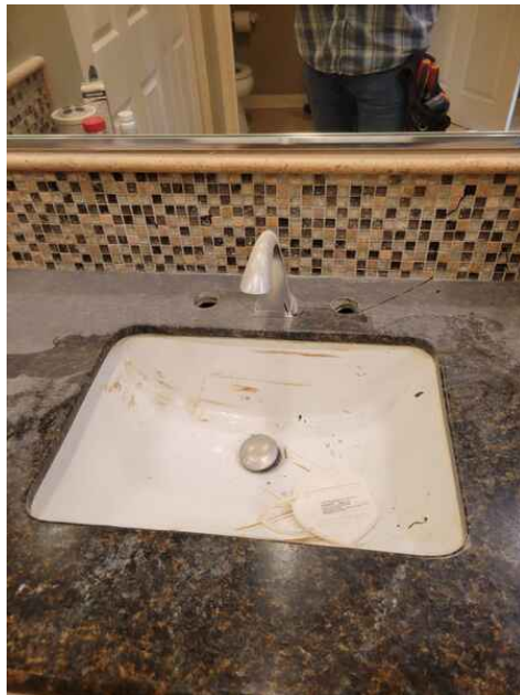
faucet not installed
