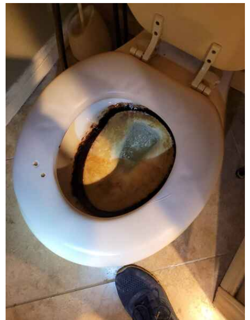
example of toilet bowl conditions
