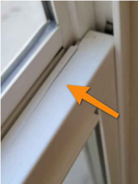
single hung windows are failing in this location throughout
