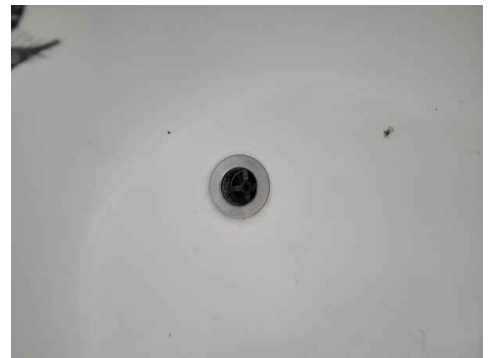
example of missing tub drain
