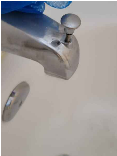
tub spouts are stuck in shower mode
