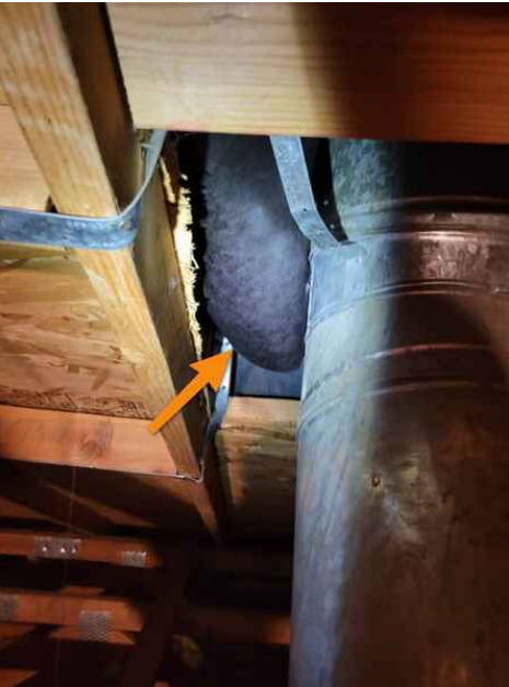
combustible material touching chimney pipe
