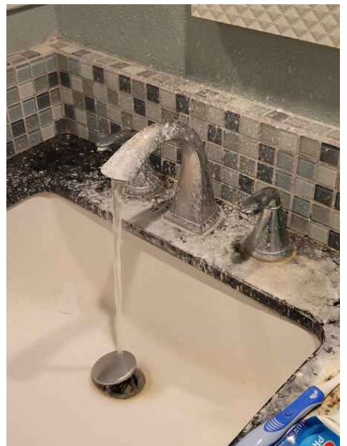
reduced flow and inoperable drain
