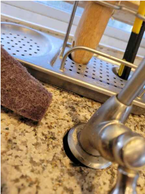
filtered water tap not connected to sink
