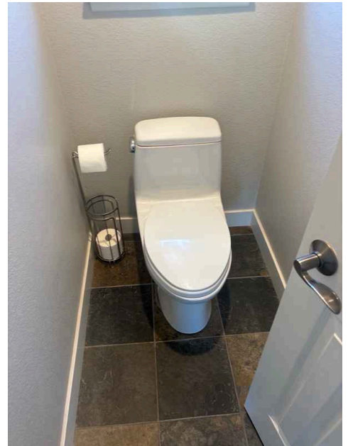
Running toilet causing flow meter movement
