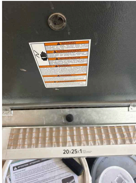
Air Conditioning: Approximate Age 26
