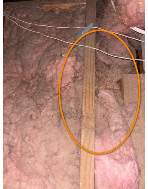
Termite dust in attic
