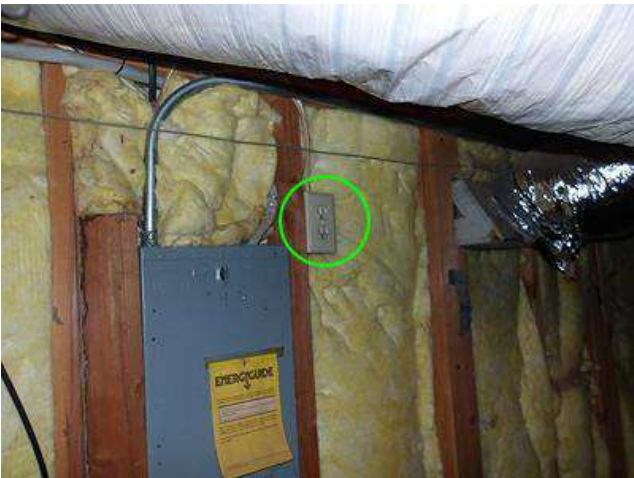
Photo 33-1 Crawl space near water heater
