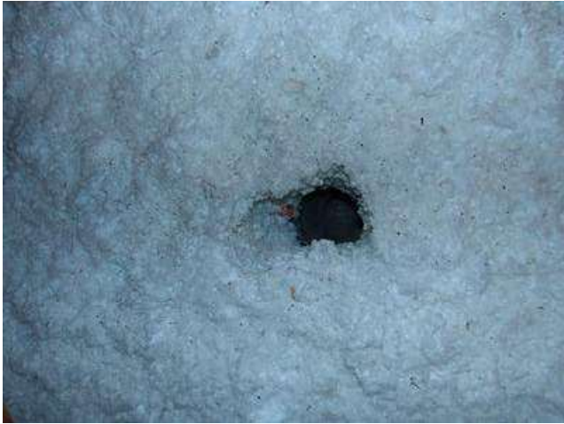
Photo 21-1 Hall bathroom exhaust fan termination
