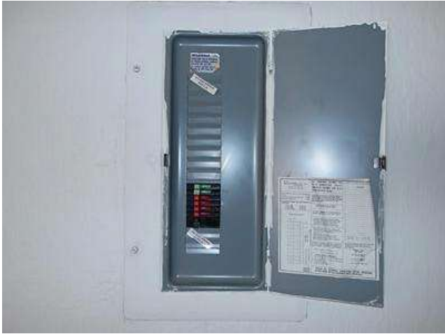
Photo 50-5 Sub panel basement
