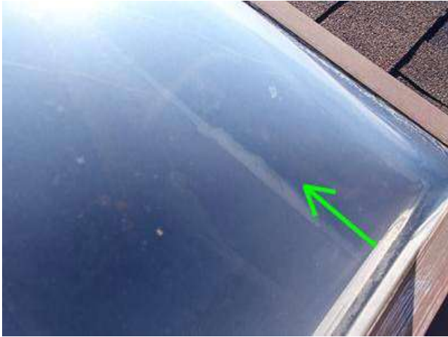
Photo 22-3 Skylight, interior substandard construction
