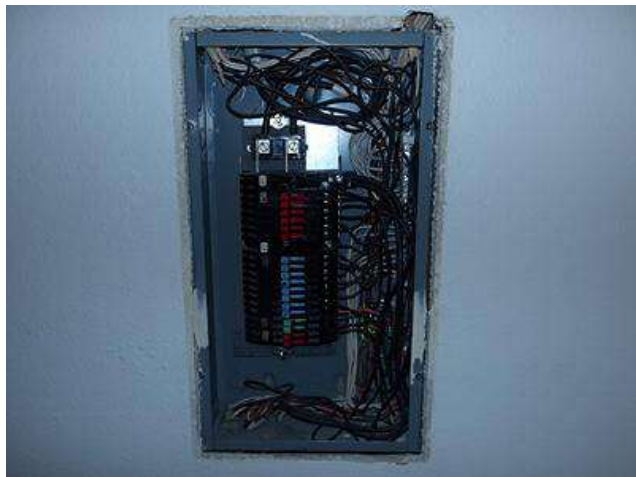
Photo 50-4 Sub panel closet
