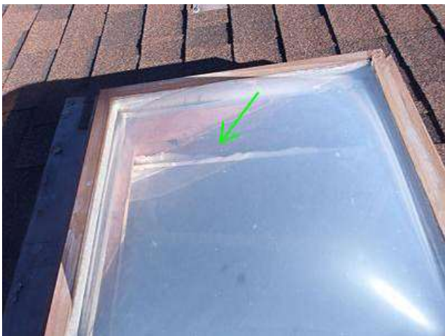
Photo 22-1 Skylight, interior substandard construction
