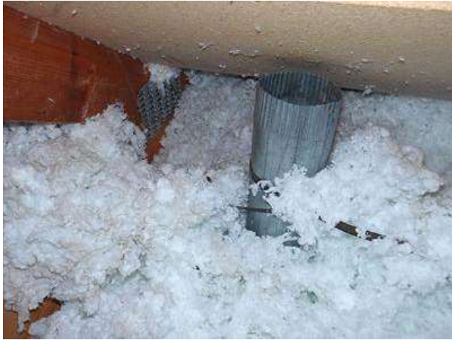
Photo 21-2 Laundry room exhaust fan termination
