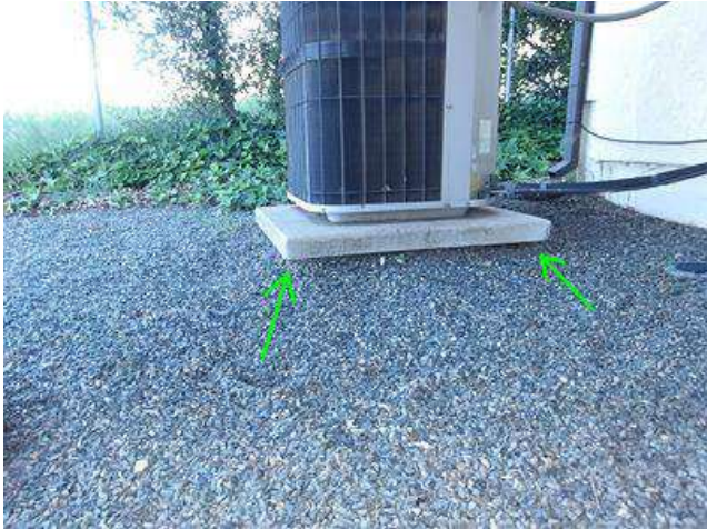
Photo 61-1 AC condenser pad
