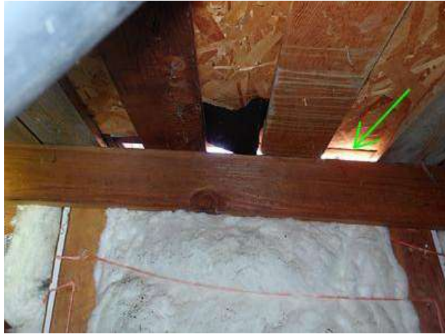
Photo 22-4 Skylight attic view (substandard construction)
