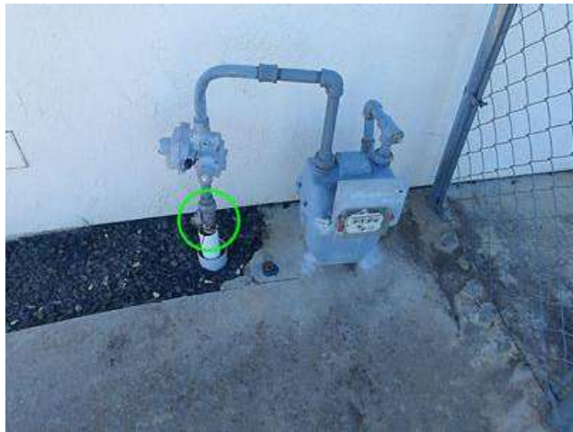
Photo 54-2 Gas shut-off, NE corner garage
