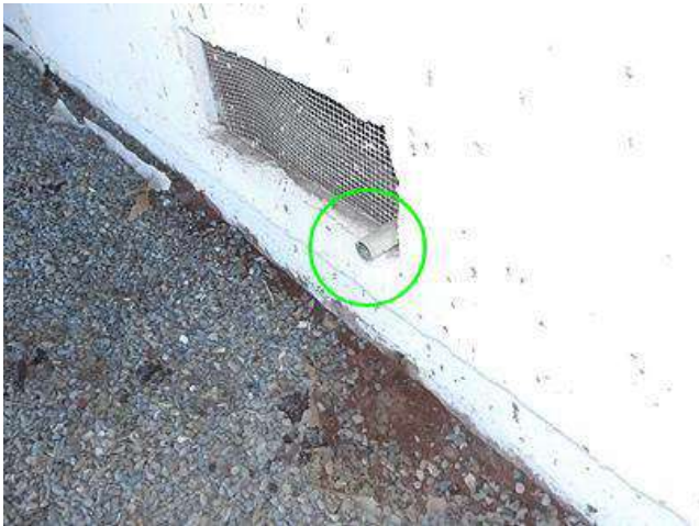
Photo 56-1 T&P drain line termination
