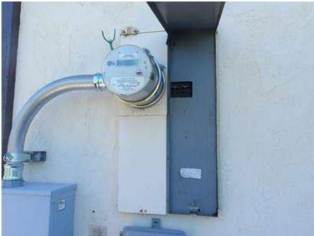
Photo 50-1 Meter & main panel
