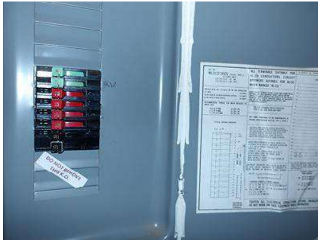
Photo 46-2 Sub panel basement
