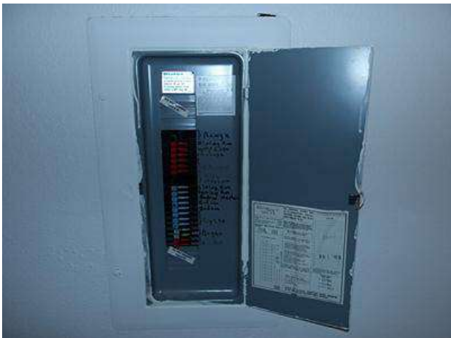
Photo 50-3 Sub panel closet
