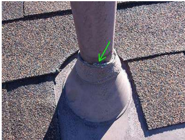
Photo 23-2 Plumbing vent above kitchen
