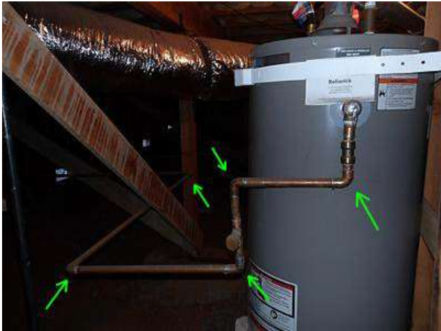
Photo 55-1 T&P drain line
