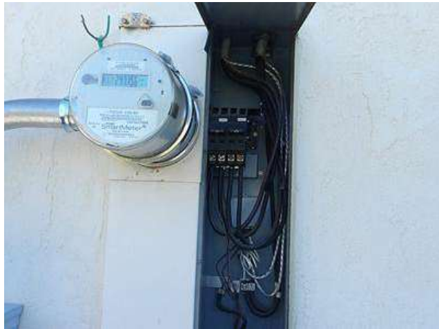
Photo 50-2 Meter & main panel
