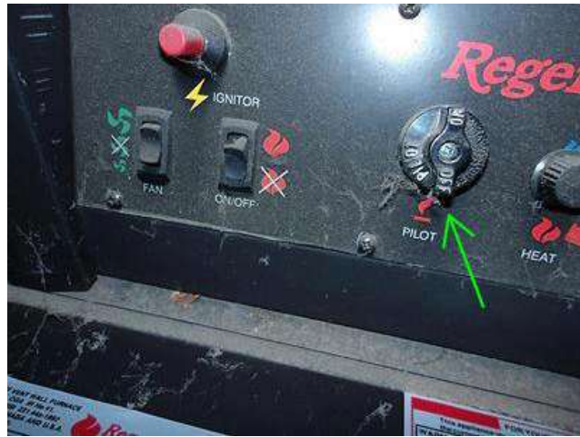
Photo 63-2 Pilot light off
