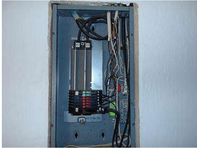
Photo 50-6 Sub panel basement
