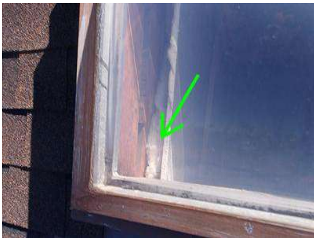
Photo 22-2 Skylight, interior substandard construction
