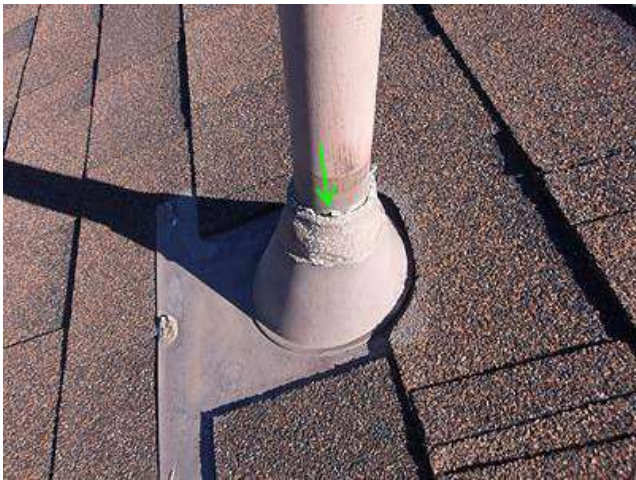
Photo 23-1 Plumbing vent above laundry
