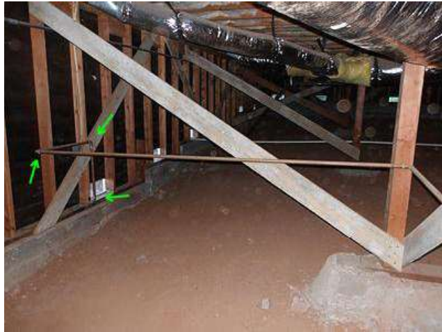
Photo 55-2 T&P drain line
