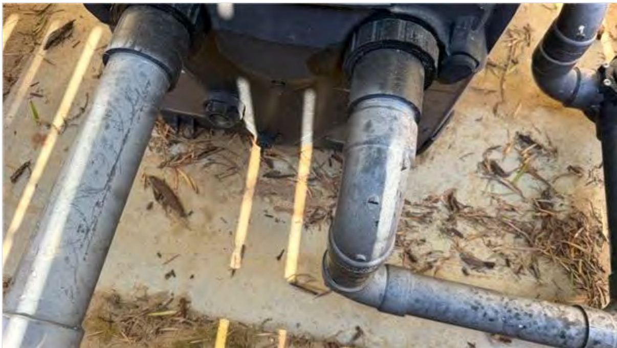
PVC Pipes to Heater
