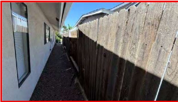
Wood Fencing is Leaning
