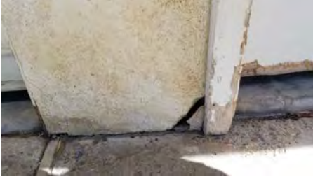
Physical Damage Due to Impact
