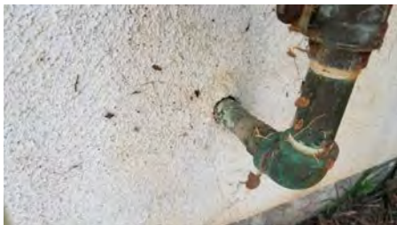
Gas Line Penetration Not Adequately Sealed
