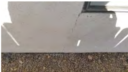
Cracking in Stucco
