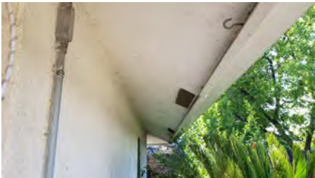
Stucco Intersection with Soffit
