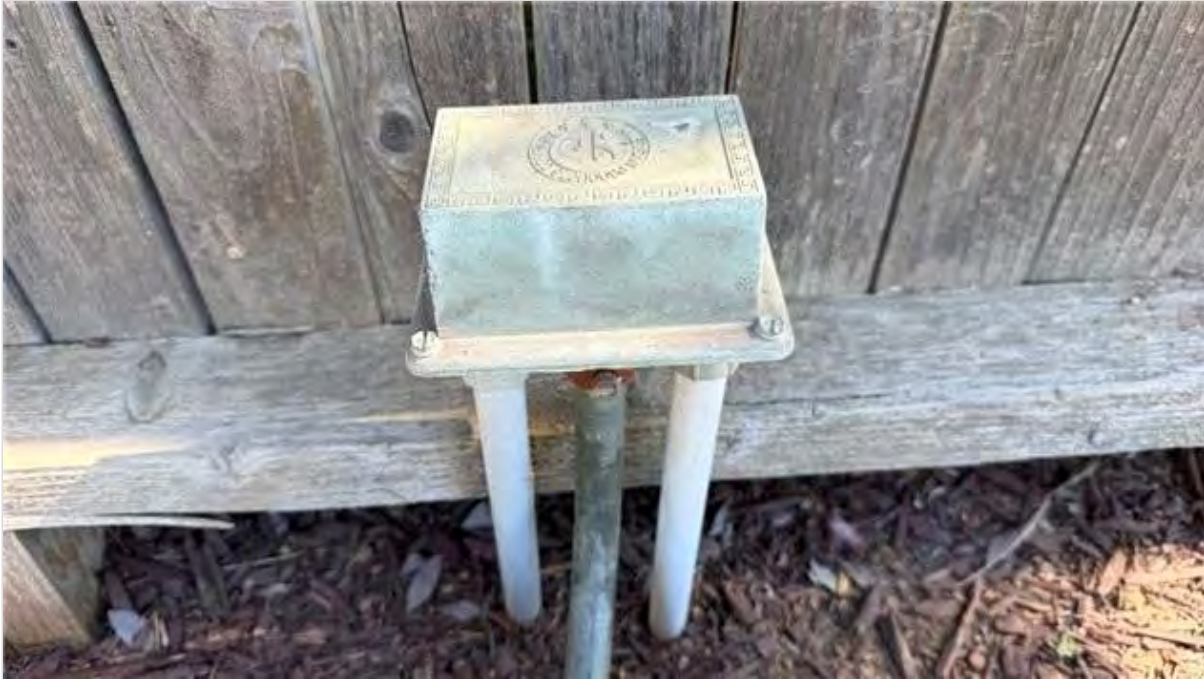
Pool Wet Nitch Box for Lighting Electrcial
