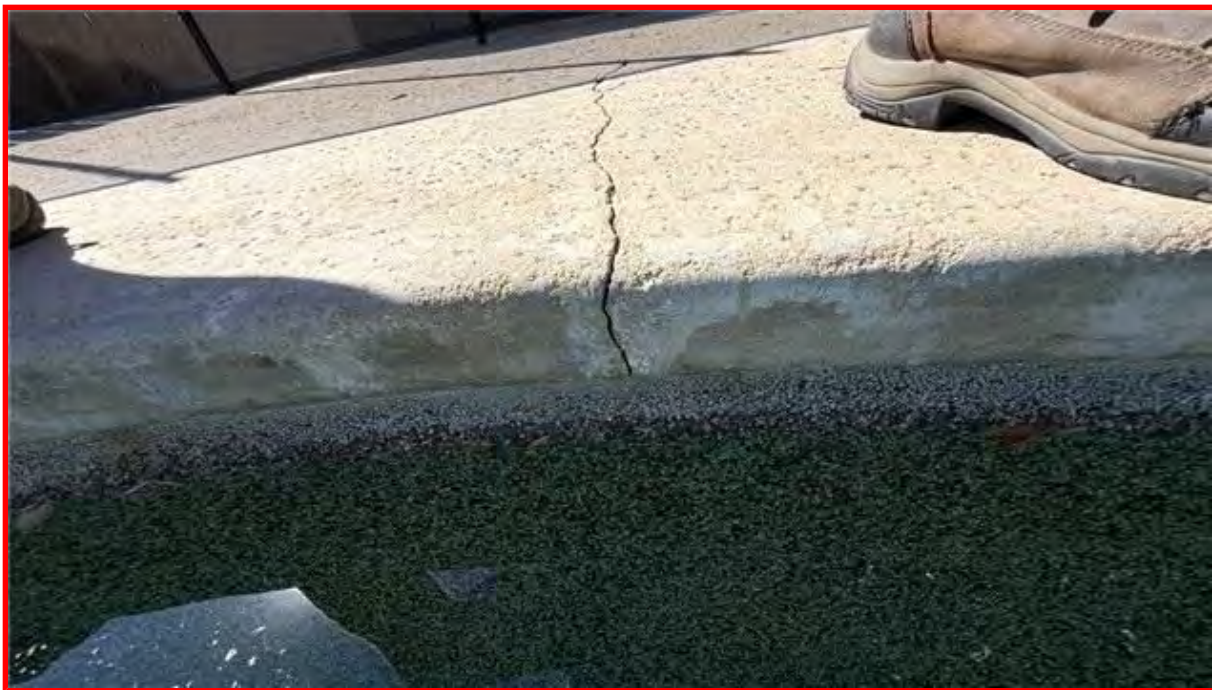
Crack at Decking
