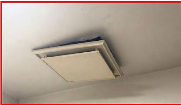
Half Bathroom Exhaust Fan Cover is Loose
