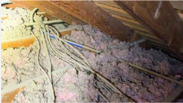
Previous Repairs at Copper Pipes in Attic
