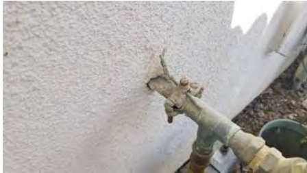
Pipe Penetration Not Adequately Sealed
