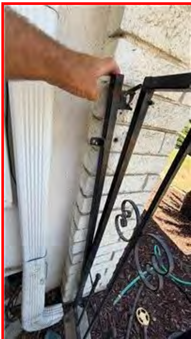
Front Yard Gate Loose / Broken Post
