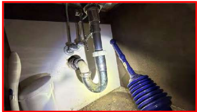
Half Bathroom Sink Leaks
