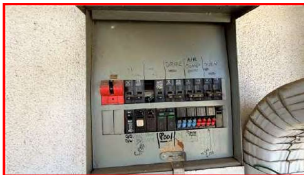
Open Breaker Slot in Electric Panel
