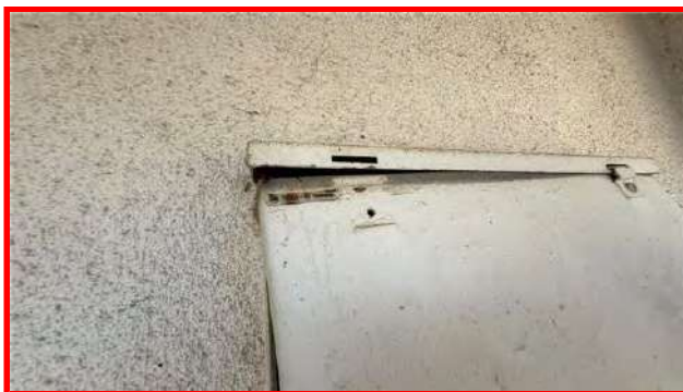
Hinge at Top of Electric Panel is Loose
