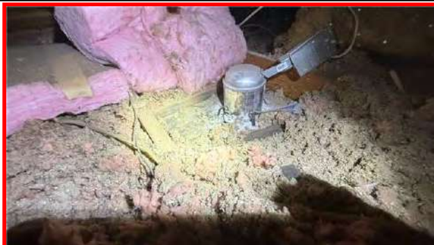
Moisture Stains / Damage on Top Side of Ceiling Drywall in Attic
