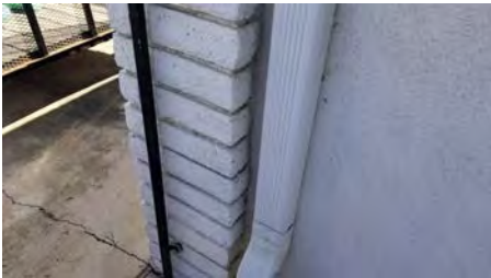
Brick Applied Directly Over Stucco Finish
