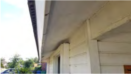
Stucco Intersection with Soffit
