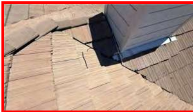
Cracked Roof Tiles Around Chimney
