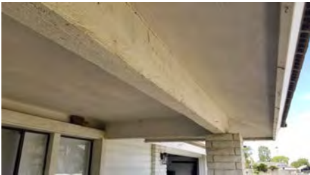
Stucco Intersection with Soffit
