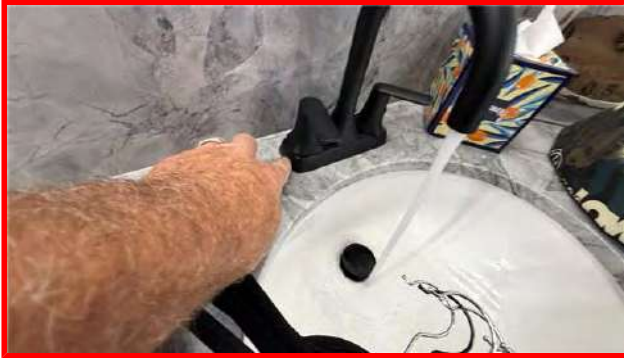
Faucet at Main Bathroom Sink is Loose
