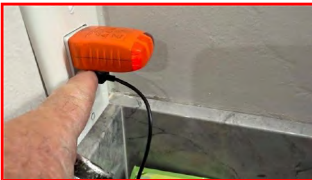
GFI Protection Missing at Main Bathroom Outlet
