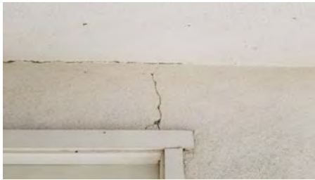
Cracking in Stucco
