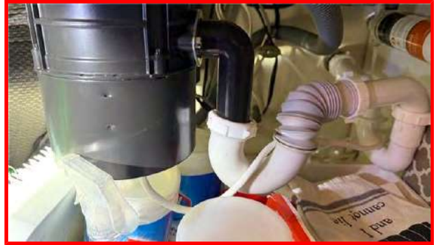
Improper Flexible Drain Pipe Below Kitchen Sink
