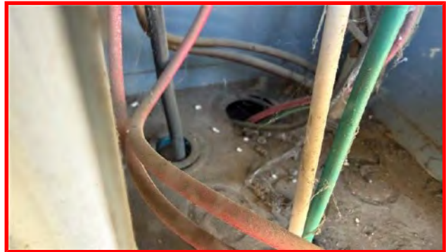
Open Knock Out in Open Breaker Slot in Electric Panel
