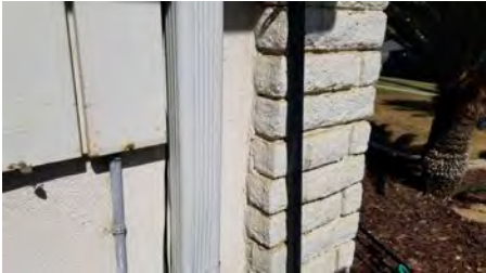
Brick Applied Directly Over Stucco Finish
