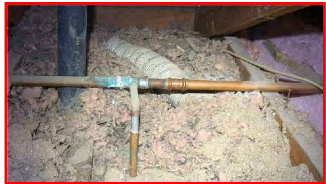
Copper Piping in Attic Corroded and Leaking
