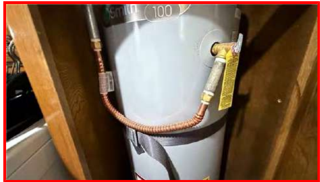
Water Heater TPR Improperly Runs Uphill
