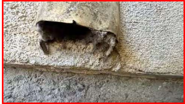
Dryer Vent Obstructed
