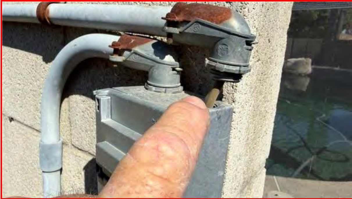
Electrical at Fencing Near Pool Equipment (Safety Issue)
