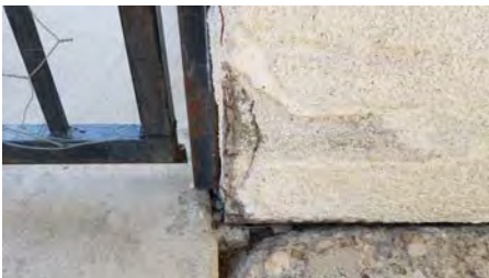
Physical Damage Due to Impact
