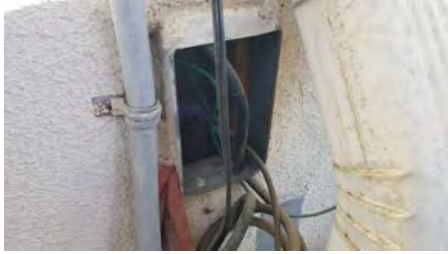
Media Panel Cover is Missing.
