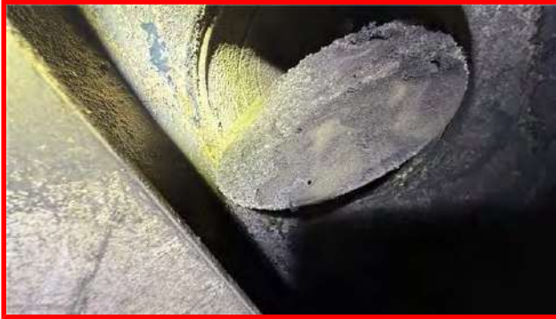
Soot Buildup and Debris in Fireplace Flue
