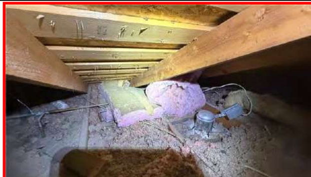
Moisture Stains / Damage on Top of Ceiling Drywall in Attic
