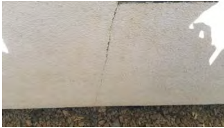
Cracking in Stucco
