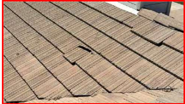
Cracked and Slid Roof Tiles
