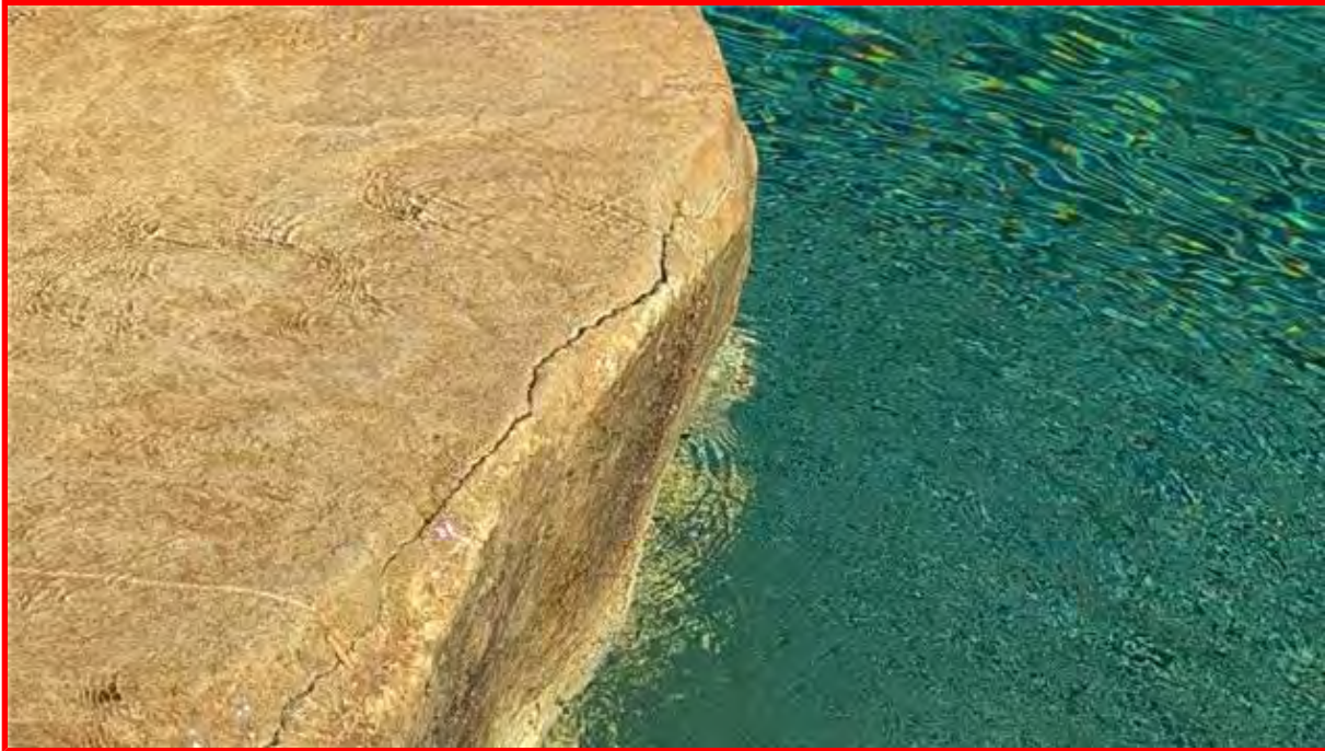
Crack at Spa
