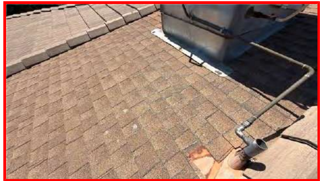
Shingles at South Side Roof Aged / Deteriorated
