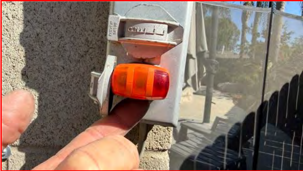
GFI Missing at Pool Area Fencing
