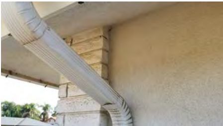
Brick Applied Directly Over Stucco Finish
