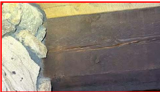
Cracks in Main Interior Beam in Kitchen
