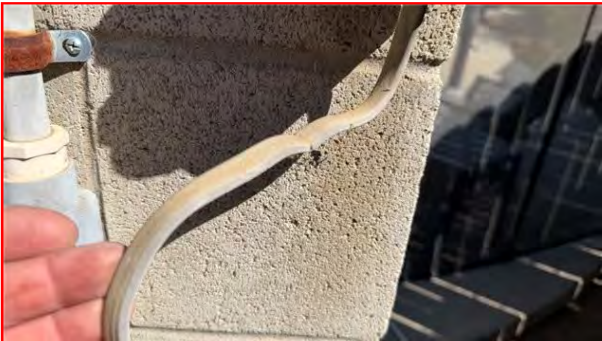
Exposed Wire Romex at Pool Area Fencing
