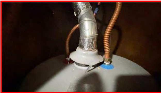
Water Heater Flue is Damaged and not Properly Centered at the Draft Hood
