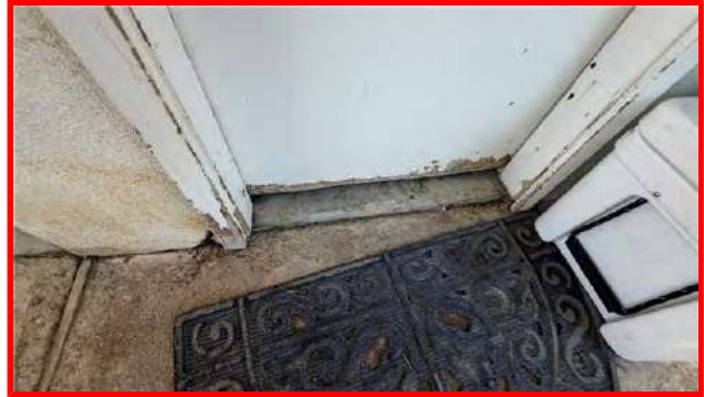
Rear Exterior Doors Deteriorated / Exposed
