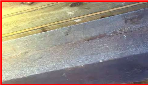
Cracks in Main Interior Beam in Kitchen
