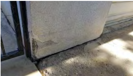
Physical Damage Due to Impact
