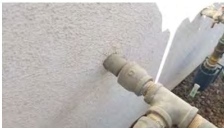
Gas Line Penetration Not Adequately Sealed
