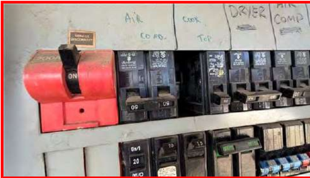
Open Breaker Slot in Electric Panel
