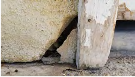
Physical Damage Due to Impact
