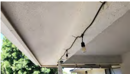
Stucco Intersection with Soffit
