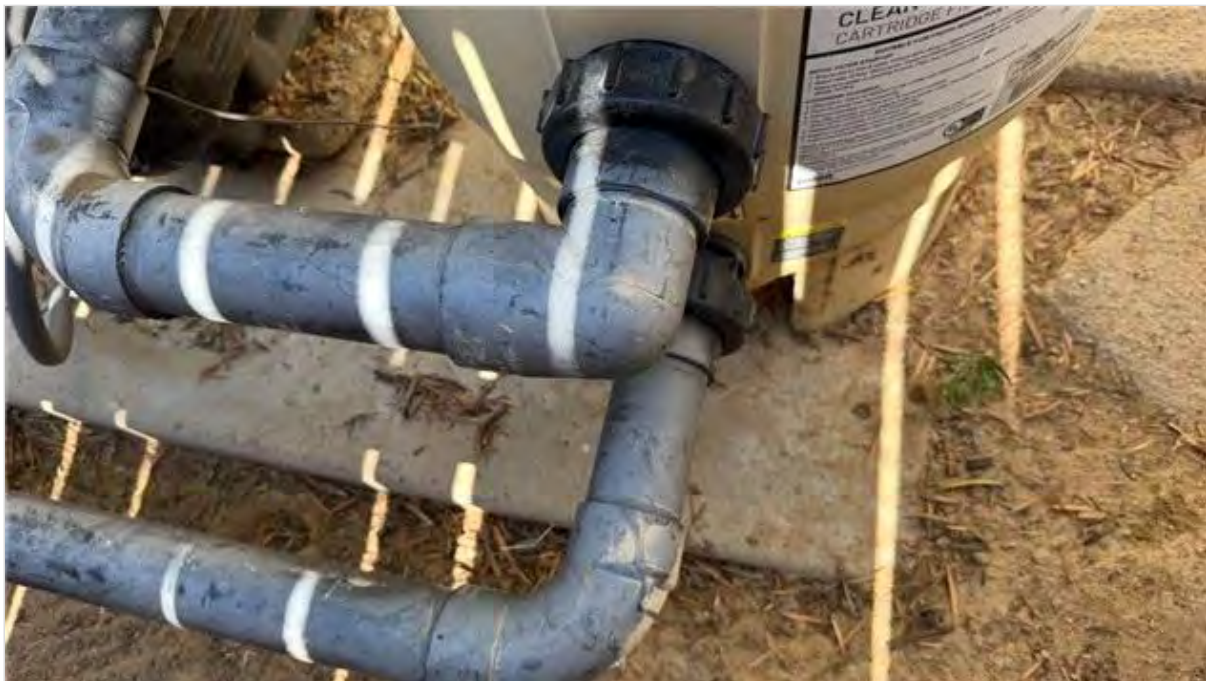
PVC Pipes at Filter
