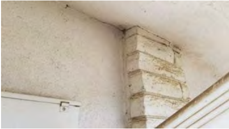
Brick Applied Directly Over Stucco Finish
