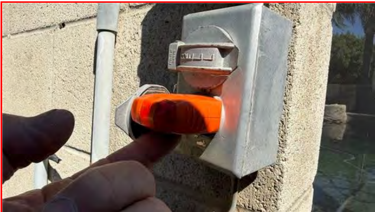
GFI Missing at Pool Area Fencing
