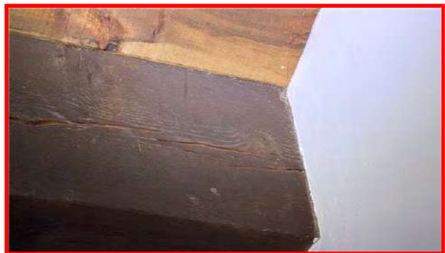
Cracks in Main Interior Beam in Kitchen
