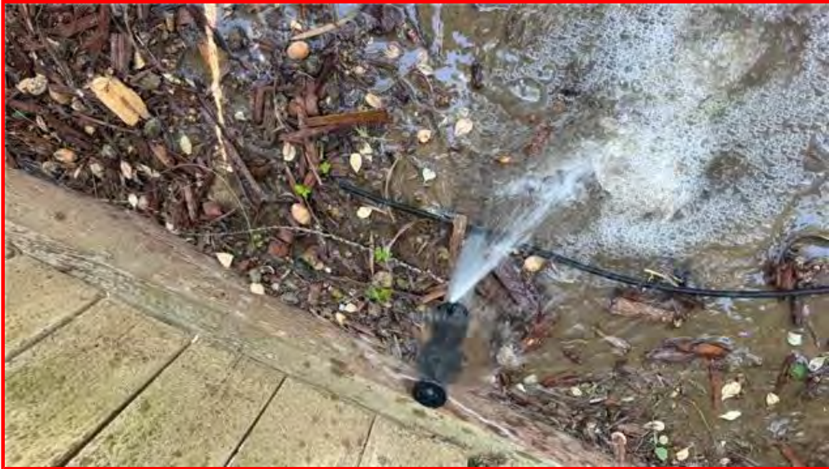
Leak at Rear Flowerbed Drip Line
