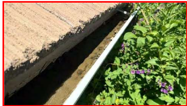
Gutters Clogged with Debris
