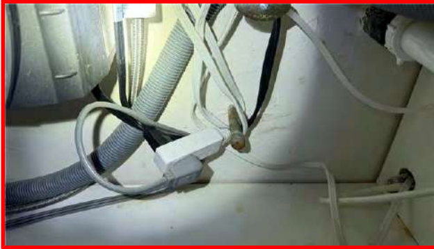
Extension Cord Wiring Improperly Being Used in a Permanent Manner Under Kitchen Sink
