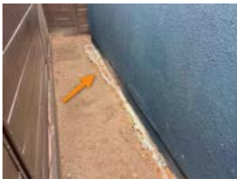
Garage Left Exterior
