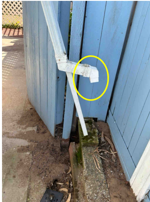
Improper termination of the carport awning downspouts
