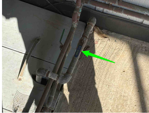
Main gas shut off valve
