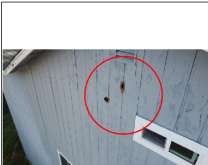
Siding has significant damage, recommend repair
