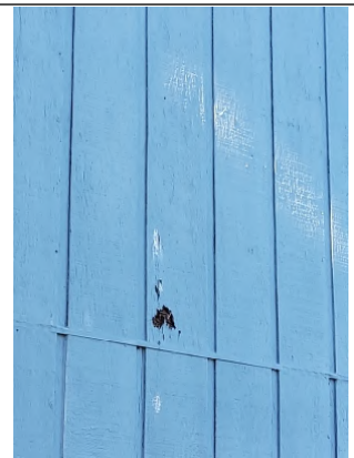
Siding has significant damage, recommend repair
