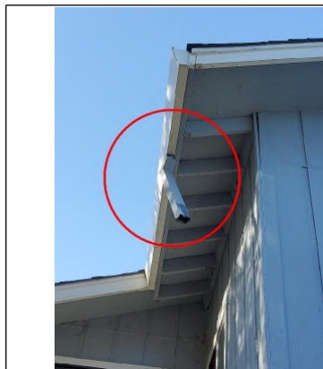
New downspout that spans to the bottom is needed, recommend repair
