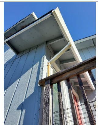
Significant rust is evident on downspout, gutters are nearing end of life, recommend replacing
