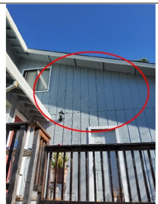
Siding at section is warped, recommend having replaced by a licensed contractor.
