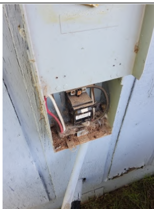
Missing cover, recommend repair
