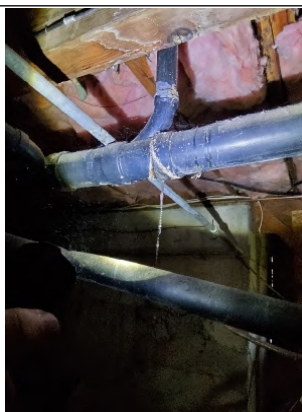
Active plumbing leak, recommend repair
