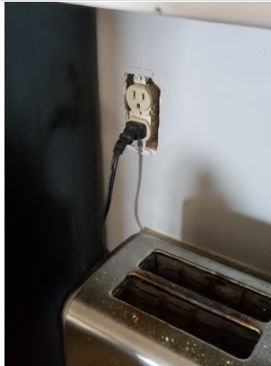
Missing cover plate, recommend repair
