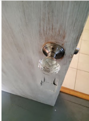
Damaged door slab, recommend replacing
