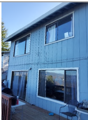
Siding at section is warped, recommend having replaced by a licensed contractor.
