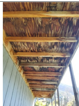
Cover installed over units is not structurally sound, recommend new posts minimum 4x4 be installed to replace 2x6. Also roll asphalt should be installed over new wood sheathing to replace existing.
