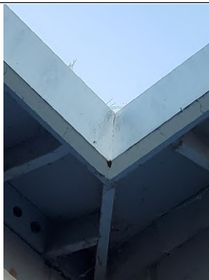
Active leak is evident on gutter, recommend replacing
