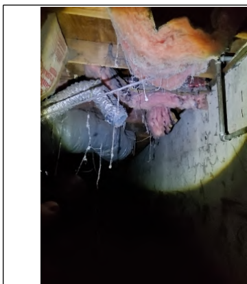
Dryer vent disconnected, recommend repair
