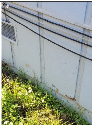
Siding has significant damage, recommend repair
