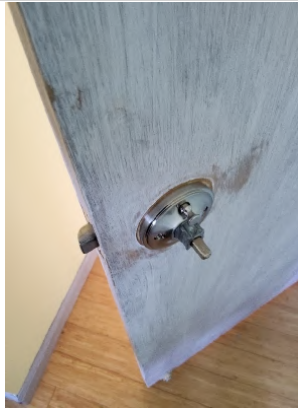
Missing door hardware, recommend installing new one
