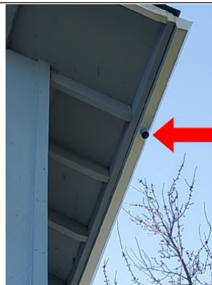
Missing downspout, recommend repair
