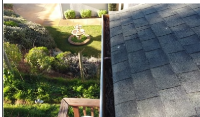
Gutter is full of debri and rusting, recommend cleaning
