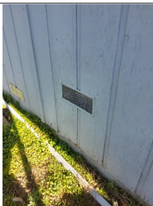
Siding has significant damage, recommend repair
