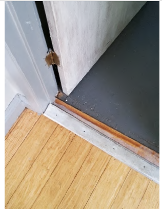
Threshold is loose, recommend fastening
