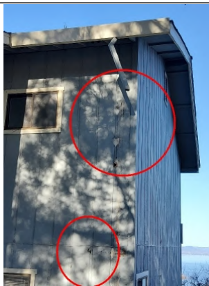
Siding has significant damage, recommend repair
