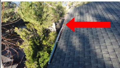
Gutter is full of debri and damaged, recommend repair
