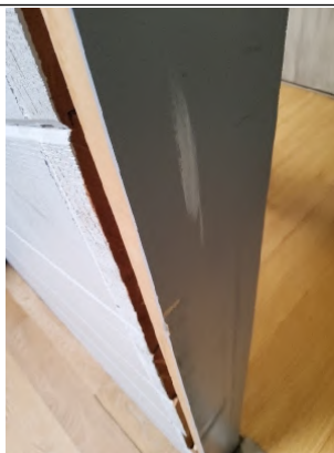
Missing door latch hardware, recommend repair
