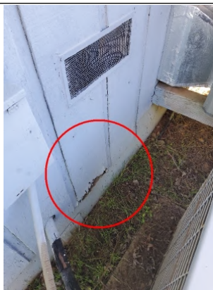
Siding has significant damage, recommend repair
