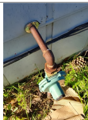
Rust is evident on gas line, recommend further evaluation and repair by a licensed plumber
