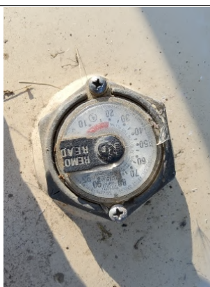
Propane tank is 80 percent full during time of inspection.
