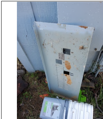
Cover is missing screws, recommend repair
