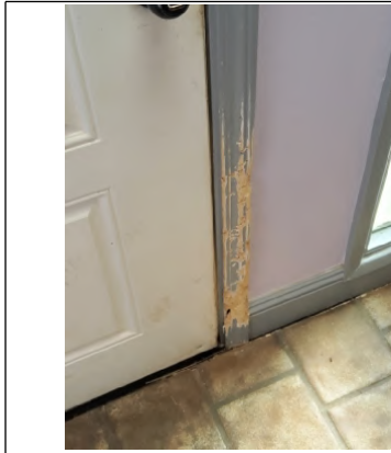
Recommend replacing damaged trim
