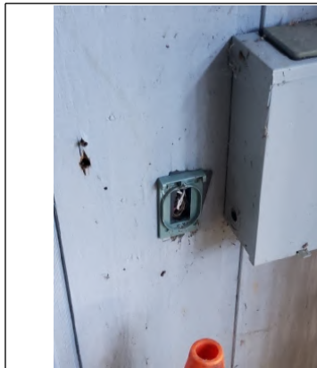
Broken outlet, recommend repair by a licensed electrician.
