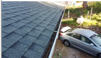
Gutter is full of debri and rust, recommend cleaning
