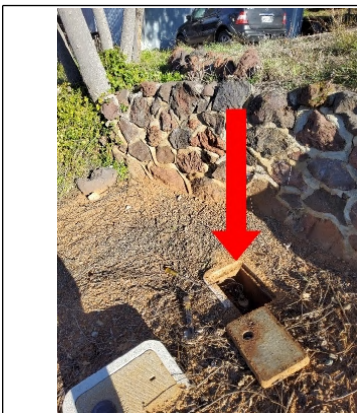
Water meter location
