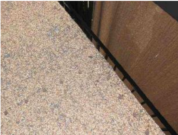
Patio cover roof improperly installed with nails.
