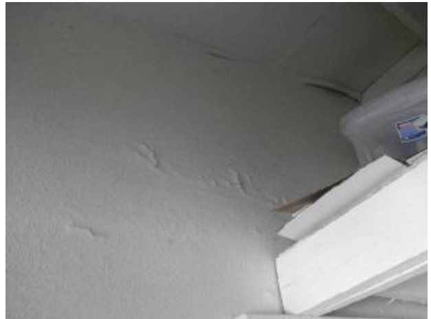
Peeling paint inside the garage.
