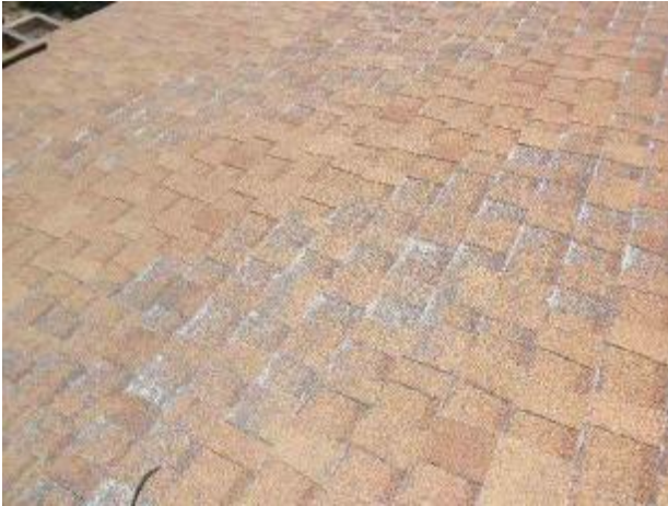
Example of deteriorated roof shingles.
