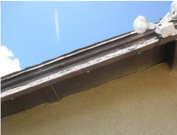
Painting needed at the south fascia boards.
