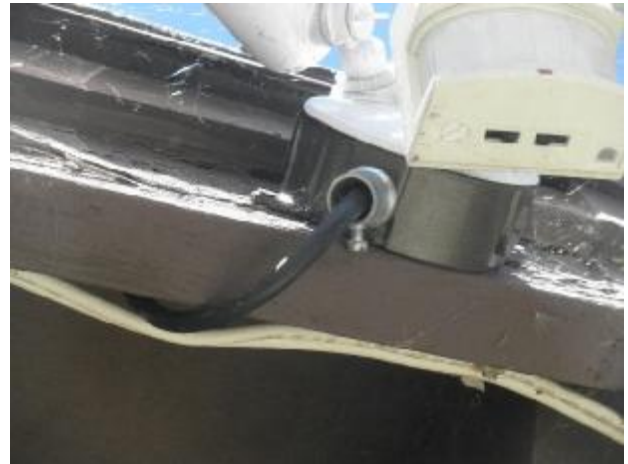
Moisture damage at the south fascia board.
