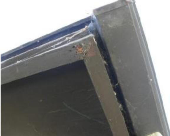
Moisture damage at the fascia boards.
