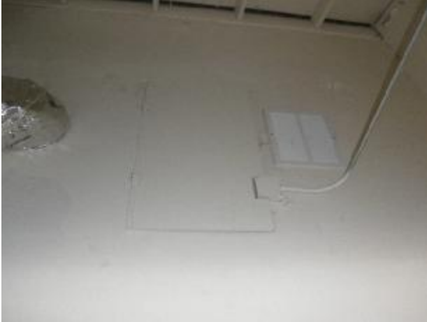
Peeling paint inside the garage.
