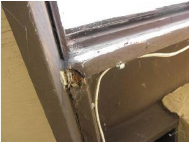
Moisture damage at the south fascia board.
