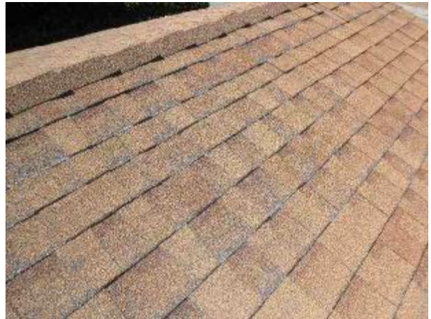
Example of deteriorated roof shingles.
