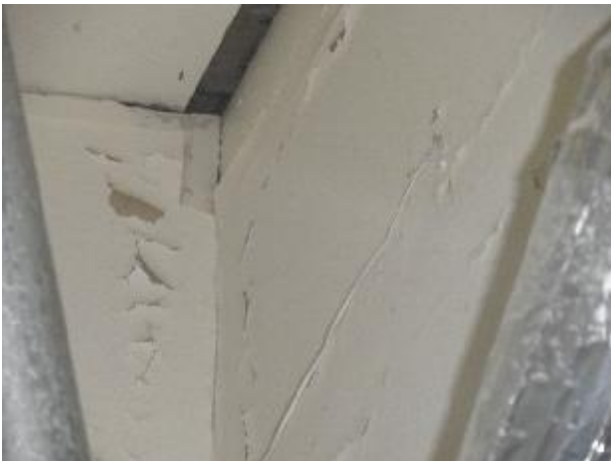
Peeling paint inside the garage.
