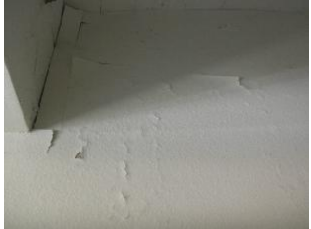
Peeling paint inside the garage.
