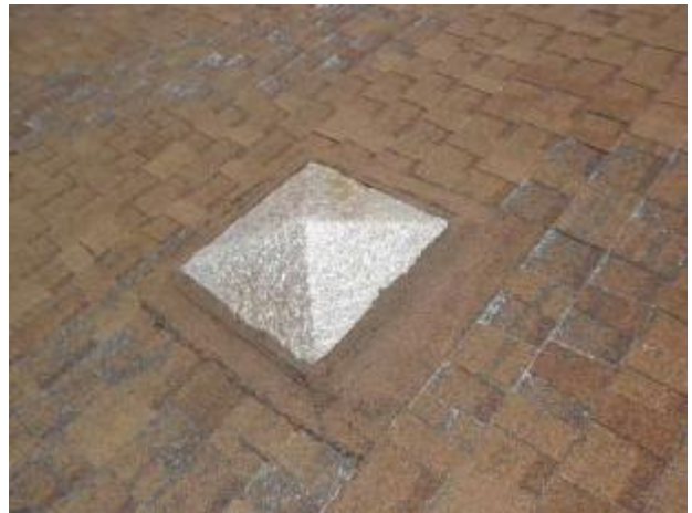
Skylight improperly installed with no visible flashings.
