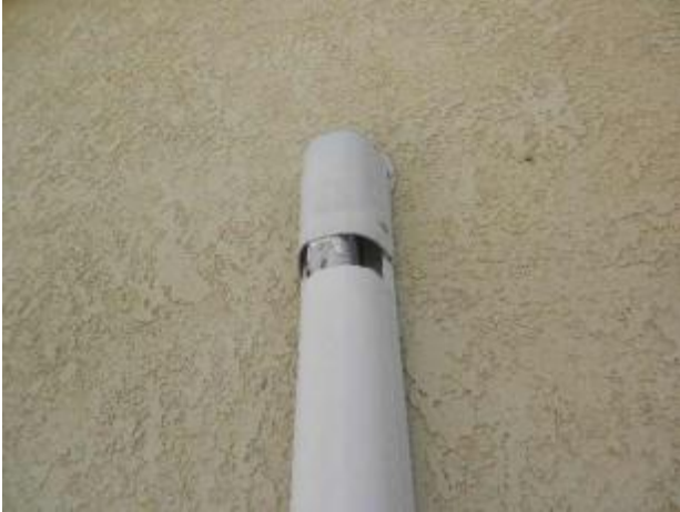
Plastic conduit for the A/C system has separated.
