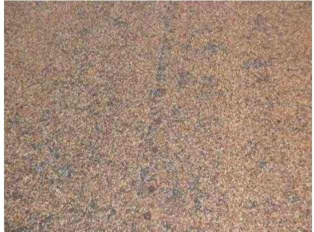
Patio cover roof improperly installed with nails.
