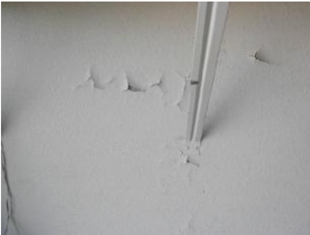
Peeling paint inside the garage.
