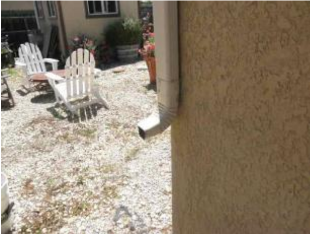
Down spouts should terminate away from the home.
