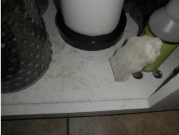
Minor moisture damage to the kitchen sink cabinet.
