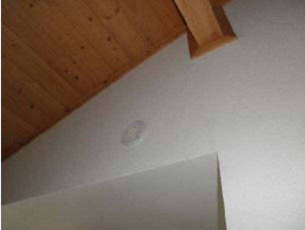
Missing smoke detector outside of the bedrooms.
