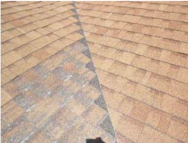
Example of deteriorated roof shingles.
