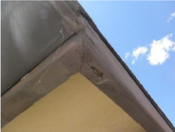
Moisture damage at the SE patio cover.
