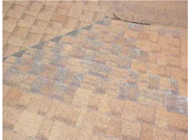
Example of deteriorated roof shingles.
