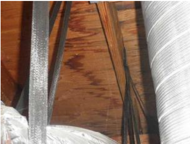
Evidence of leaks around the skylight.
