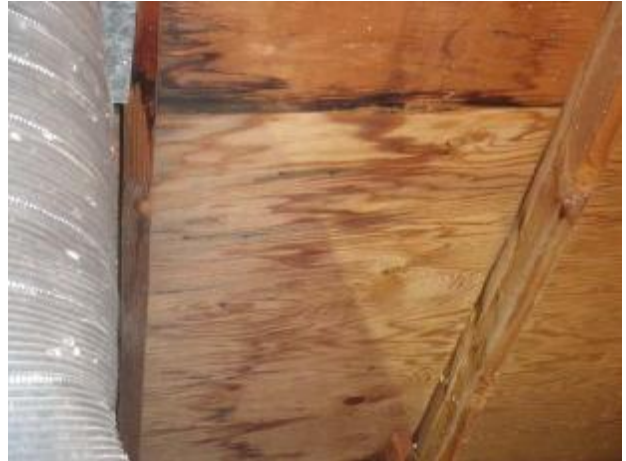
Evidence of leaks around the skylight.
