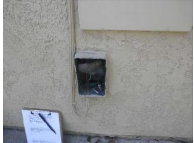
TV box cover is missing.
