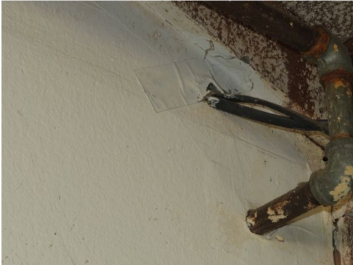
romex wire runs through a firewall
