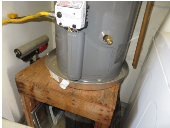
missing drain line at the drip pan, does not extent to the exterior
