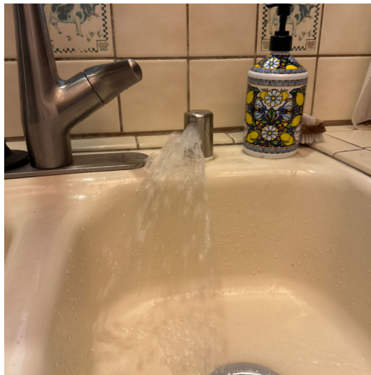
water discharged out of the air gap while draining
