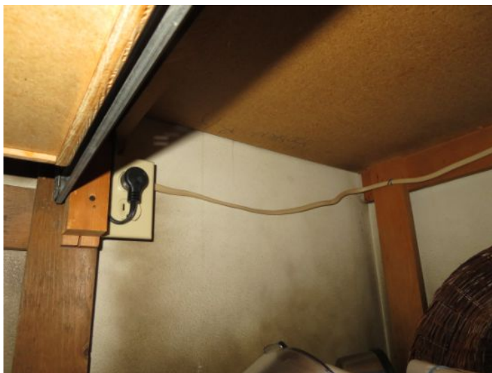
romex wiring in the cabinet
