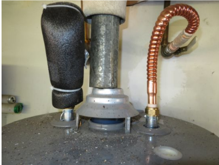
loose connection at the draft diverter
