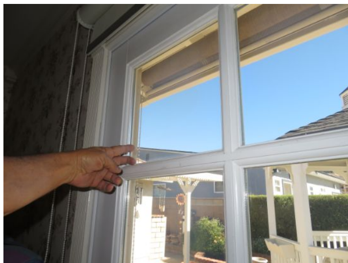
condensation present between the glass
