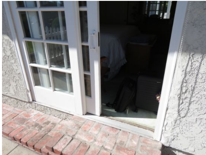
sliding screen door is missing
