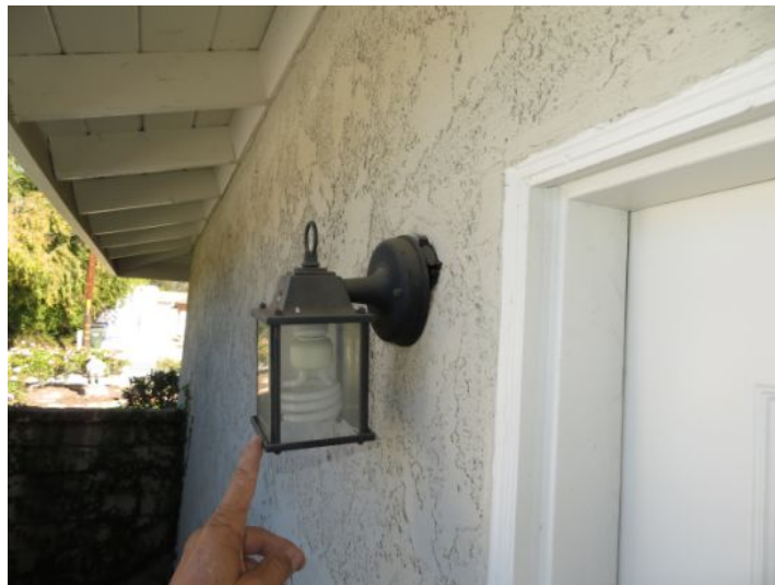
loose light fixtures
