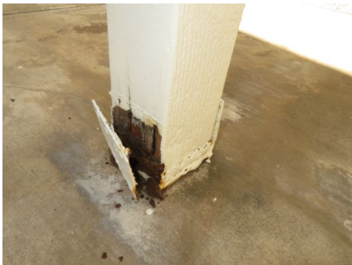
rusted and broken post ties
