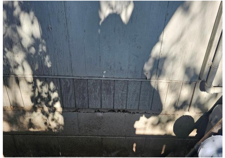
3A - Damaged siding.
