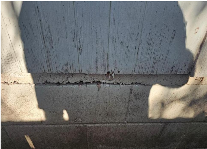
3A - Damaged siding.
