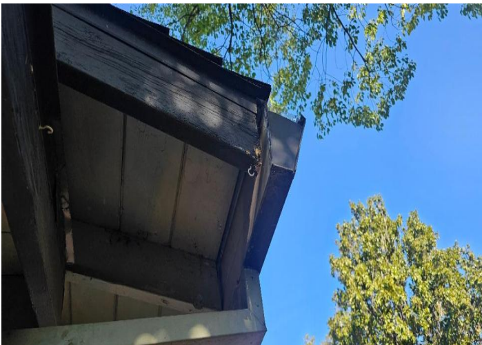
3B - Damaged roof rafter.
