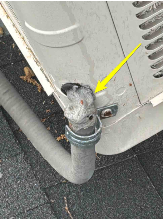
Improper, unsafe conduit connection
