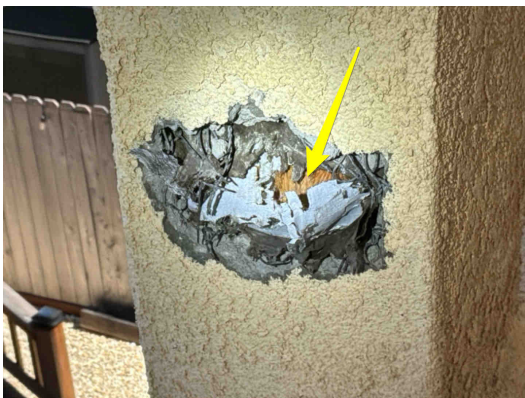
Support post Stucco damage
