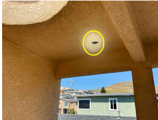
Ceiling stucco damage
