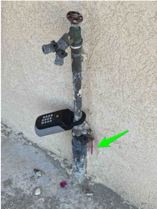
Main water shut off
