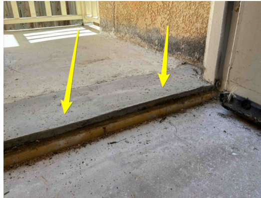
Concrete installed too high above the door threshold
