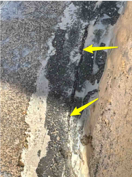
Current sealant heavily deteriorated
