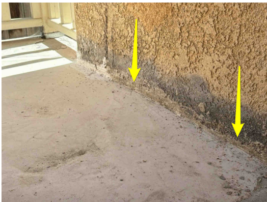
Concrete outside the pedestrian door improperly installed too high at the exterior stucco
