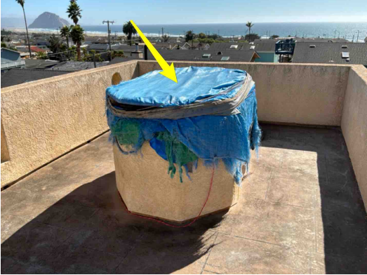
Suspected past roof leakage. Area appears to been covered with a tarp
