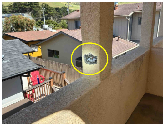
Support post Stucco damage
