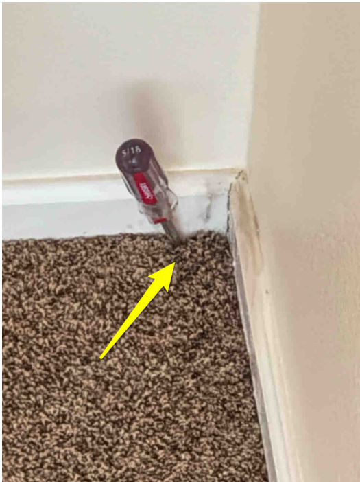
Shows the excessive damage of the wood subfloor
