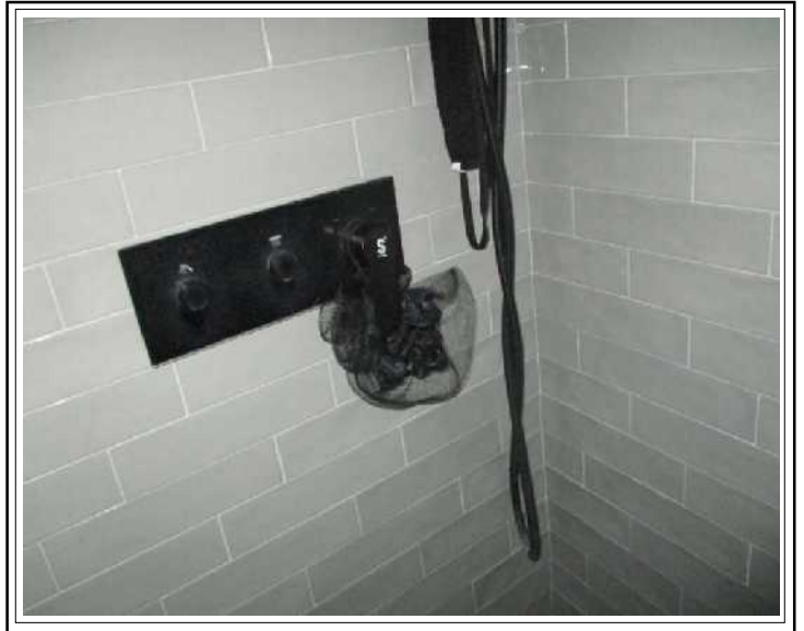
high end fixtures
