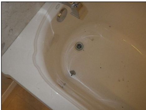
Drain stopper not operating - needs to be serviced - laundry room
