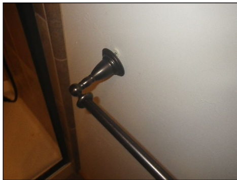
Loose towel rack at bathroom ADU
