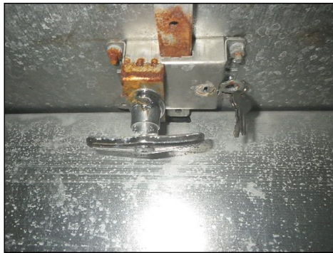
Latch on hatch to terrace is corroded and difficult to operate
