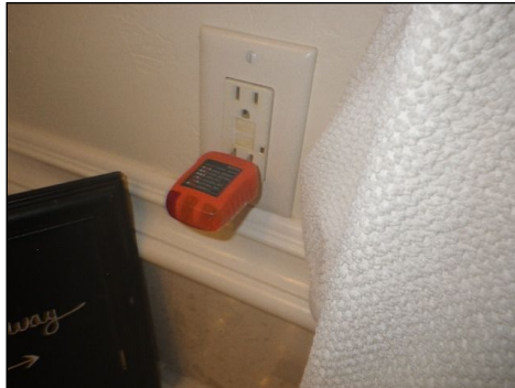
debris stuck in bottom half of left outlet - laundry area
