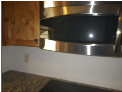
Microwave, disposal and dishwasher on counter GFCI outlets - irregular installation - ADU
