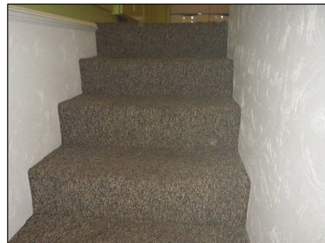
Rise too tall (maximum rise should be 7.75") - unsafe - needs to be serviced - to attic and basement
