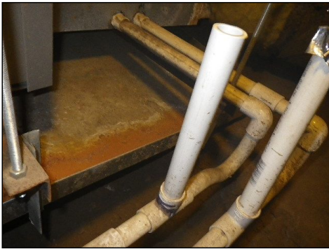
Rust stains/evidence of condensation in catch pan - recommend further evaluation by HVAC contractor - sub floor
