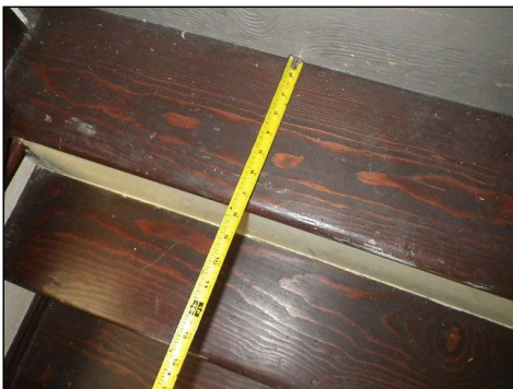
Stair run is less than 10" - needs to be serviced - to attic
