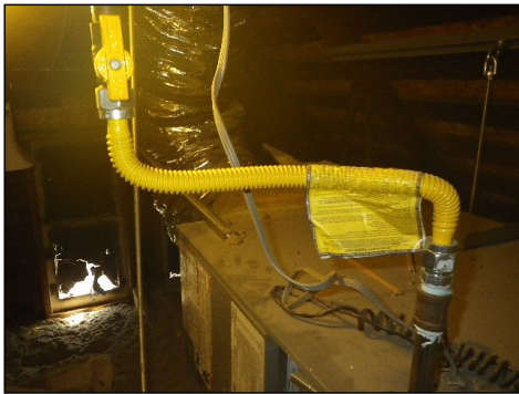
No sediment trap at gas supply - required since the early 2000s
