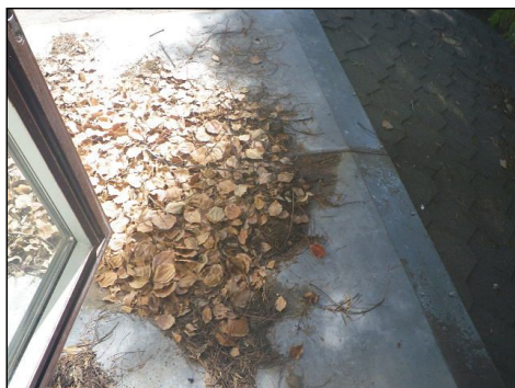
Debris present in areas - recommend cleaning roof area of all debris
