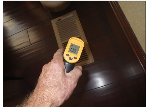
Heater Temperature at Registers: 115 degrees upstairs, 130 degrees downstairs
