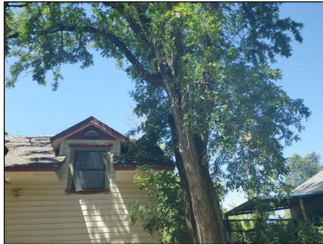
Tree branches hanging over roof - needs to be serviced
