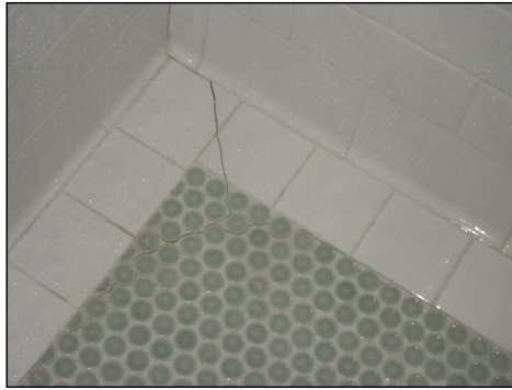
Cracked at pan - needs to be serviced/repaired - master
