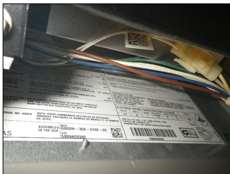
Newer unit/not original to the structure (2009) - check all installation permits to ensure that this unit was installed to proper code
