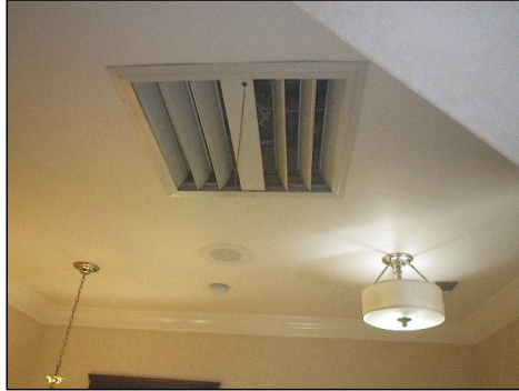
Whole house fan operated
