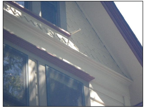
Secondary drain line present
