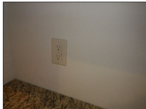
Not operating properly/trips counter outlet GFCI - needs to be serviced - ADU
