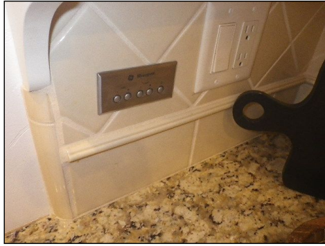
Does not operate - needs to be serviced
