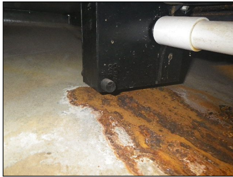
Rust stains/evidence of condensation in catch pan - recommend further evaluation by HVAC contractor - sub floor
