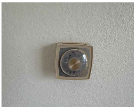
Thermostat: Location Dining Area
