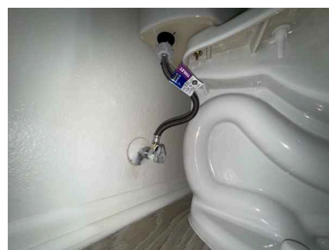
Toilet: Angle Stops
