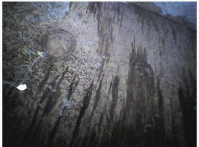
Some signs of water intrusion
