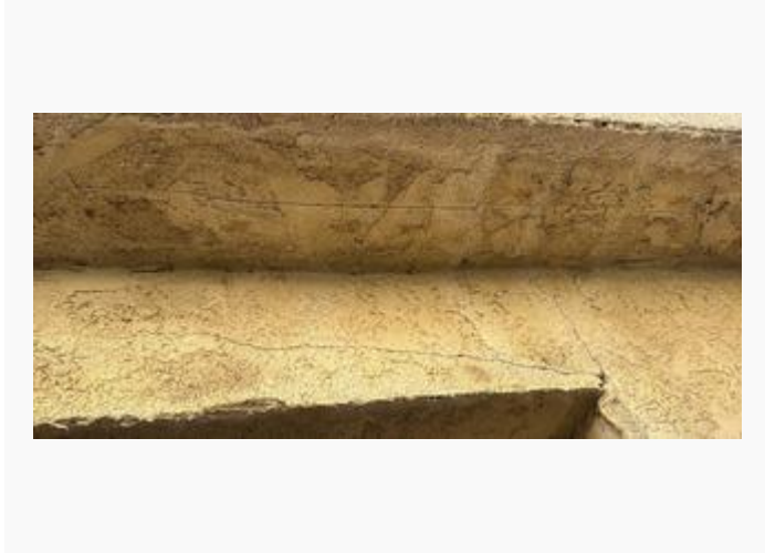
Minor cracking on under side of Balcony
