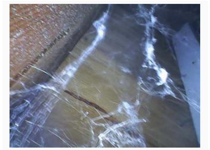
Interior shows no signs of water intrusion and loadbearing elements are good
