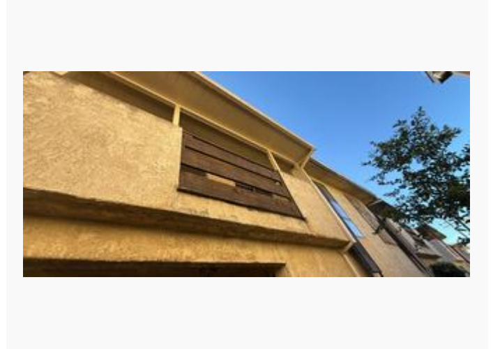
Exterior view shows minor, cracking, in Stucco
