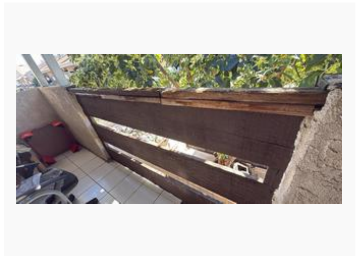
Wall stable and secure, but top railing needs to be replaced is worn and potentially hazardous
