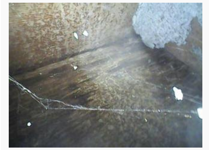
Minor signs of water intrusion, but no significant loadbearing damage
