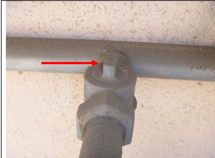
Main gas valve.
