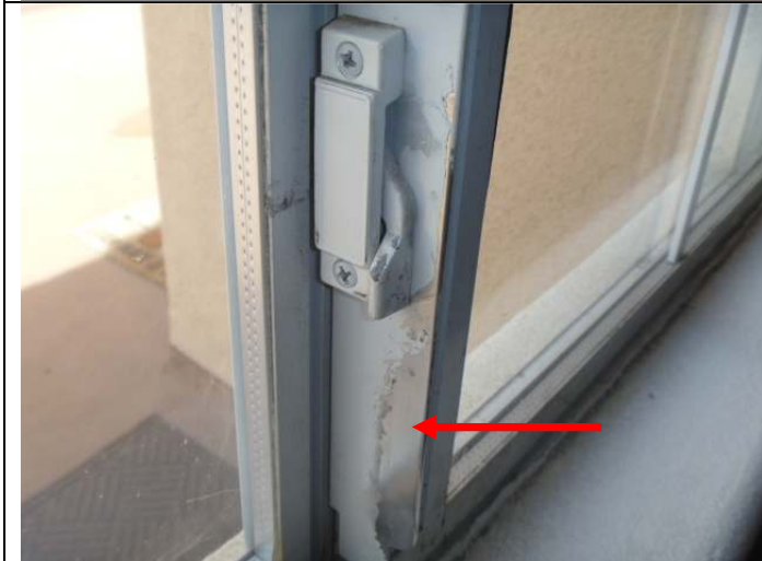
Dining room window surface wear.
