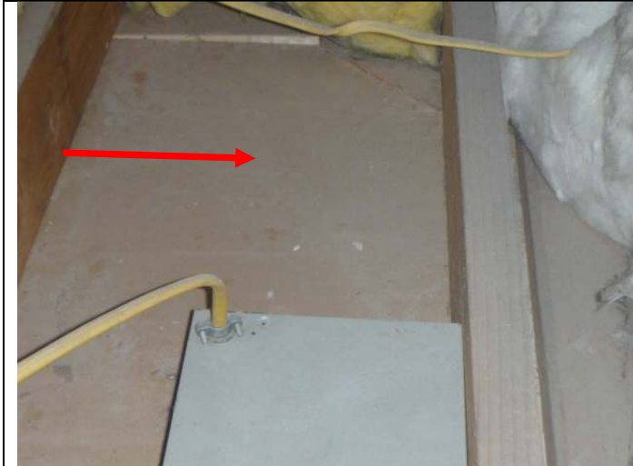
Area of missing attic insulation.
