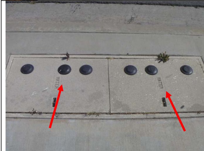
Water meters location along the sidewalk.
