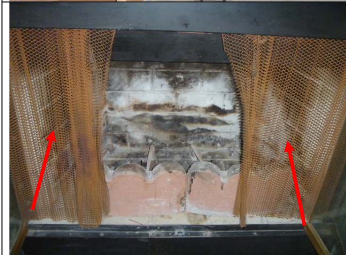
Fireplace. Note: The rusted screens.
