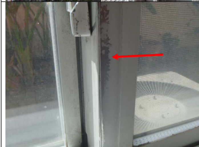
Downstairs bedroom window surface damage.
