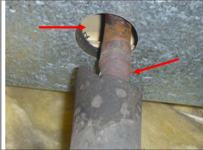
Gap in the air conditioner coil housing at the refrigerant suction line. Note: The missing section of refrigerant line insulation.
