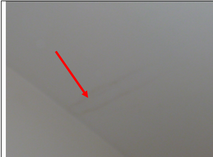
Moisture related discoloration in the living room ceiling at the west wall.
