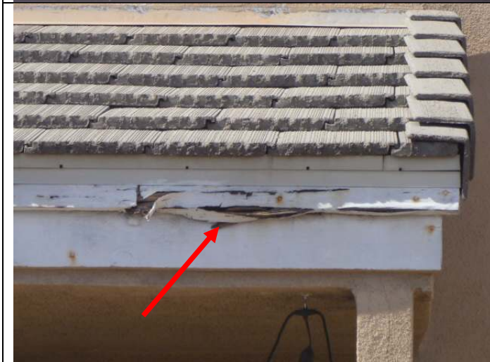
Example of damaged wood.
