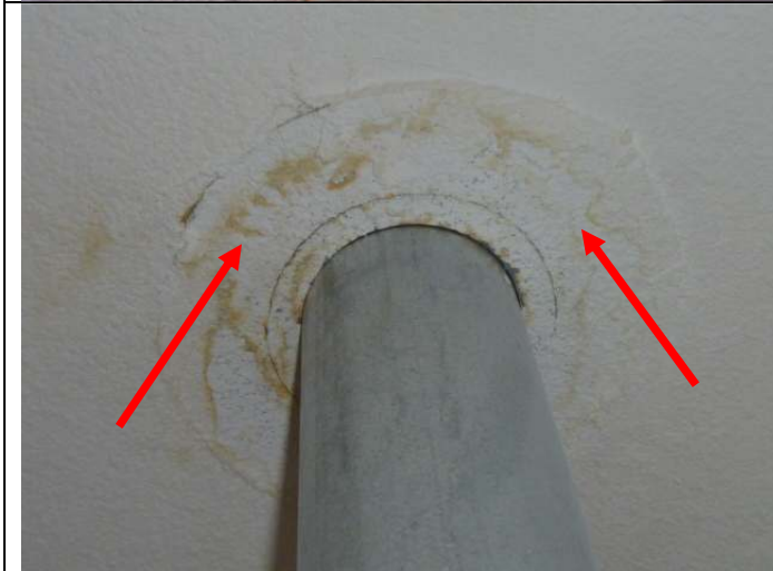
Moisture related discoloration in the laundry room ceiling at the water heater vent pipe.
