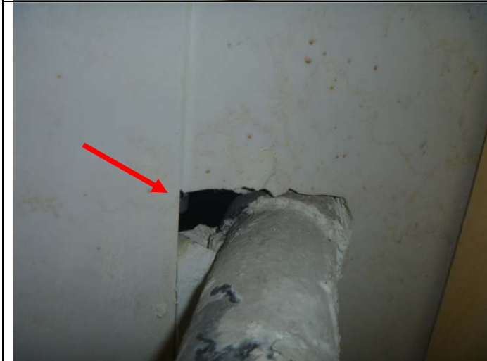
Gap in the wall at the drain pipe below the downstairs 3/4 bathroom sink.
