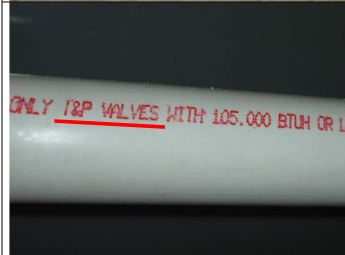
Pressure relief valve PVC drain pipe (with temperature and pressure relief valve rating).
