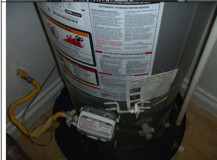
Water heater lower section.
