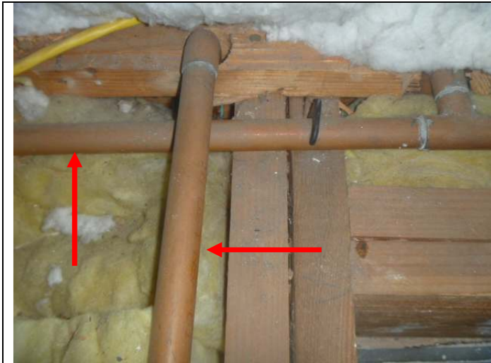
Copper water piping routed through the attic.
