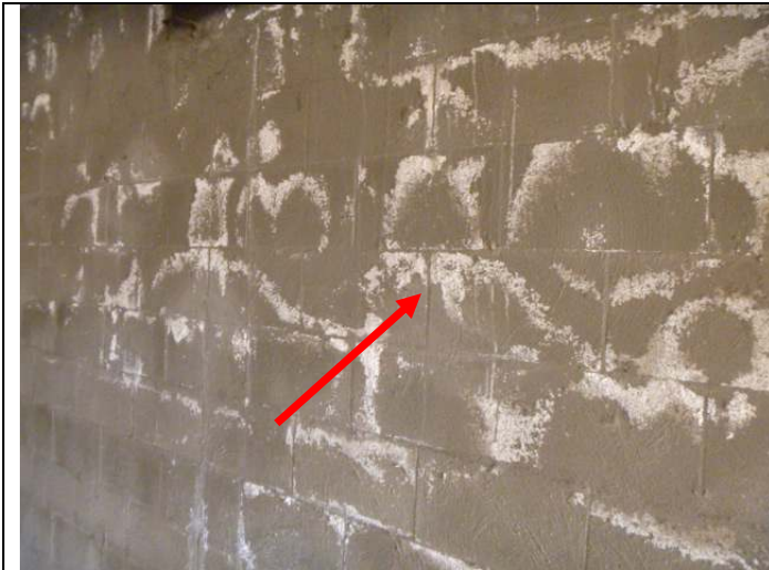
Moisture related efflorescence of the garage east wall.
