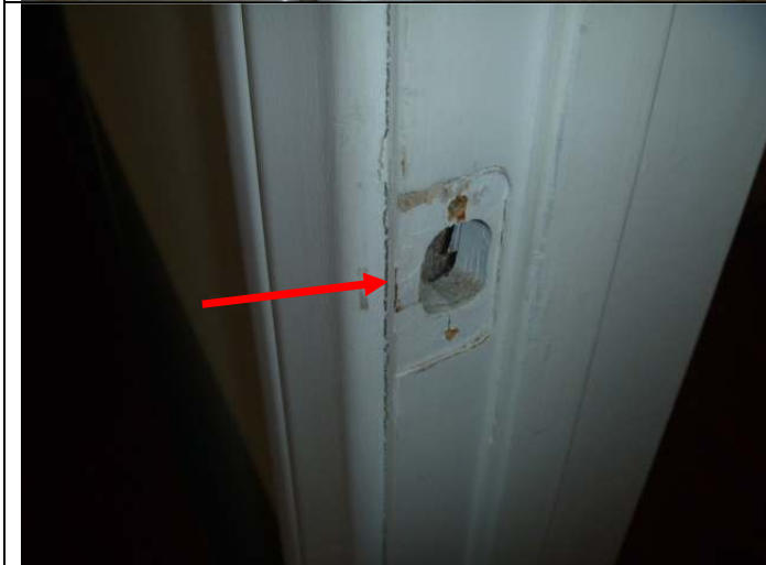
Missing strike plate for the west bedroom entry door.
