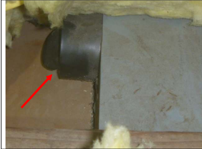
Full bathroom vent fan venting into the attic.
