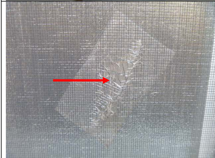
Kitchen torn window screen with transparent tape.
