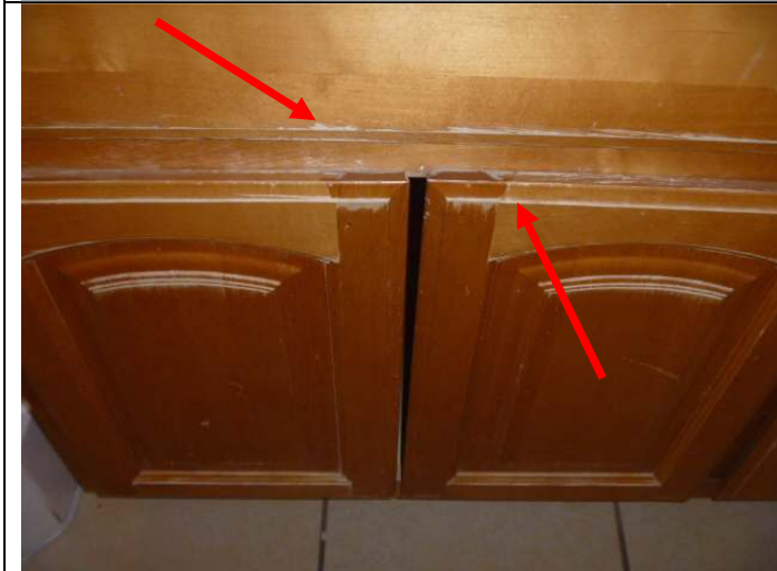
Upstairs 3/4 bathroom sink cabinet wear.
