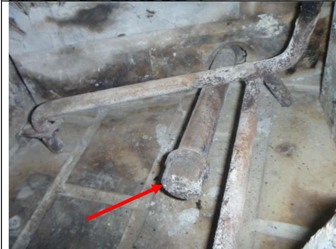
Capped gas pipe in the fireplace.
