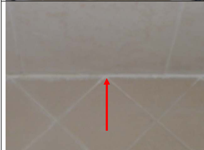
Sealant along the base of the upstairs 3/4 bathroom wall.
