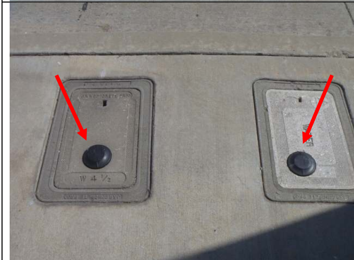
Water meters location along the sidewalk.
