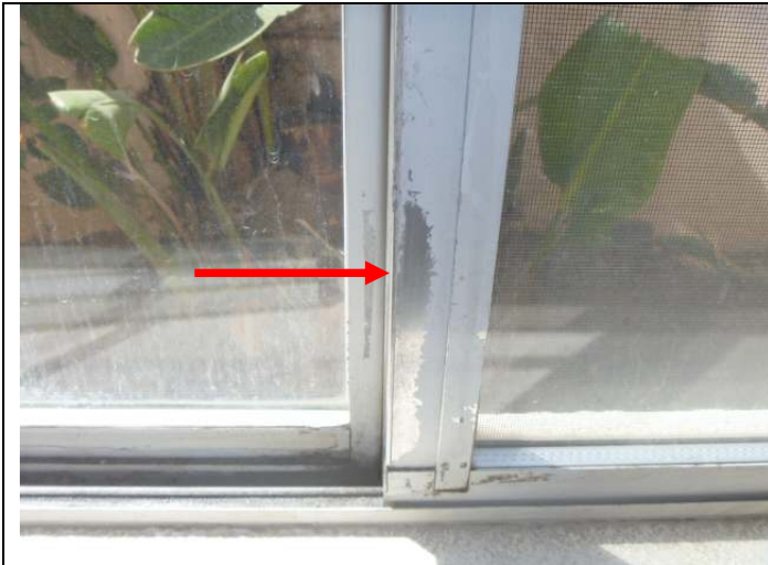
Kitchen window surface damage.
