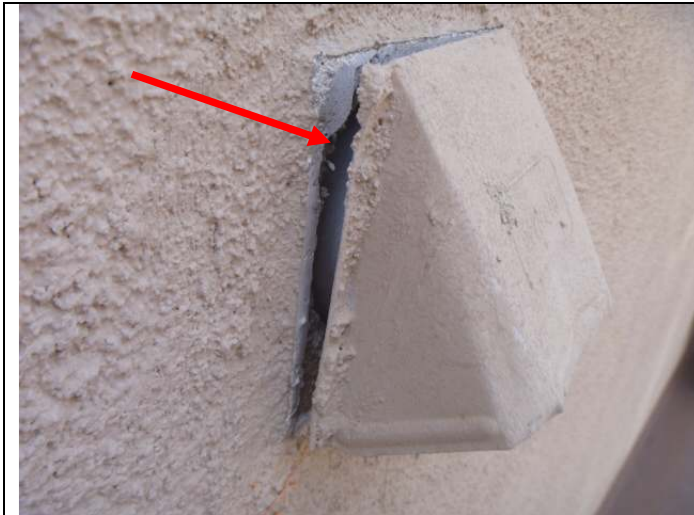
Dryer vent exterior cover not flush with the wall.
