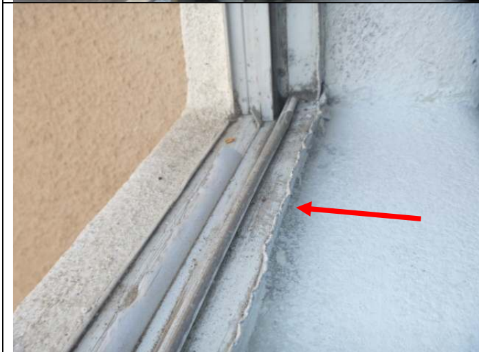
Dining room window bent lower track.
