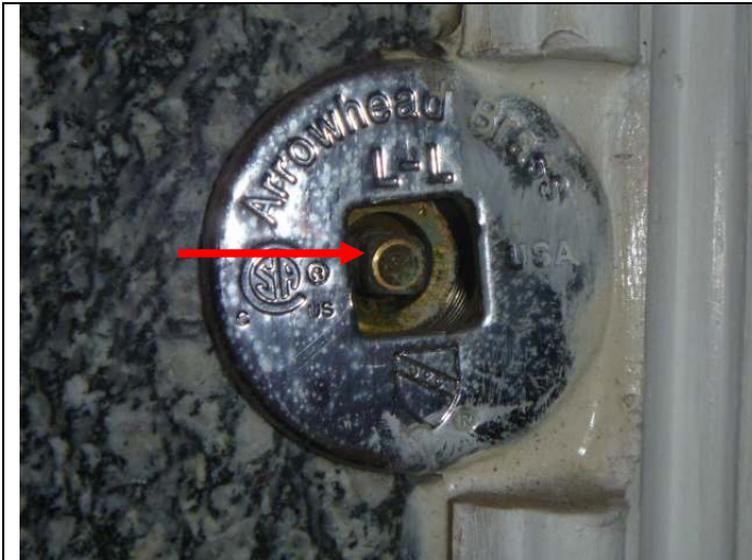
Fireplace gas valve.
