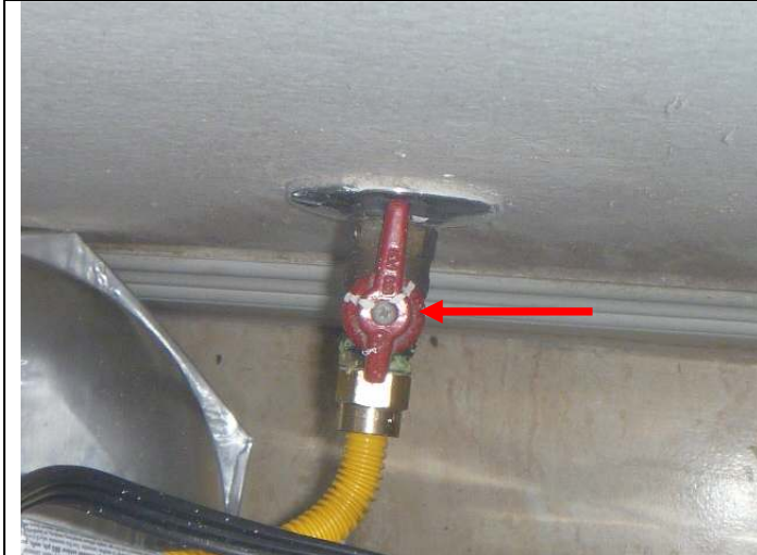
Dryer gas valve.
