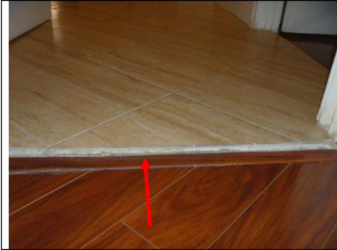
Step along the downstairs bedroom entry doorway.
