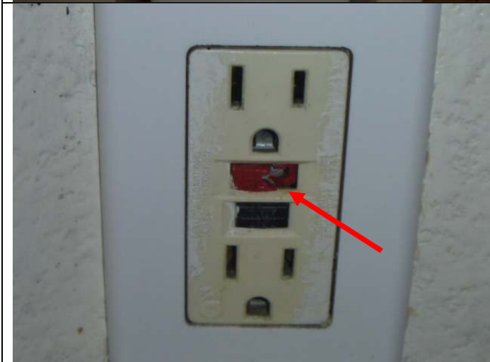
Damaged ground fault circuit interrupter (GFCI) receptacle to the right of the sink.
