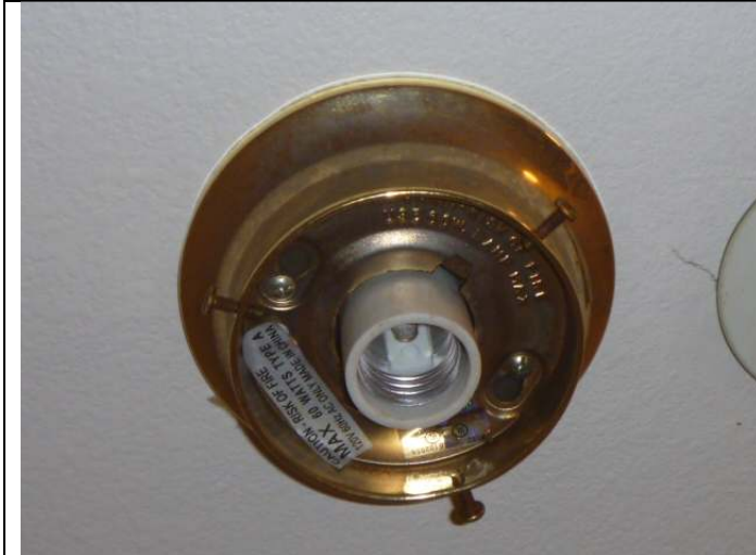
Upstairs 3/4 bathroom ceiling light fixture with missing cover.
