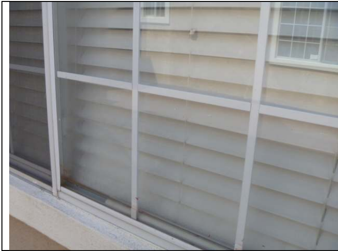
Office fogged window pane.
