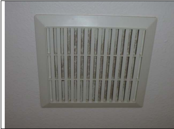
Full bathroom vent fan (which is relatively noisy).
