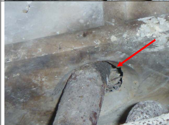
Gap in the fireplace side wall at the gas pipe.
