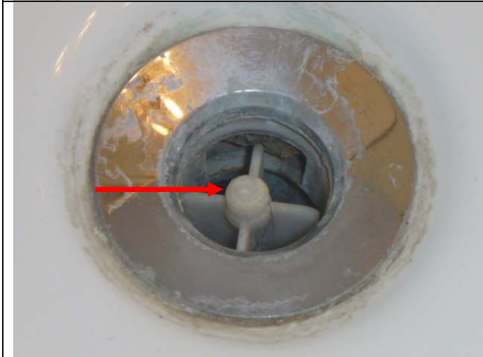
Full bathroom sink stopper with missing top piece.
