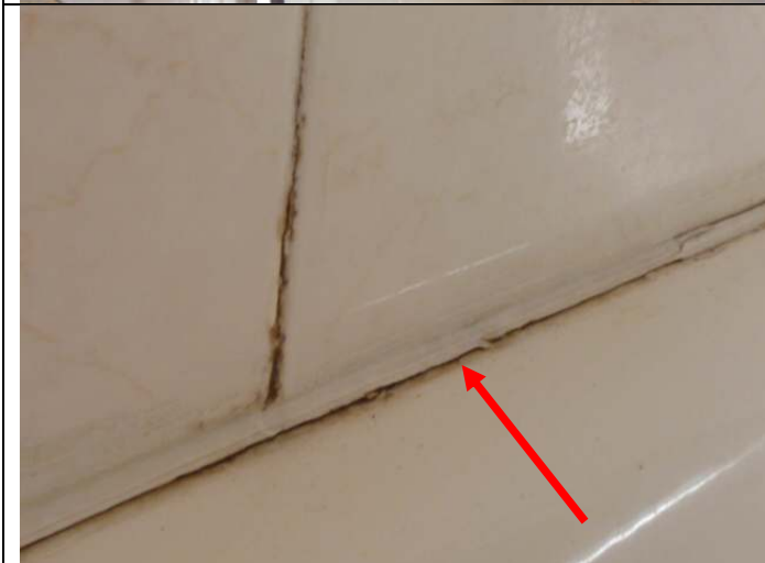
Cracked sealant along the perimeter of the tub.
