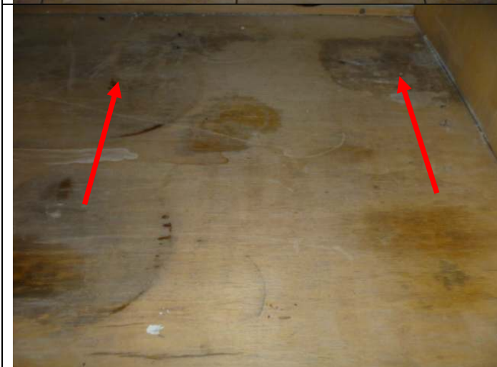
Discoloration in the kitchen cabinet below the sink.
