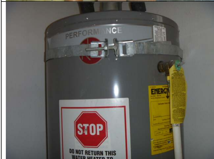
Water heater upper section.
