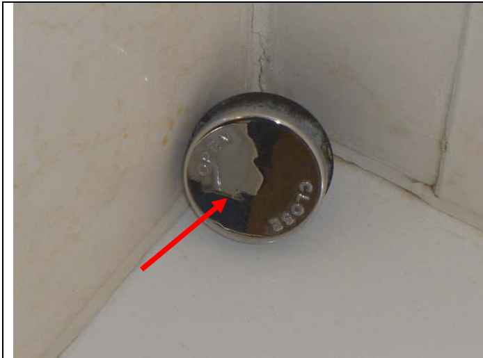
Tub stopper (screw-in type) not installed.
