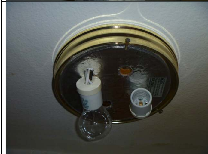
Downstairs bathroom light fixture with missing cover.
