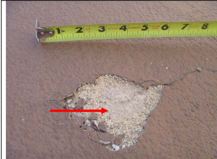
Courtyard surface damage.
