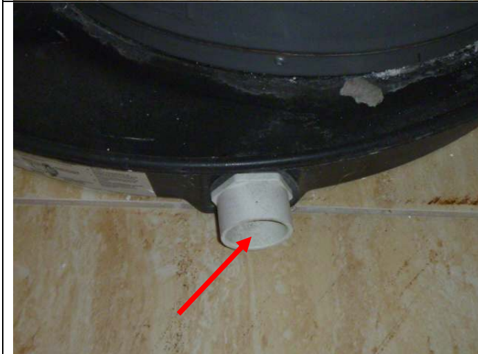
Water heater catch pan without a drain pipe.
