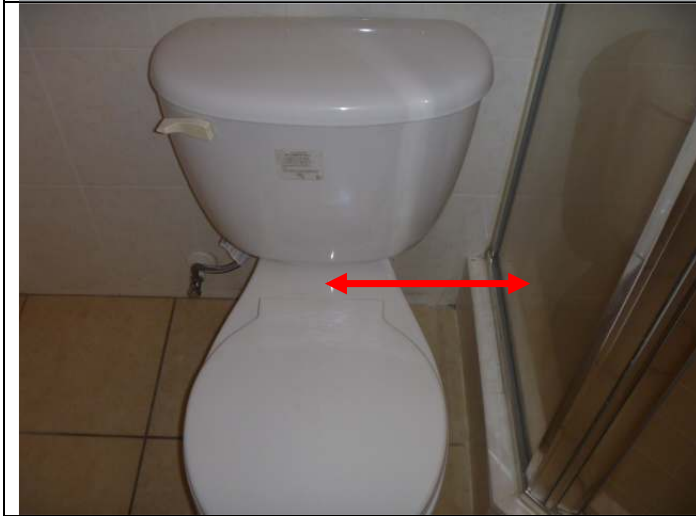
Upstairs 3/4 bathroom toilet relatively close to the shower enclosure.
