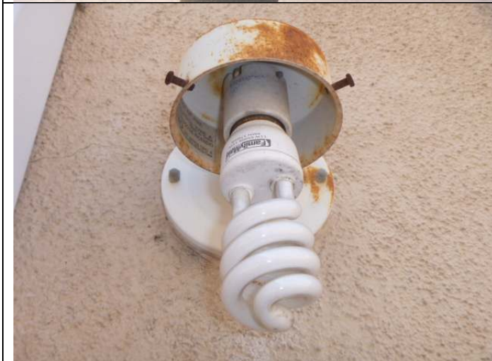
Missing light exterior light fixture to the right of the living room exterior door.
