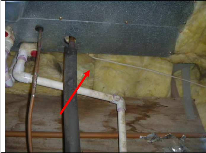
Air conditioner coil without a catch pan.
