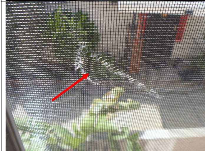
West bedroom torn window screen.
