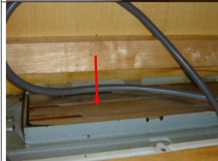
Microwave vent fan venting into the above cabinet.
