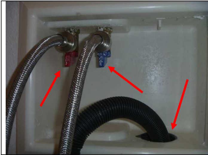
Washer hookups and drain.
