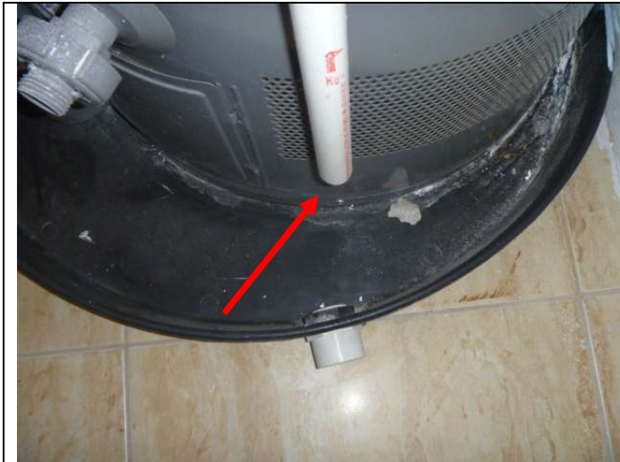
Water heater pressure relief valve drain pipe draining into the catch pan.
