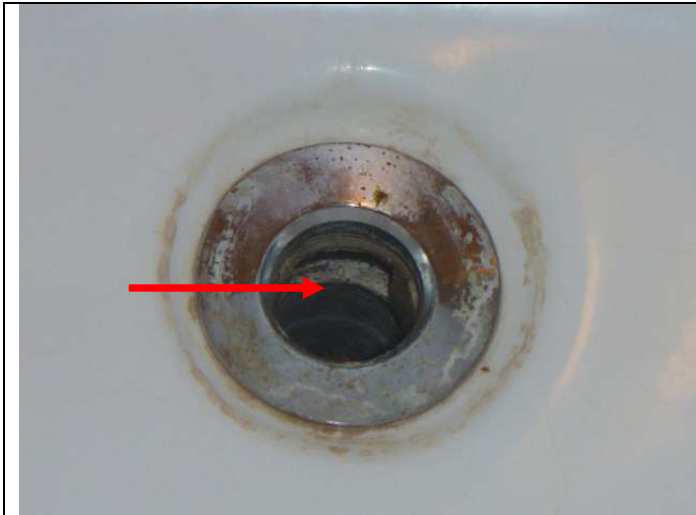
Upstairs 3/4 bathroom missing sink stopper.
