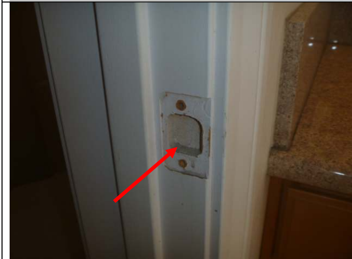
Missing strike plate for the door leading to the full bathroom toilet area.
