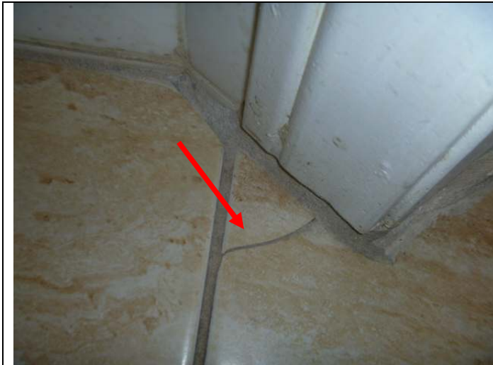
Cracked floor tile to the left of the downstairs 3/4 bathroom entry door.
