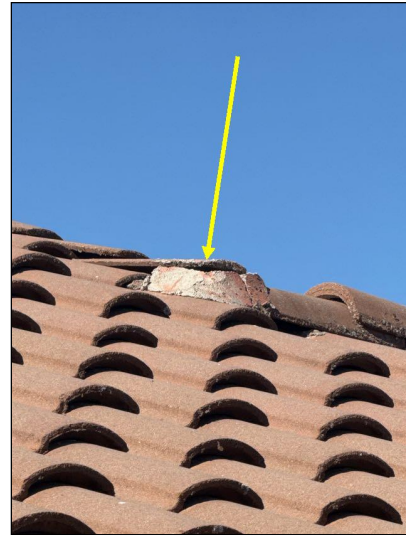
Roof ridge cap tiles are mastic sealed at intersections, the mastic is cracked
