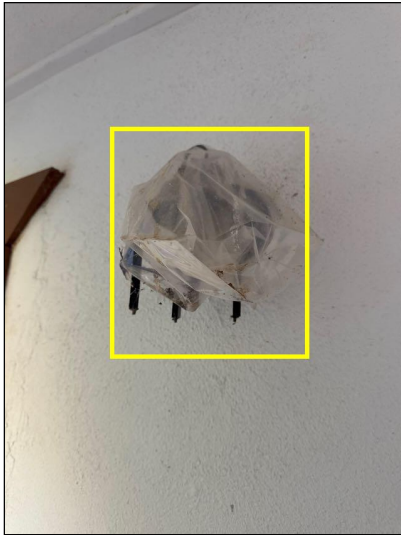
Several exterior light fixture were damaged
