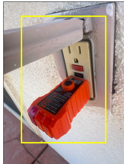
GFCI electrical receptacle was inoperable at the time of the inspection. (left side of the home)
