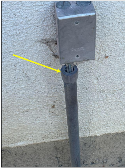
The electrical conduit is separated and/or damaged. (north garage area)
