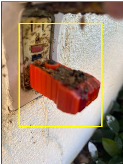
GFCI electrical receptacle was inoperable at the time of the inspection. (courtyard)
