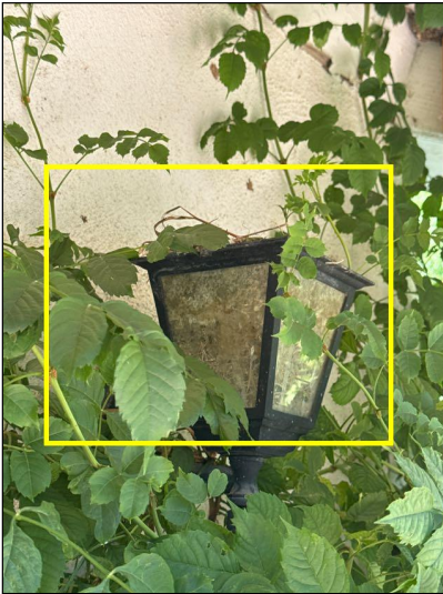
Several exterior light fixture were damaged
