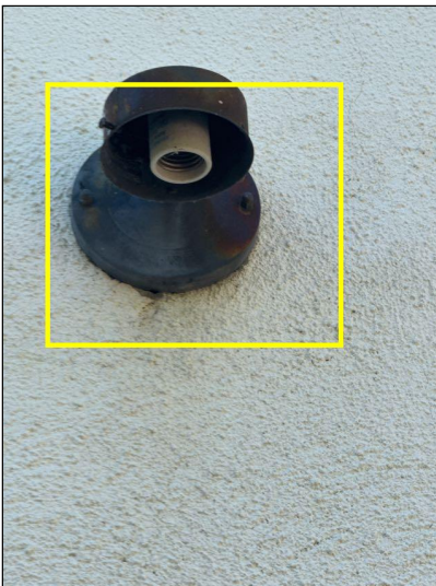
Several exterior light fixture were damaged
