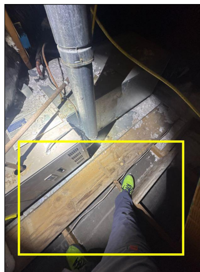
The furnace maintenance platform was of inadequate size for good service access.
