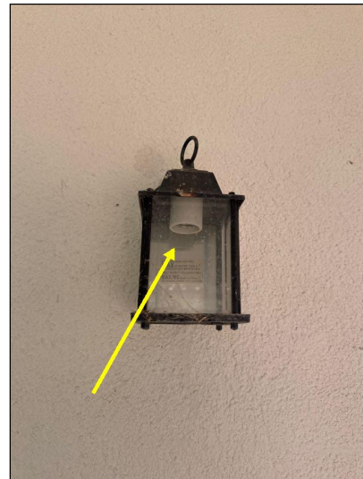
Several exterior light fixture were missing light bulbs at the time of the inspection.
