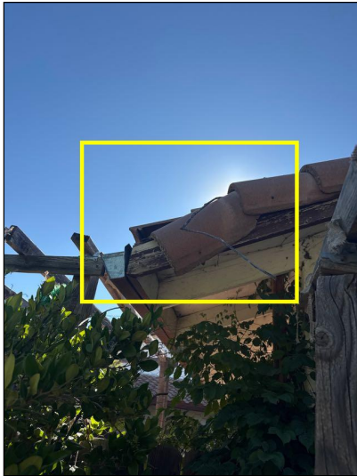
Tiles along the rakes (sloped roof edges) were loose and fasteners were visibly protruding.
