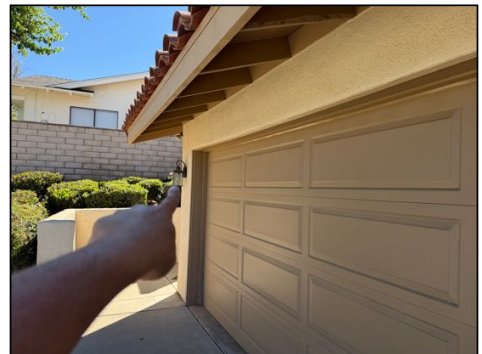
Some light(s) did not function (some may be on sensors or timers) - check bulbs first, then consult an electrician to further evaluate as needed
