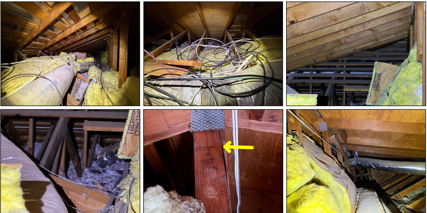
Cracked wood - typical for age
