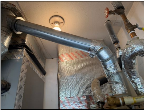
Recommend sealing all connections at venting
