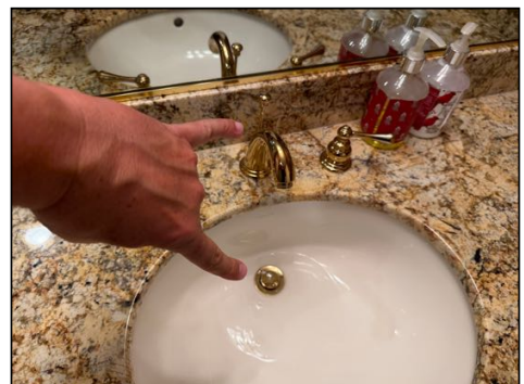
Drain stopper not operating properly - needs to be serviced - hall bathroom, left sink and bathroom near kitchen
