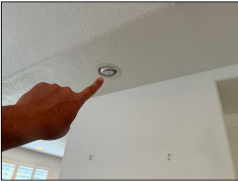
Some bulbs defective/missing/light(s) did not function - check bulbs/consult electrician to further evaluate
