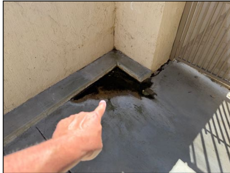
Standing/ponding water in areas – signs of poor drainage
