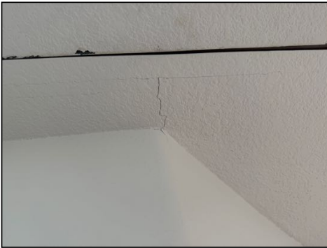
Small cracks/holes/chipped/dirty areas/cosmetic blemishes observed - typical for age of structure
