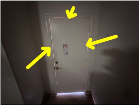
Visible daylight is present around the exterior door - recommend proper weatherstrip seal and/or maintenance
