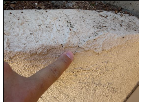
Cracking/chipping small and typical for age at block - monitor for further cracking and repair as needed
