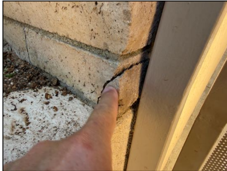
Cracking/chipping small and typical for age at block - monitor for further cracking and repair as needed
