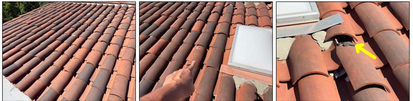
Loose/slipping tiles/shingles - recommend servicing
