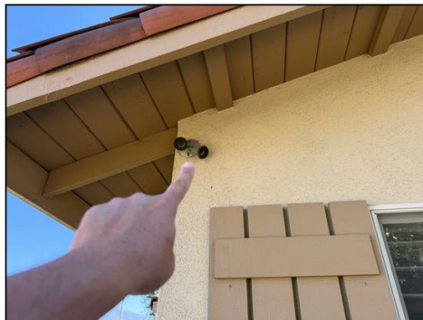
Some light(s) did not function (some may be on sensors or timers) - check bulbs first, then consult an electrician to further evaluate as needed
