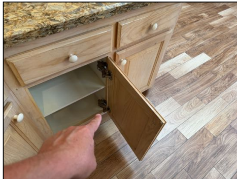
Worn cabinets with loose/worn hardware - typical for age
