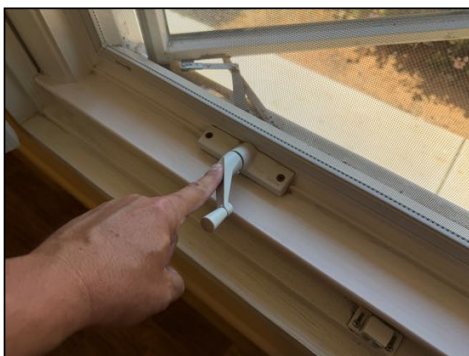
All crank windows are difficult to close – service needed
