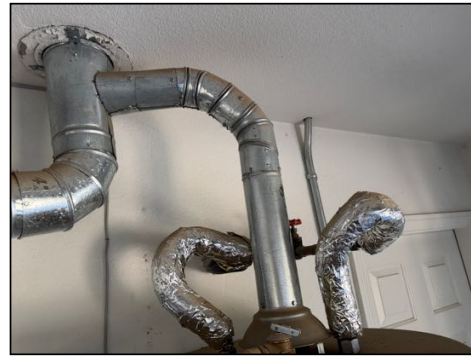
Recommend sealing all connections at venting
