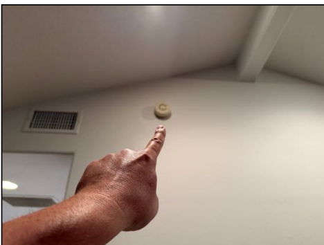
All smoke detectors are visibly too old – not tested – replacement needed
