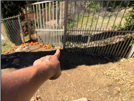
Metal fence, buried beneath soil in some locations stash recommend service in an effort to prolong life
