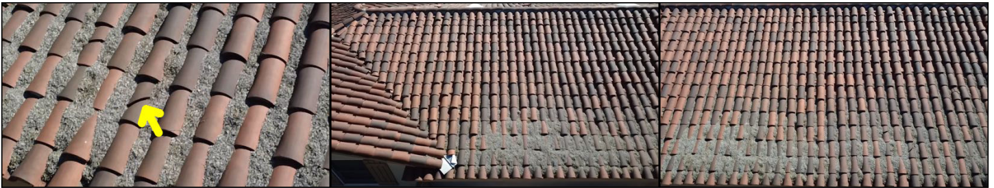
Broken tiles - needs to be serviced
