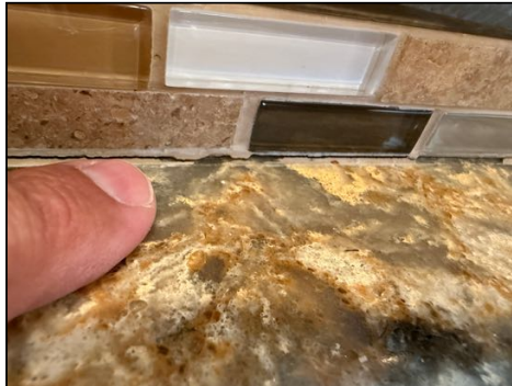
Cracked/loose/missing grout in areas – service needed
