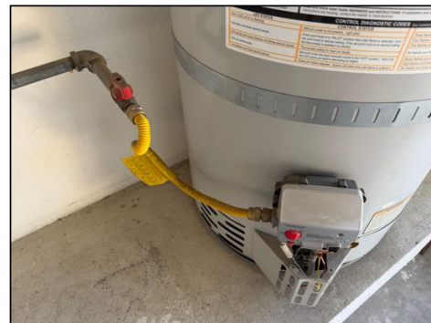
No sediment trap at gas supply - may have not been required at time of original installation, but is recommended
