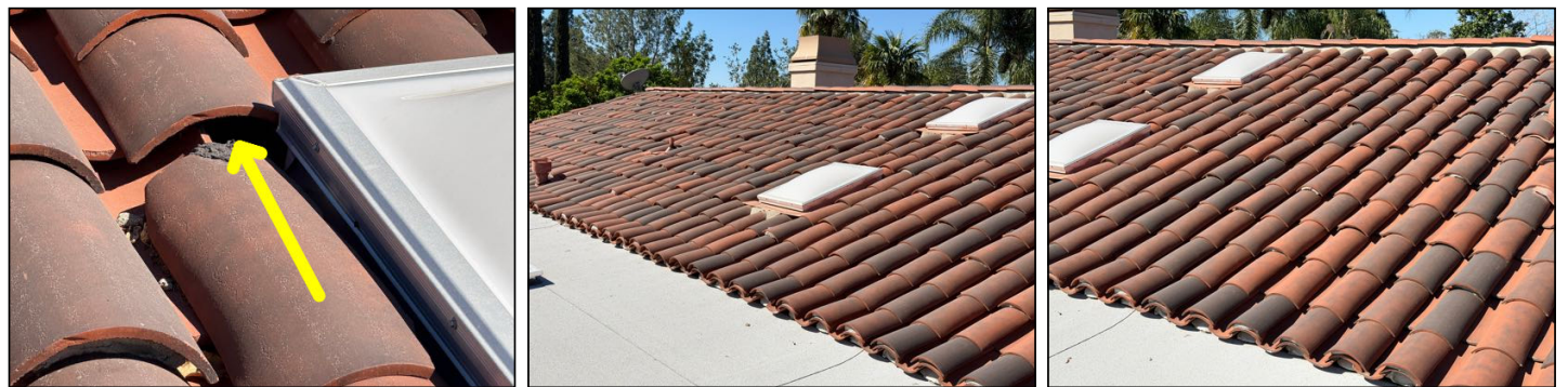
Loose/slipping tiles/shingles - recommend servicing
