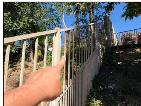
Rust/rust damage at metal fence materials - needs to be serviced
