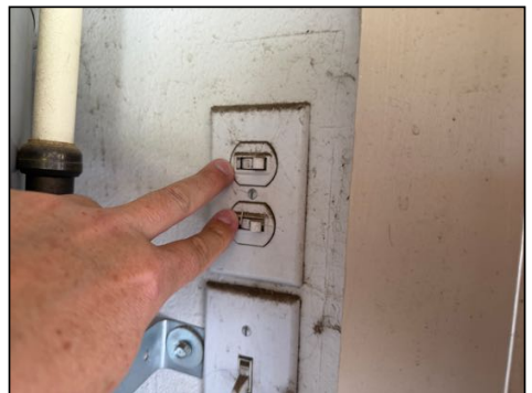
Some switches have unknown function - not inspected - inquire with seller regarding operation
