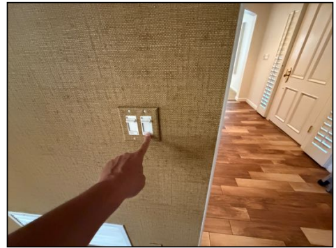
Some switches have unknown function - not inspected, inquire with seller regarding operation
