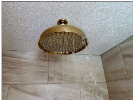
Showerhead not spraying properly – master and hall bathroom – service needed
