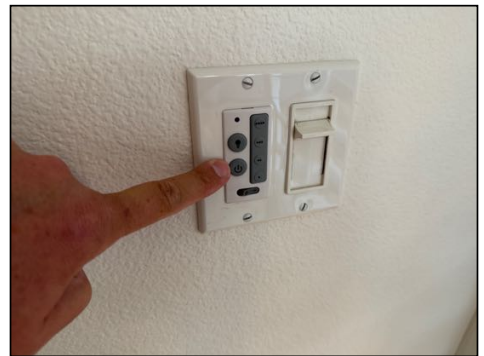
Did not operate - needs to be serviced or further evaluated - kitchen area
