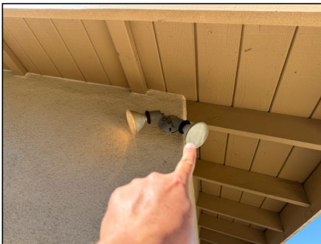
Some light(s) did not function (some may be on sensors or timers) - check bulbs first, then consult an electrician to further evaluate as needed
