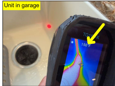
Unit in garage Temperature was above 120 F at one or more fixtures within the structure, this a potential scald hazard - needs to be serviced/adjusted - consult a plumber - both
