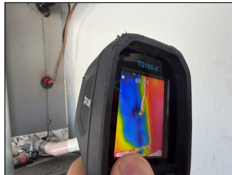
Air leaking at refrigerant or condensate line connection areas - needs to be sealed to prevent air loss - both
