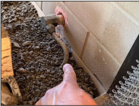
Flex/aluminum gas line in firebox to loglighter without cosmetic logset present - needs to be serviced
