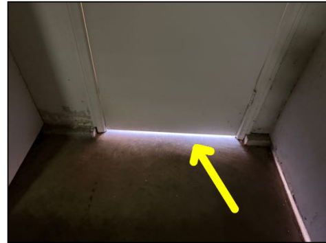
Missing threshold - recommend installing a proper threshold in an effort to prevent weather/pest intrusion
