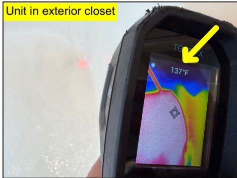
Unit in exterior closet Temperature was above 120 F at one or more fixtures within the structure, this a potential scald hazard - needs to be serviced/adjusted - consult a plumber - both
