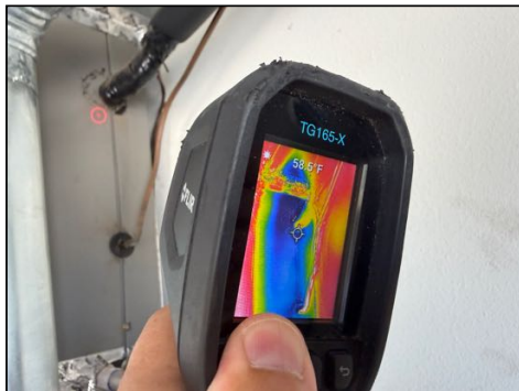
Air leaking at refrigerant or condensate line connection areas - needs to be sealed to prevent air loss - both
