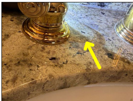
Hot fixture handle leaks above countertop when operated – master bathroom, right sink
