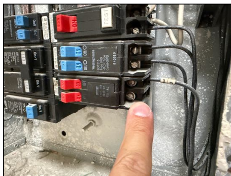
Unused breaker present – consult seller
