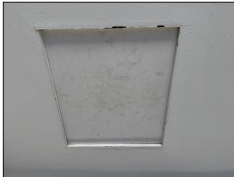
Access door is dirty with cosmetic blemishes present
