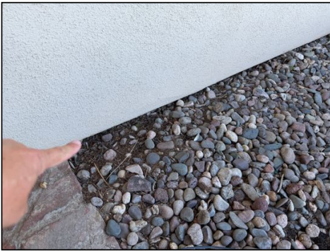
Weep screeds should be minimum 4-inches from grade - needs to be serviced
