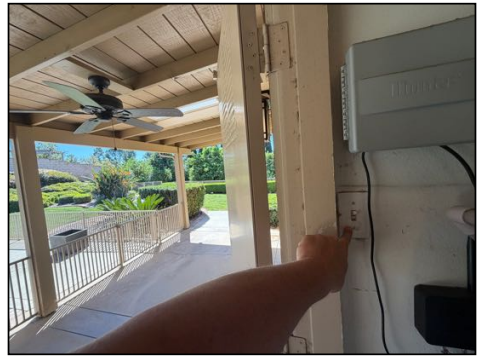
Ceiling fans operated properly at the time of inspection – switch located inside heater/water heater closet at exterior of master bedroom suite
