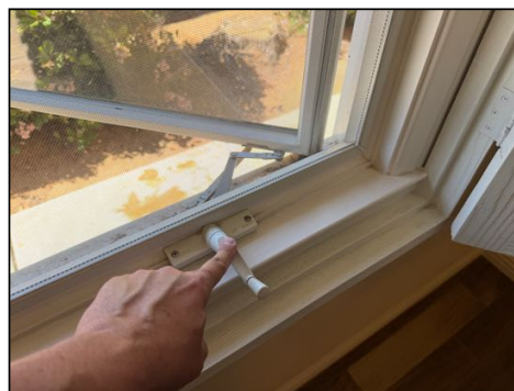
All crank windows are difficult to close – service needed
