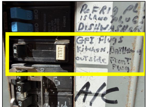
Master control GFCI located in: main electrical panel
