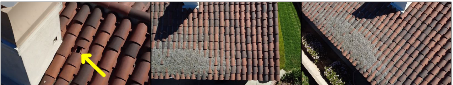
Loose/slipping tiles/shingles - recommend servicing
