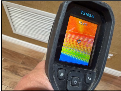
Temperature at Air Return
