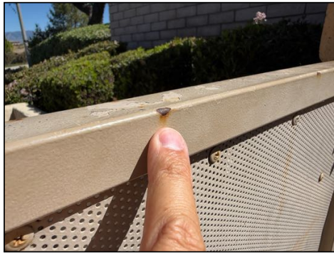
Rust present - recommend rust treatment to prolong material life
