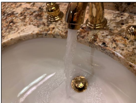
Irregular spray when operated - needs to be serviced - both in hall bathroom
