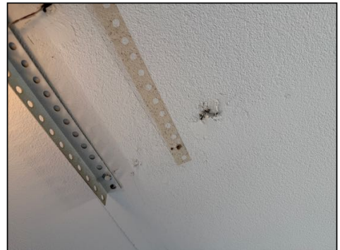
Holes small - recommend patch/paint as needed
