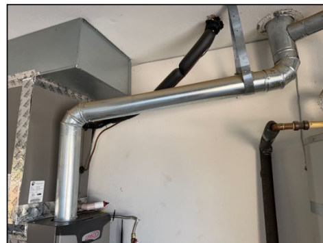
Recommend securing and sealing all vent connections
