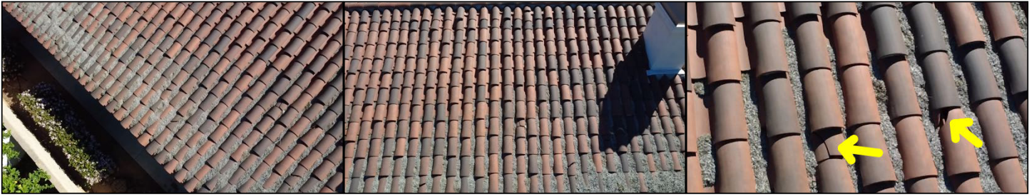
Broken tiles - needs to be serviced
