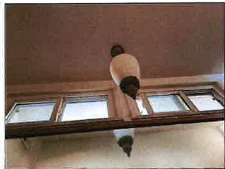
Some bulbs defective/missing/light(s) did not function - check bulbs/consult electrician to further evaluate
