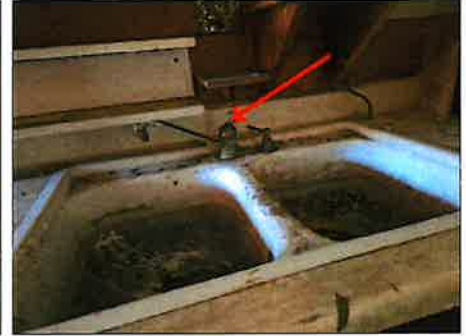
Not operating/ needs servicing
