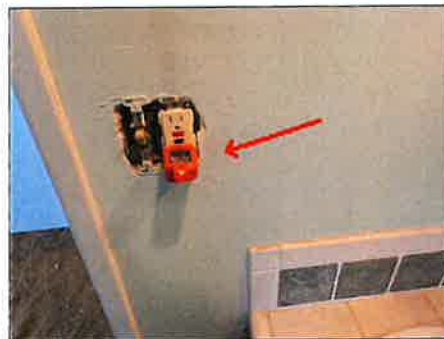
GFCI not grounded - typical for old ungrounded system pre-1965
