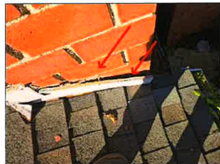
Flashing at base of chimney appears to need some maintenance to ensure a continued waterproof seal
