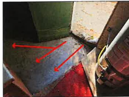
Evidence of moisture intrusion/ needs servicing and further evaluation
