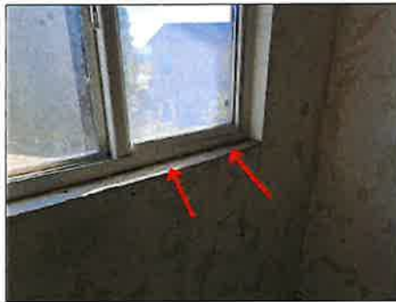
Stains/blisters at sill - tested dry for moisture at the time of the inspection - monitor the areas for moisture intrusion
