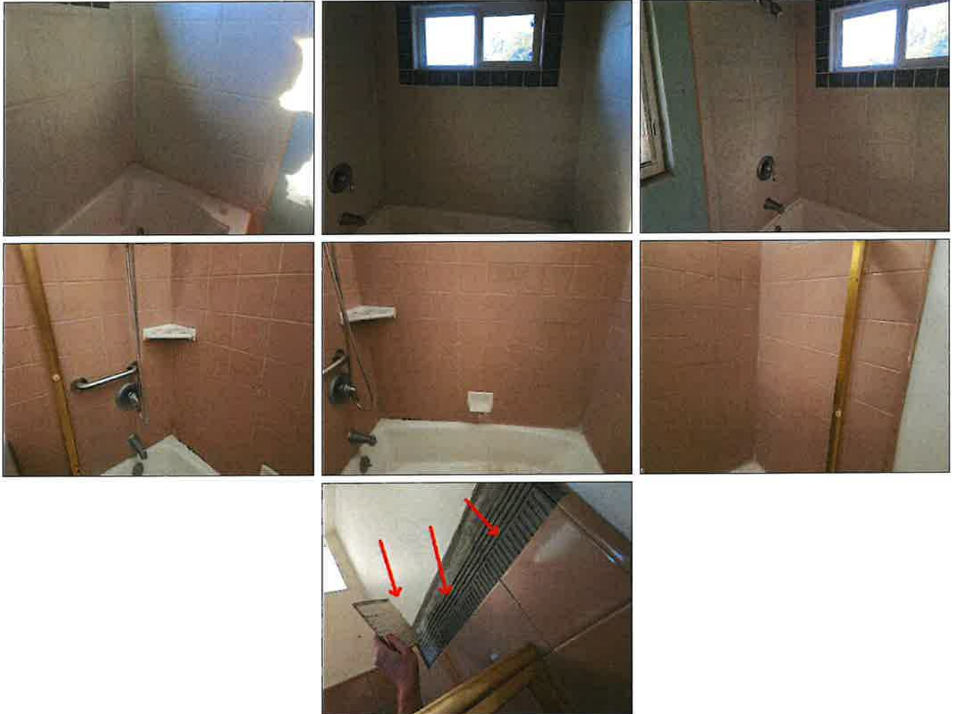
Broken/loose tile(s) - needs to be serviced
