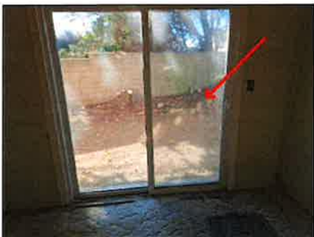
Difficult to slide/operate- needs to be serviced
