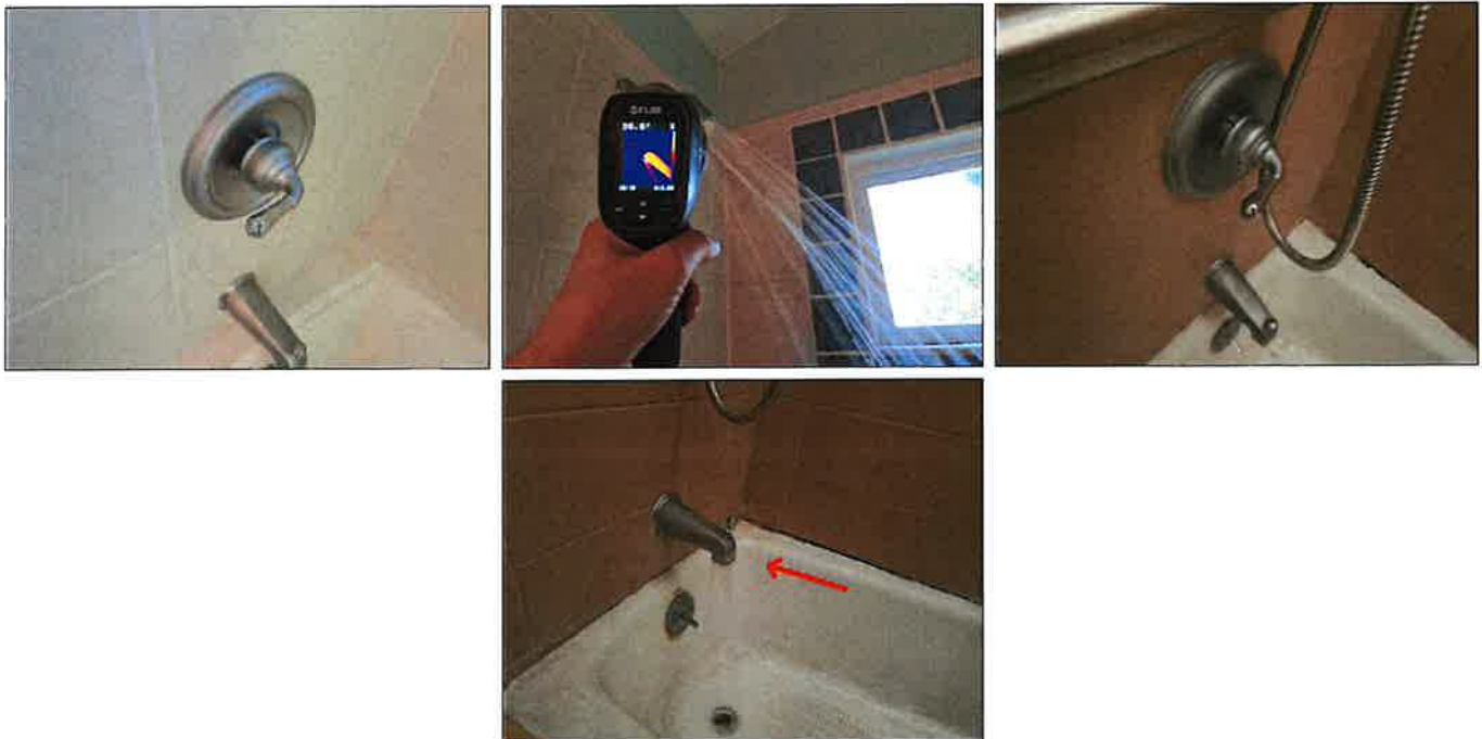
Diverter does not properly divert water to shower head - needs to be serviced
