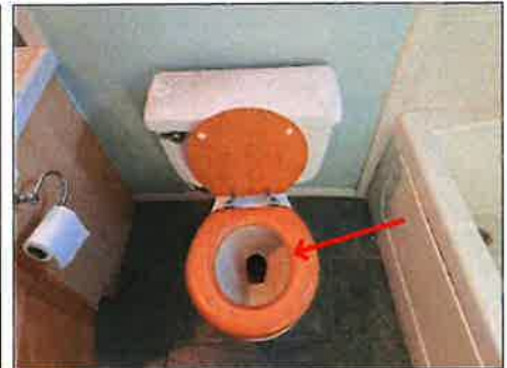
Toilet did not flush - needs to be serviced
