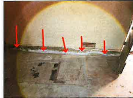
Efflorescence present heavy - needs to be further evaluated
