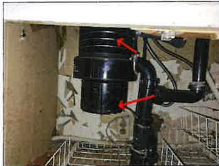
Leaking under sink - needs to be serviced
