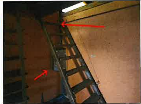
Pull down ladder access is worn/loose/difficult to operate- / irregular counter weight/ recommend maintenance
