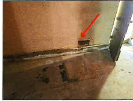
Vents obstructed - drywall/panel covered - needs to be serviced
