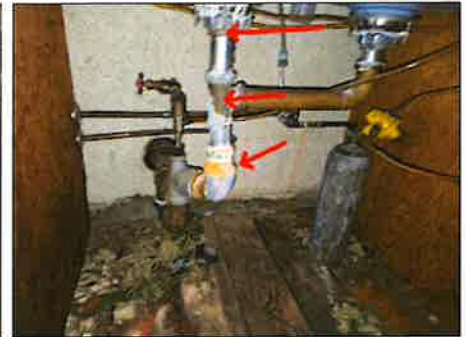
Corroded plumbing - may require repair soon, recommend servicing
