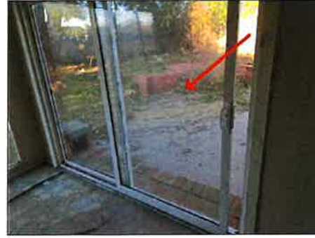
Difficult to slide/operate- needs to be serviced
