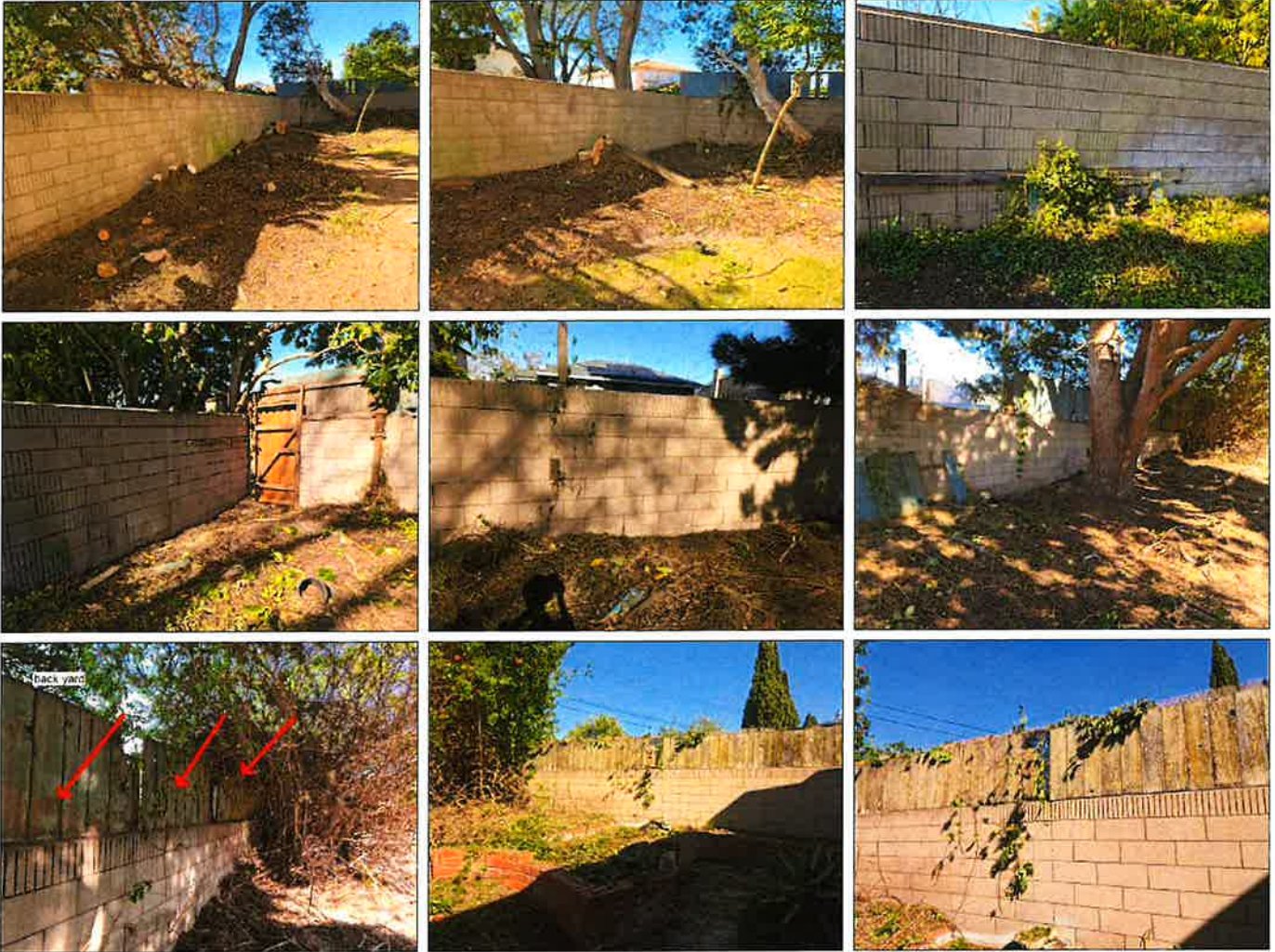
Damaged fencing/walls - needs to be serviced
