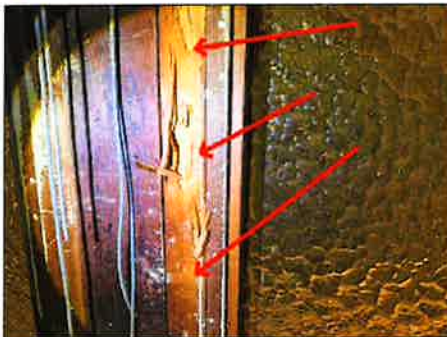
Deteriorated frames - recommend servicing
