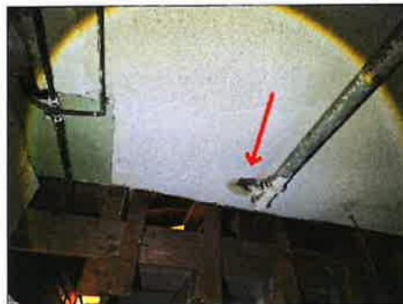
Stains present - tested positive for moisture at time of inspection - recommend further evaluation
