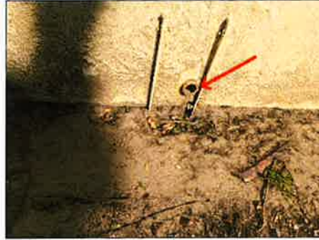
Clean out cap for sewer damaged/missing - recommend servicing
