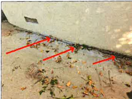
Weep screeds encapsulated in concrete - needs to be serviced
