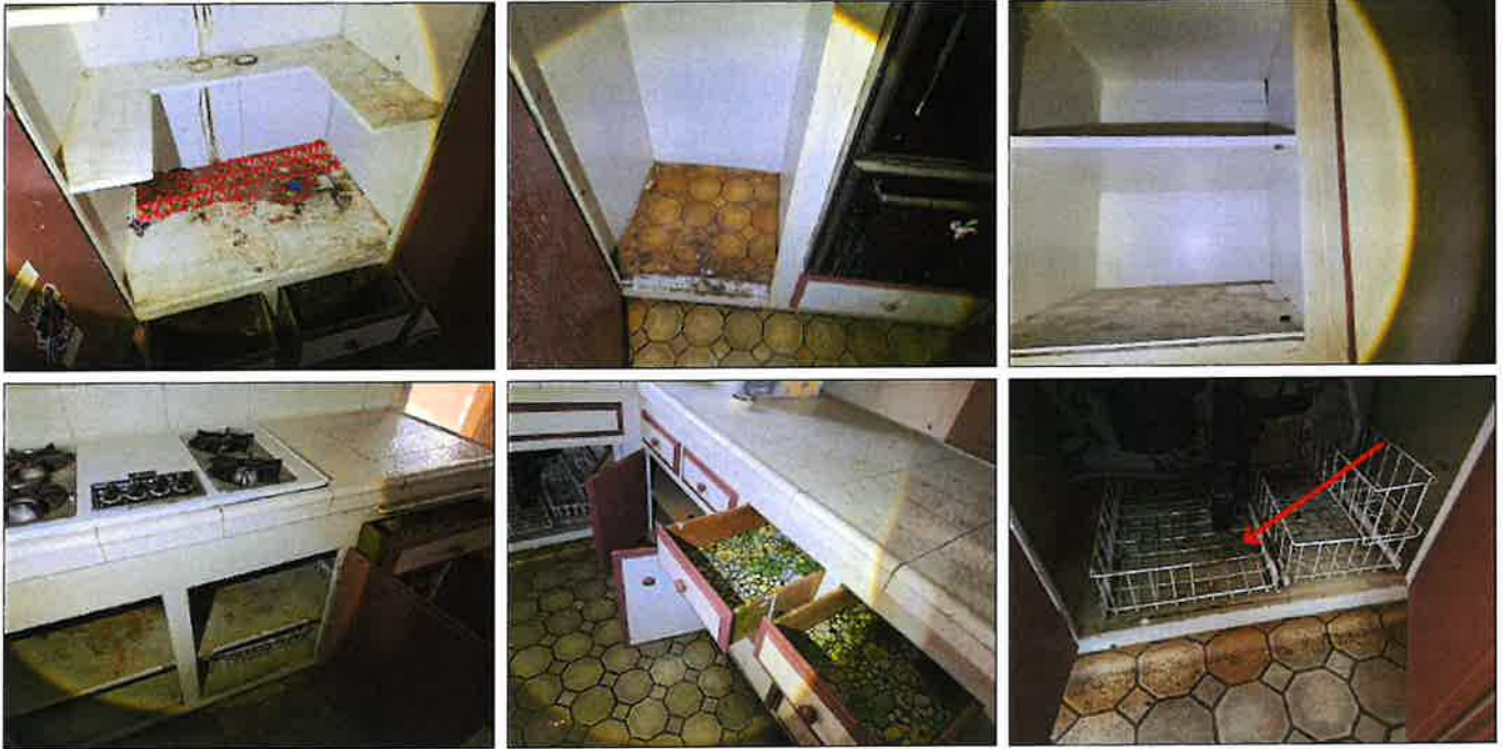
Stained/blistered area(s) - moisture present at time of inspection - needs to be serviced/further evaluated
