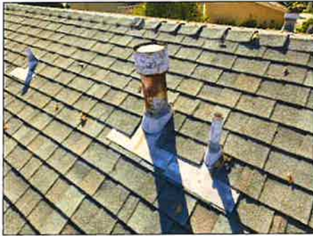
Rusted - needs to be serviced
