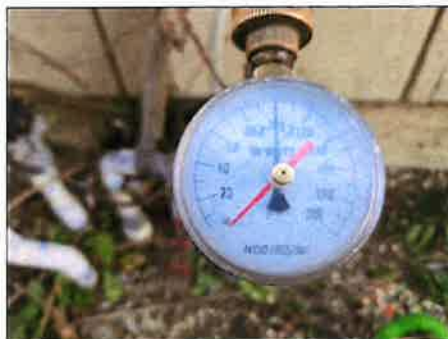
Approximate pounds per square inch: 100 - needs to be serviced
