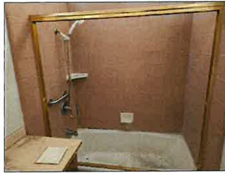
Missing or no door is present
