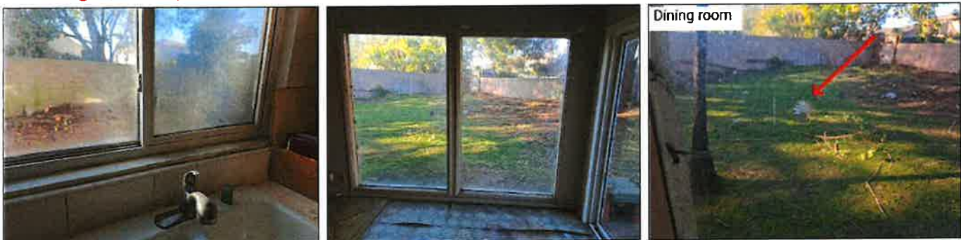
Hole in glass- needs to be serviced
