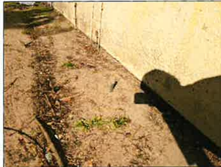
Condensation/moisture damage - needs to be serviced
