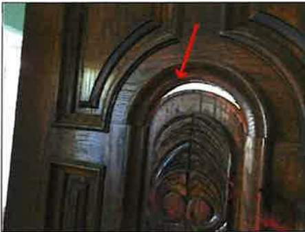
Damaged _ needs to be serviced
