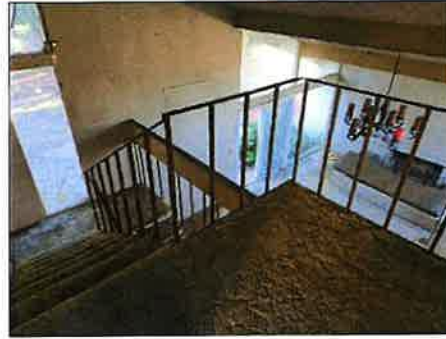
Rail opening too wide- unsafe - needs to be serviced
