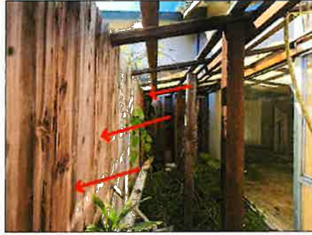
Moisture damage - needs to be serviced - hidden defects may exist
