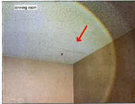
Stains/blistered areas present - tested dry with moisture meter at time of inspection
