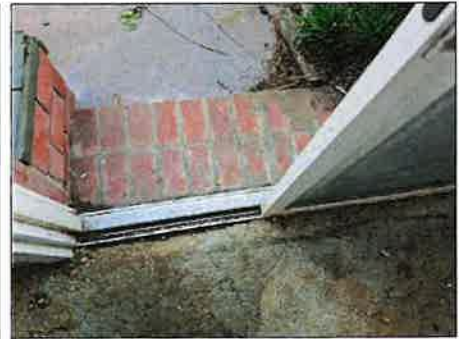
Dirty tracks - needs to be serviced
