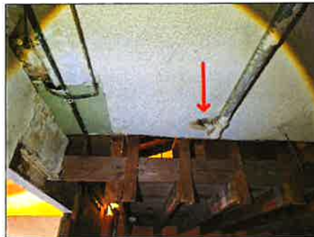
Leaking plumbing - needs to be serviced
