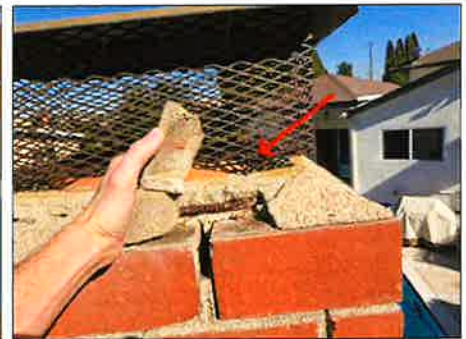
Cement chimney cap deteriorated - needs to be serviced
