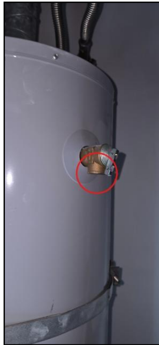
33. Discharge tube missing
