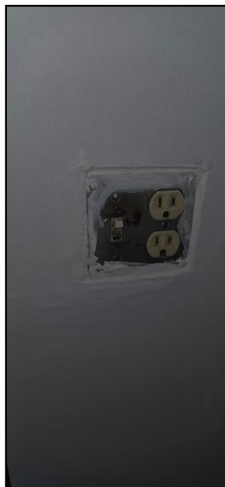
18. GFCI/GFI needed (Ground Fault Circuit...)
