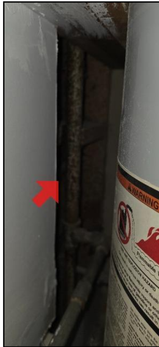
50. Loose or missing
