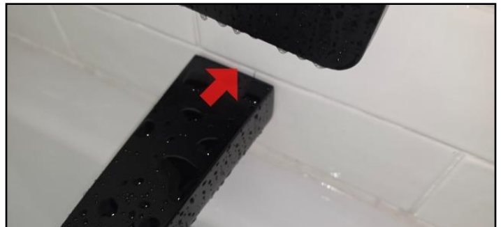
44. Caulking loose, missing or deteriorated
