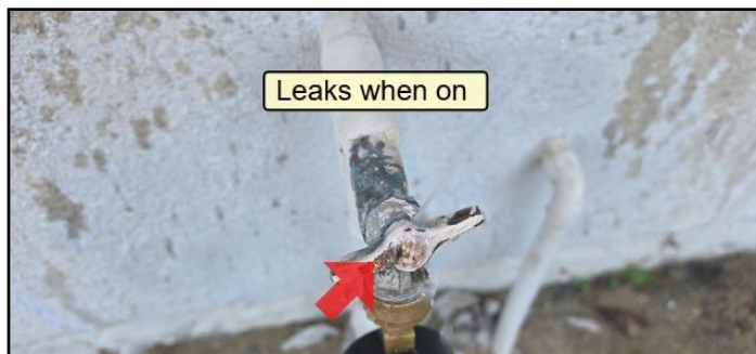
38. Leak or drip
