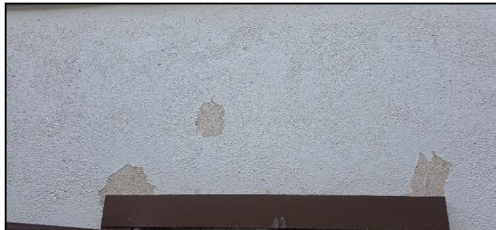
12. Paint or stain - needed
