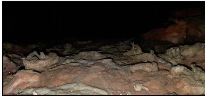
25. Amount less than current standards
