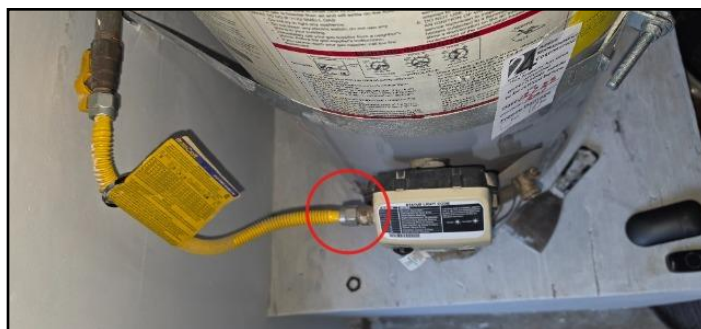
34. No drip leg (sediment trap/dirt pocket)
