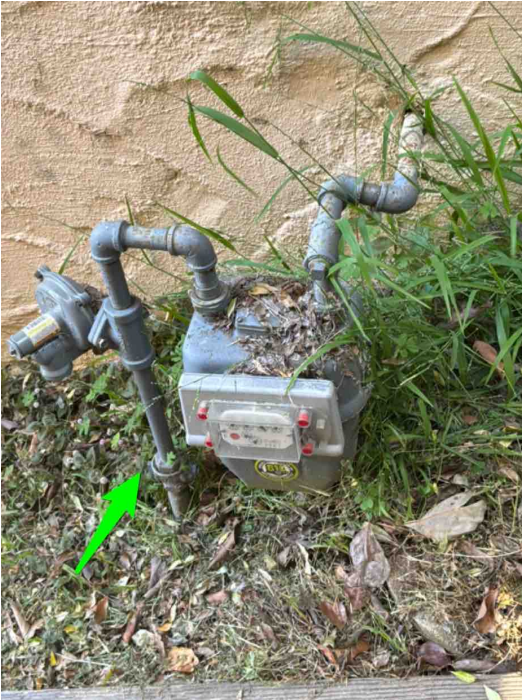
Main gas shut off valve
