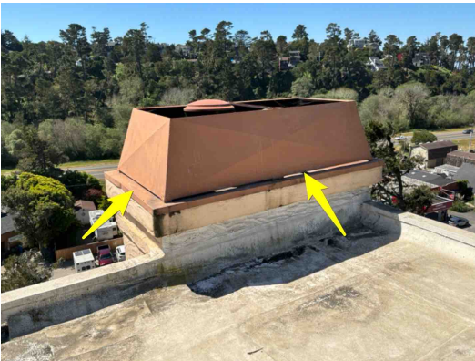
Must have a minimum of a 4 inch opening around the decorative surround
