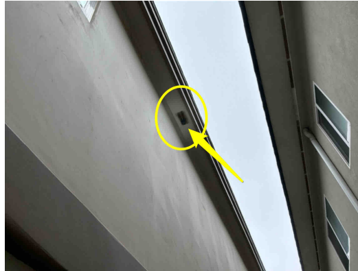
A visible hole found in the west side vent screen
