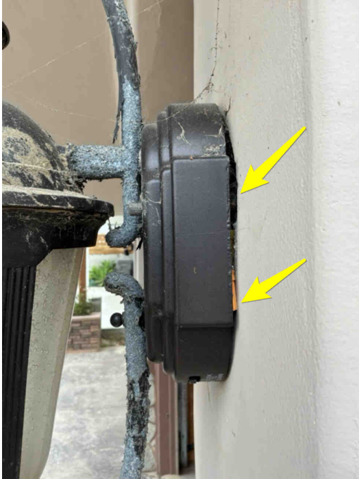
Visible electrical wiring
