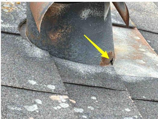
A visible hole in the roof flashing
