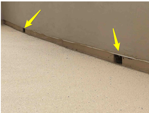
Scupper is undersized
