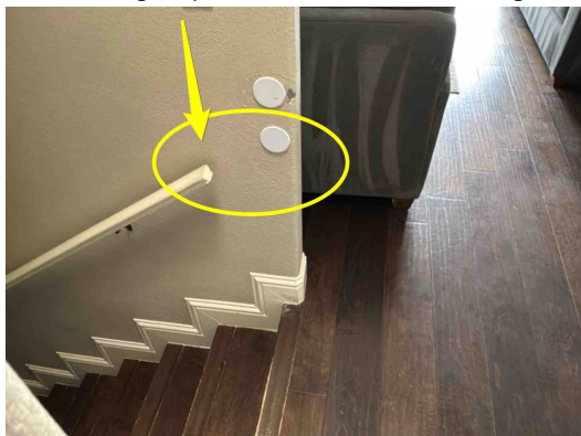
Handrail stop shorts at the top of the stairway
