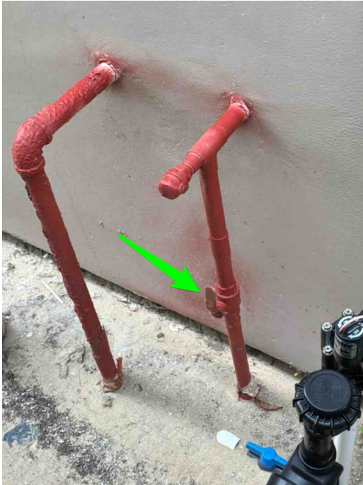
Main water shut off valve
