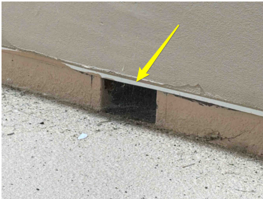
Scupper is undersized
