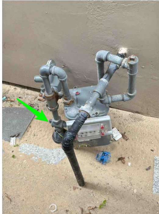
Main gas shut off valve
