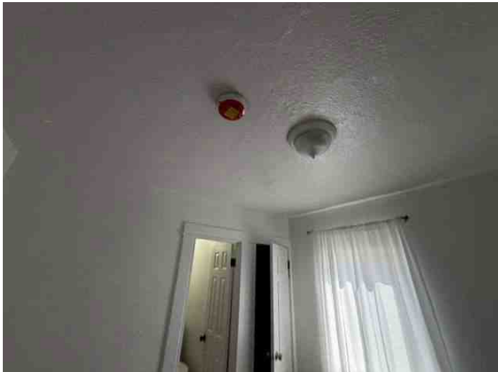
UNIT D-Smoke/Carbon Monoxide Alarm
